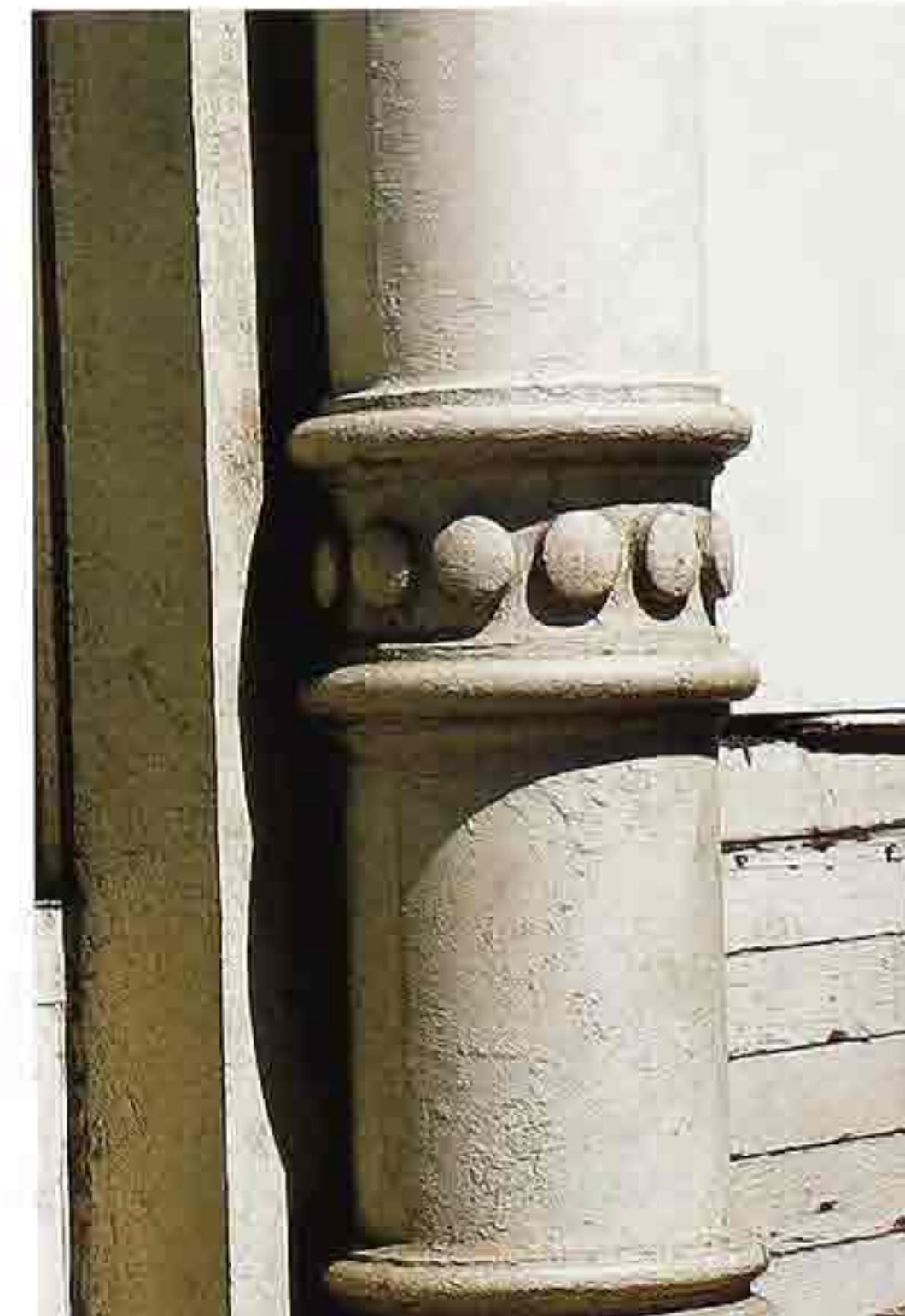
CP-63 Cast-iron column with Doric/Tuscan base and a band of round ornaments on round pedestal with Attic base
