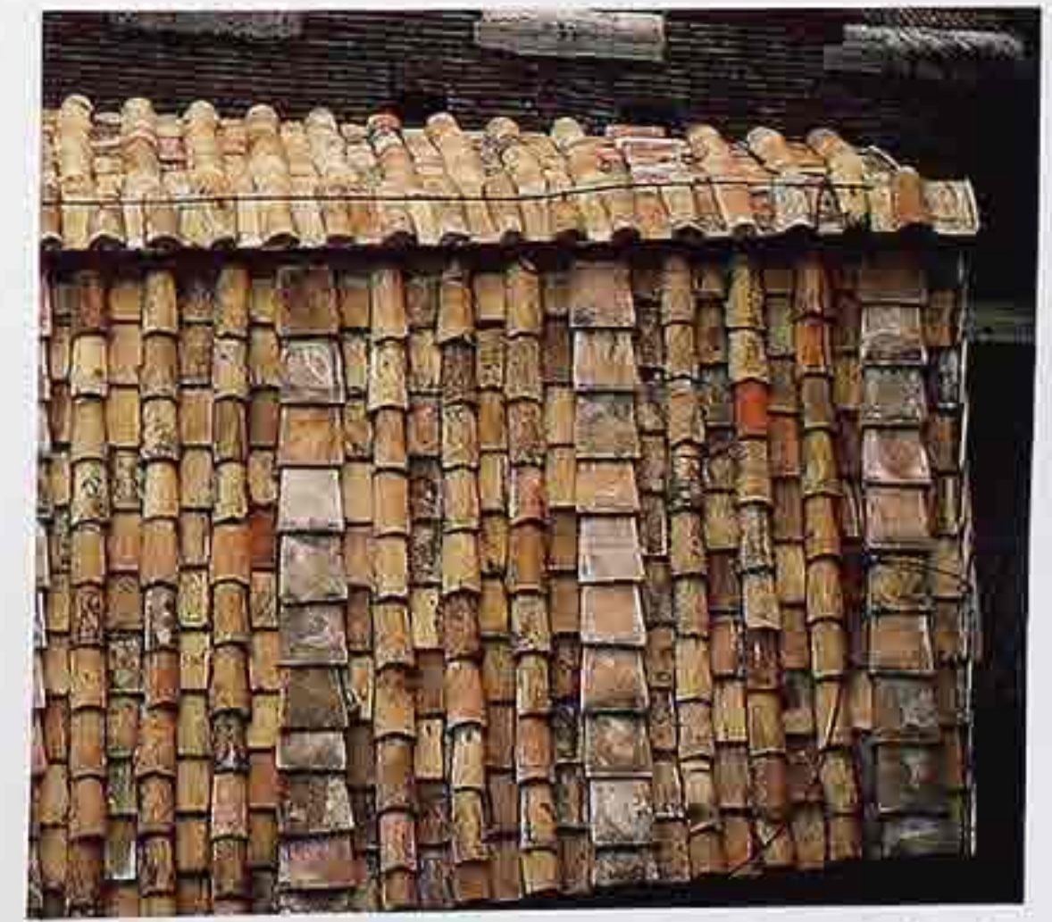
CR-43 Weathered terracotta mission and flat tiles on shed roof
