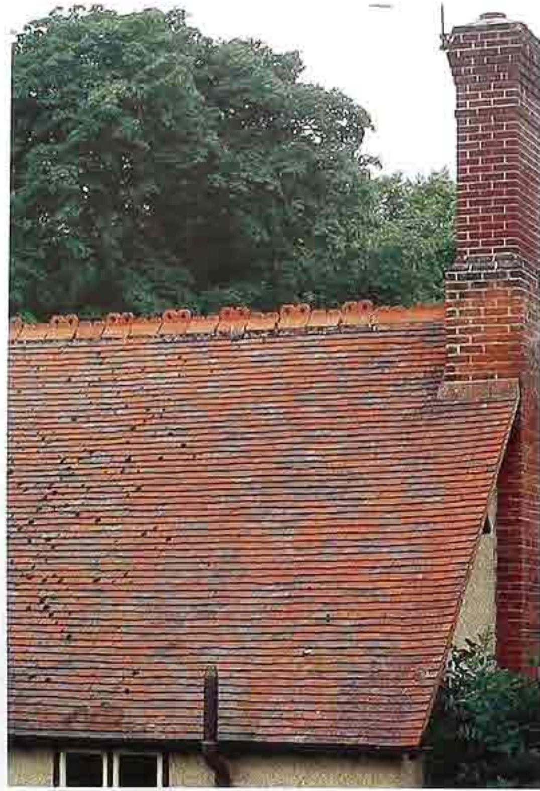
CR-54 Flat shingle terracotta tiles on gable roof with decorative ridge tiles, 19th-c. English house
