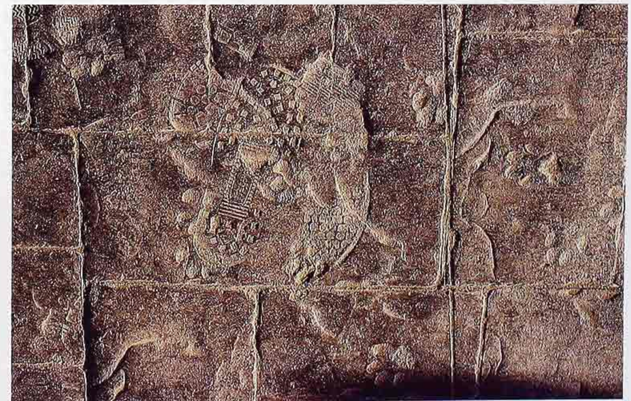
FP-80 Cast-in-place concrete stamped with pattern of stone paving and footprint in sidewalk
