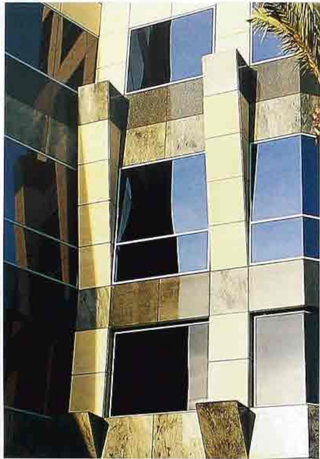
WA-145 Polished veneer in polychrome bands with plaster strips, modern commercial building
