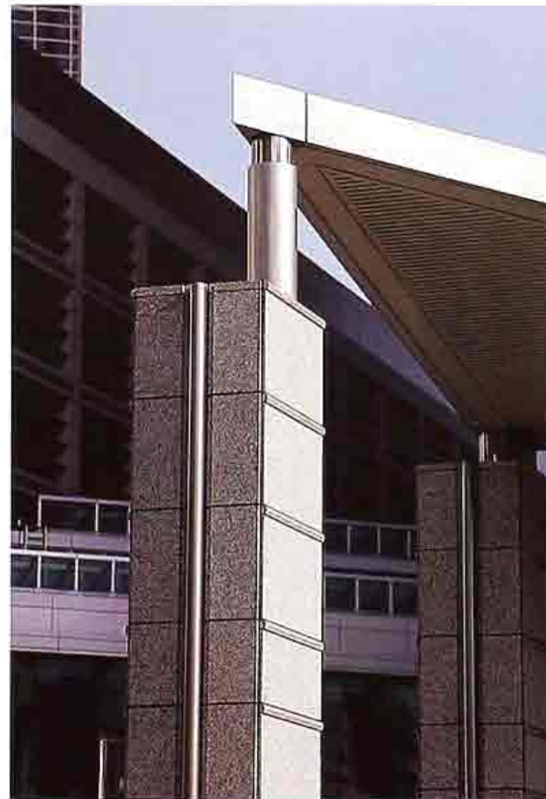
CP-131 Pier with metal post and stone cladding supporting entry canopy, modern commercial building
