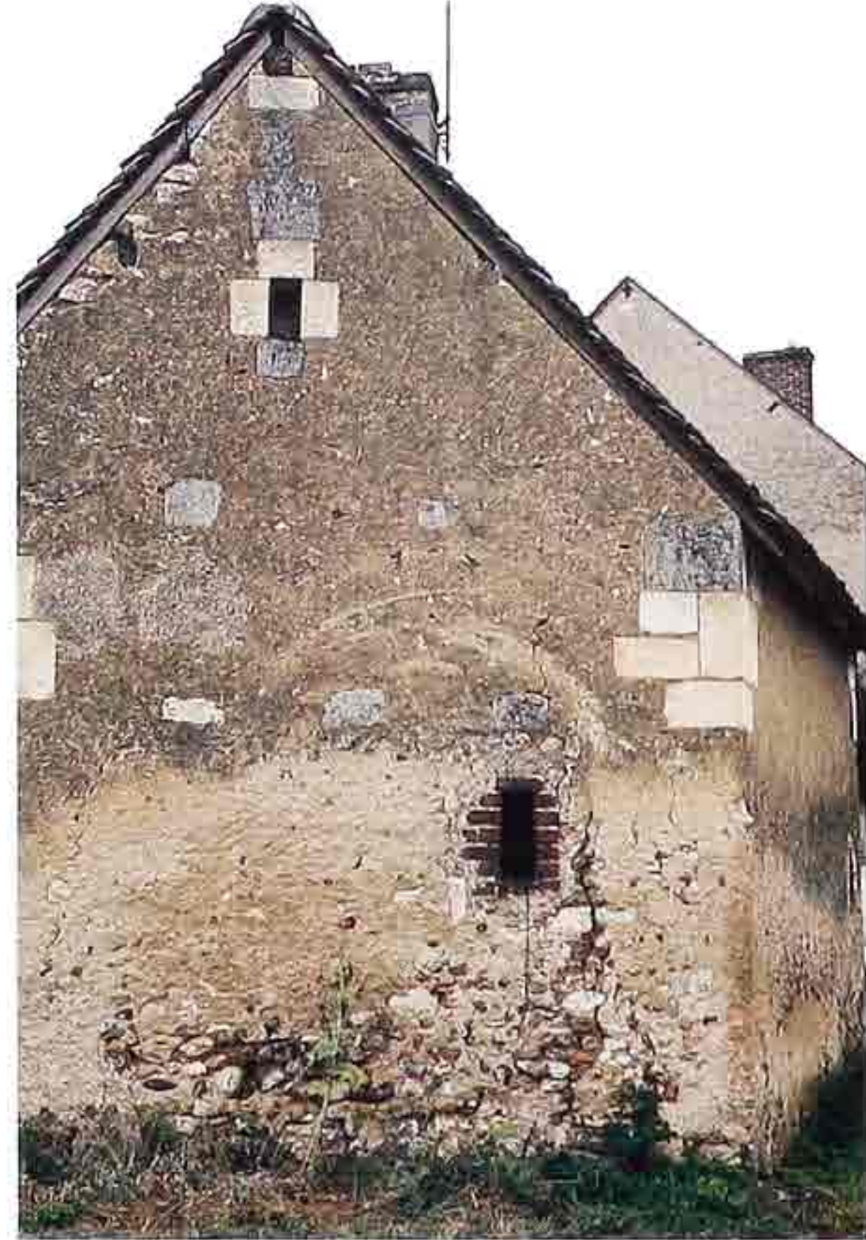
WA-249 Large-aggregate stucco with cobbles and quins on weathered gable-end wall, farm building
