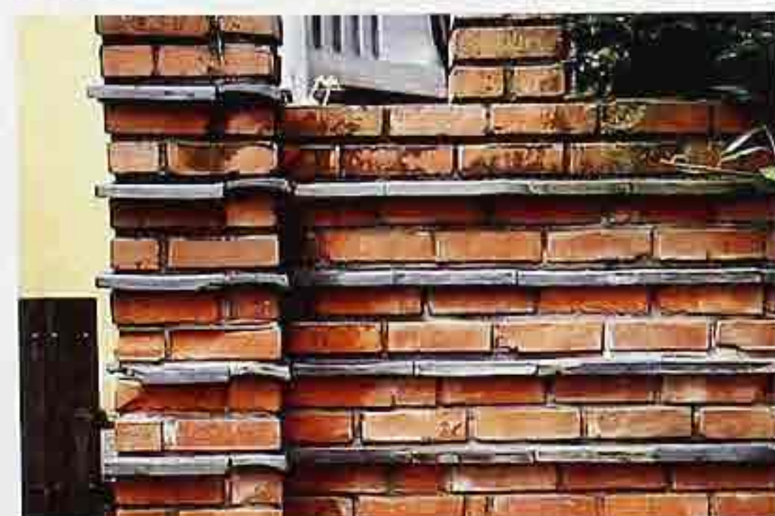
WA-268 Single courses of slate alternating with double courses of brick in running bond, garden wall
