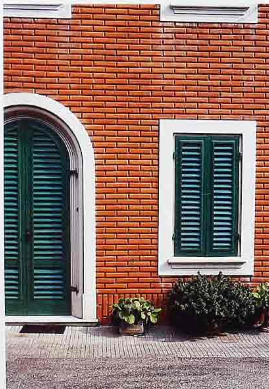
WA-177 Modern variation of Roman brick in running bond with tinted mortar and soldier base course; louvered shutters on door and window
