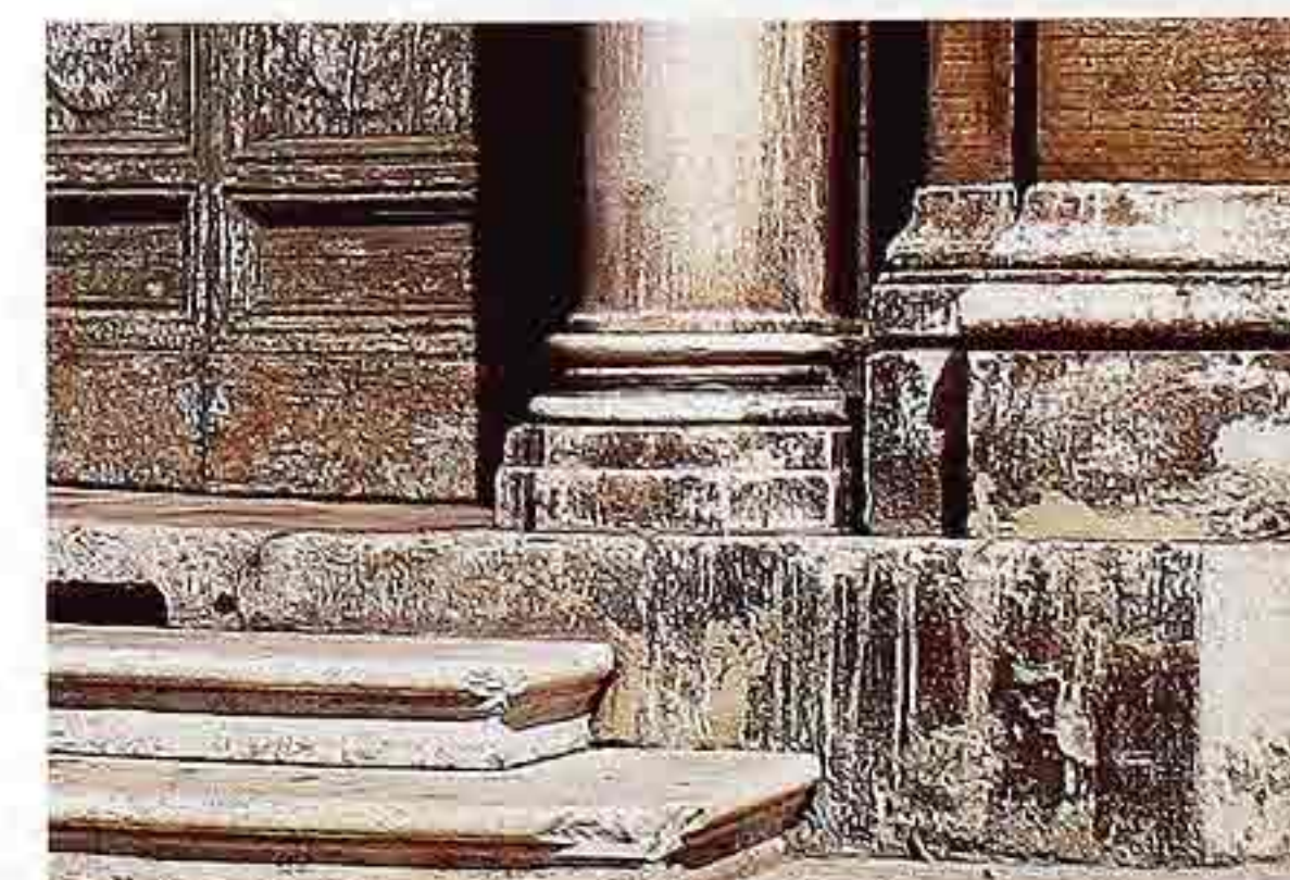
CP-39 Weathered marble column with Attic base on stepped octagonal plinth; right: brick pilaster on square marble base
