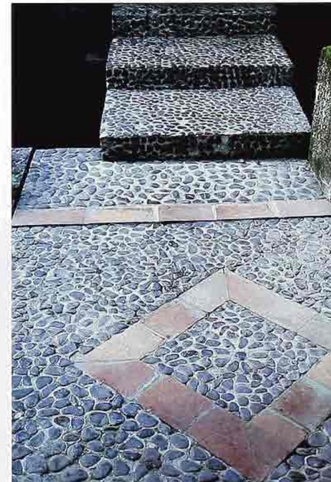
FP-70 Exposed aggregate with terracotta tile insets on steps and floor in entryway. Aggregate applied, not revealed by washing
