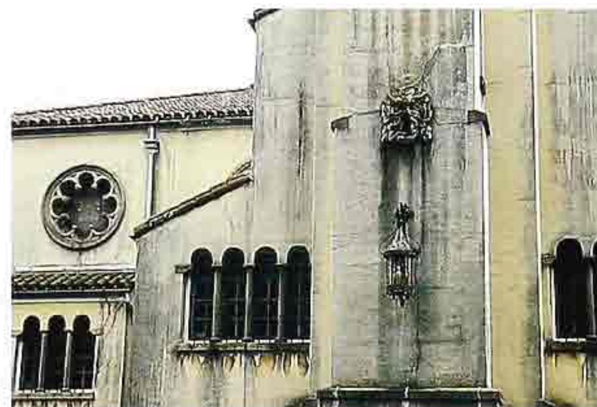
WA-257 Weathered colored stucco, Italianate building
