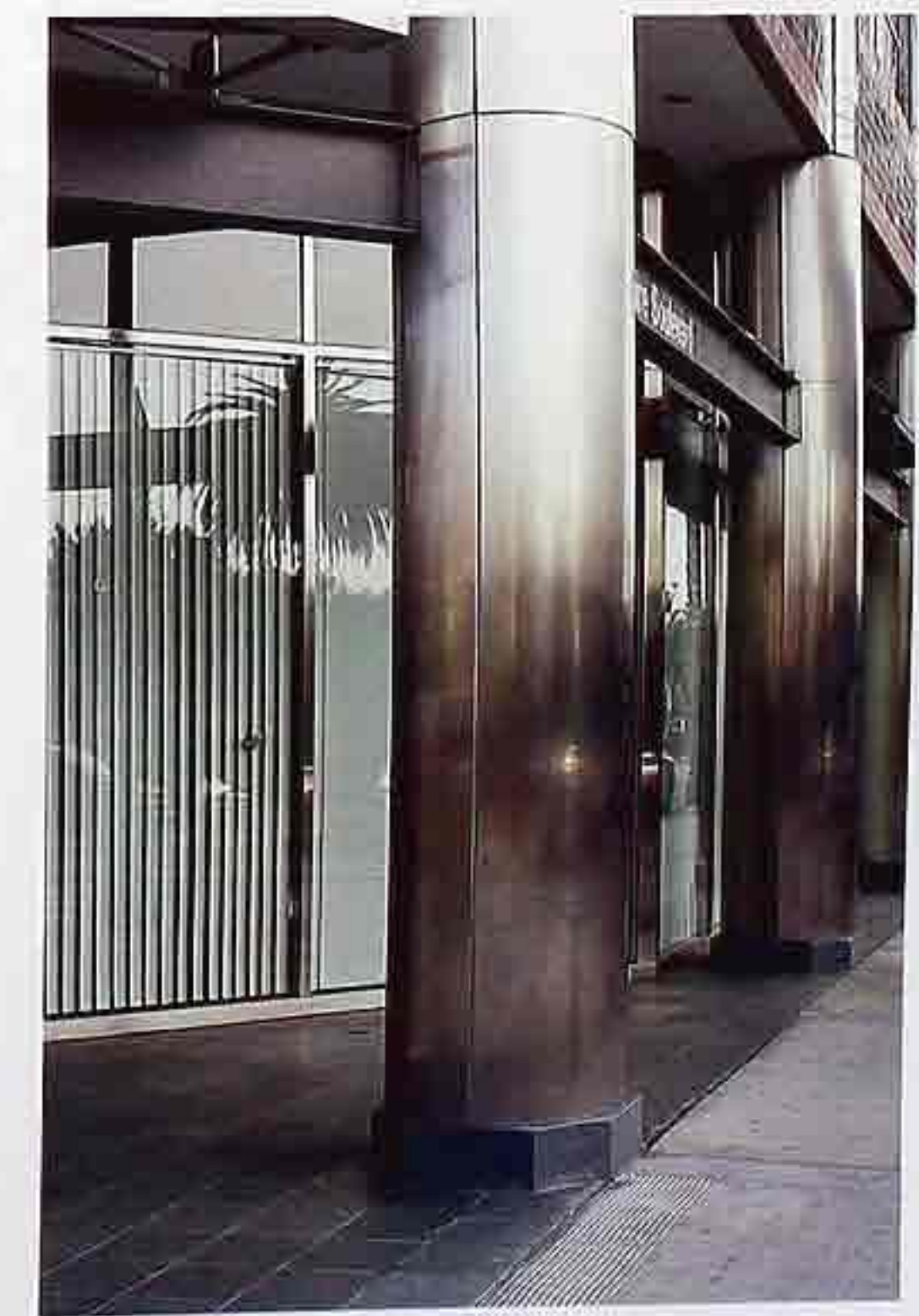
CP-129 Steel column with stainless-steel cladding supporting entry canopy, modern commercial building
