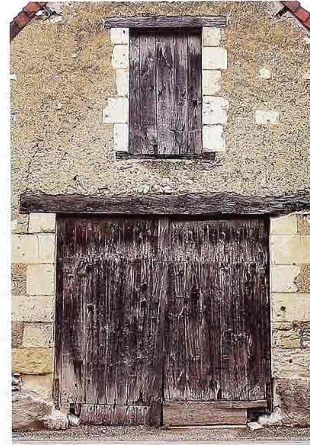
DW-26 Weathered plank doors under rough-hewn timber lintel; rustic stone and stucco gable wall of barn and hayloft
