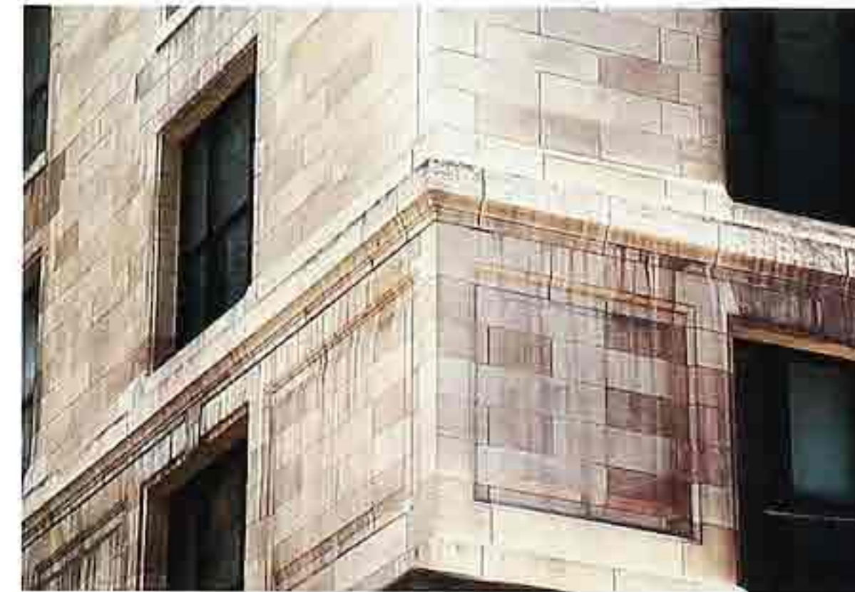
WA-103 Limestone in coursed ashlar with molding course and framed, recessed panels, water-damage weathering
