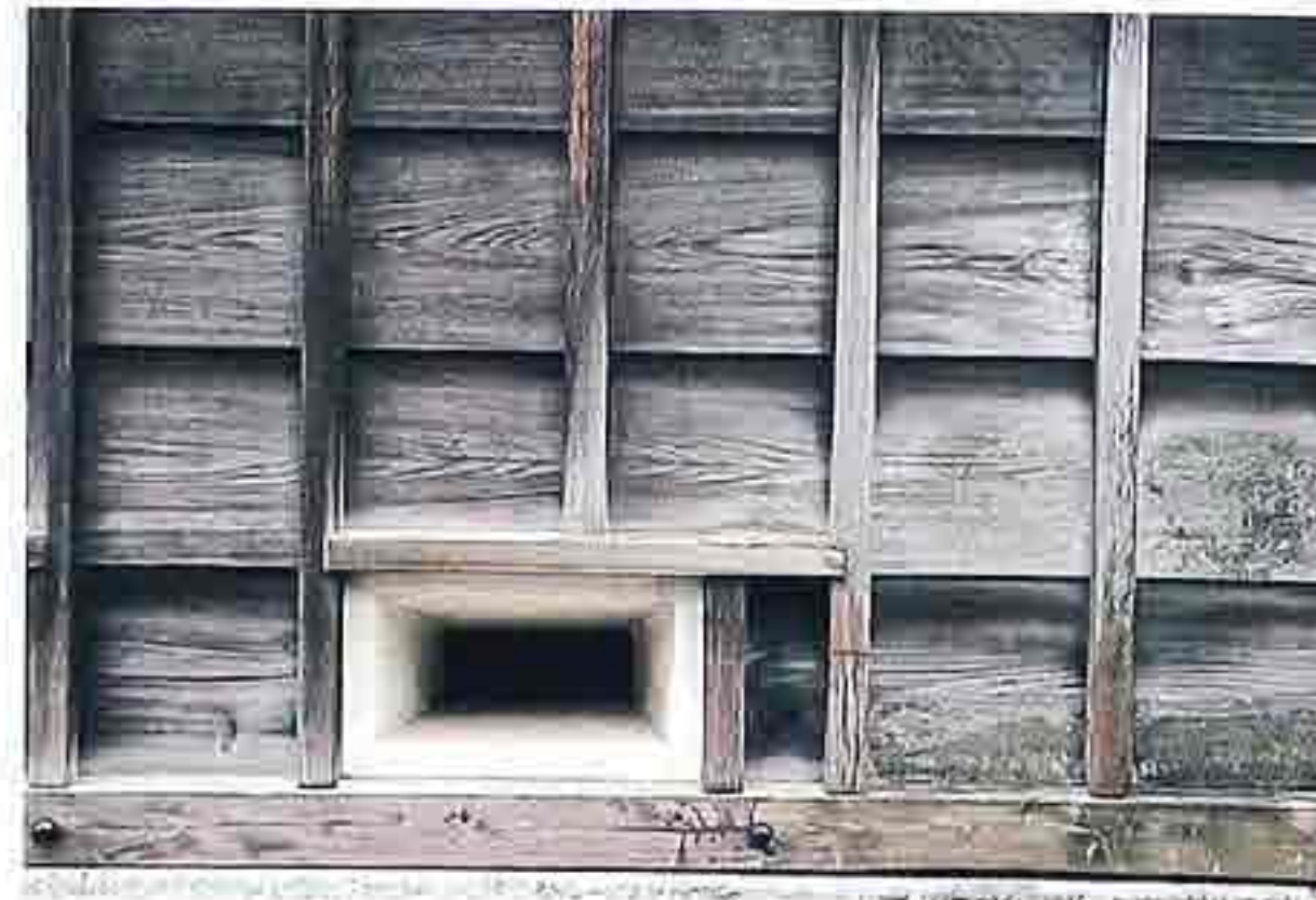
WA-10 Timber-frame construction with infill of plain-sawn cedar planks with ceramic ventilation opening
