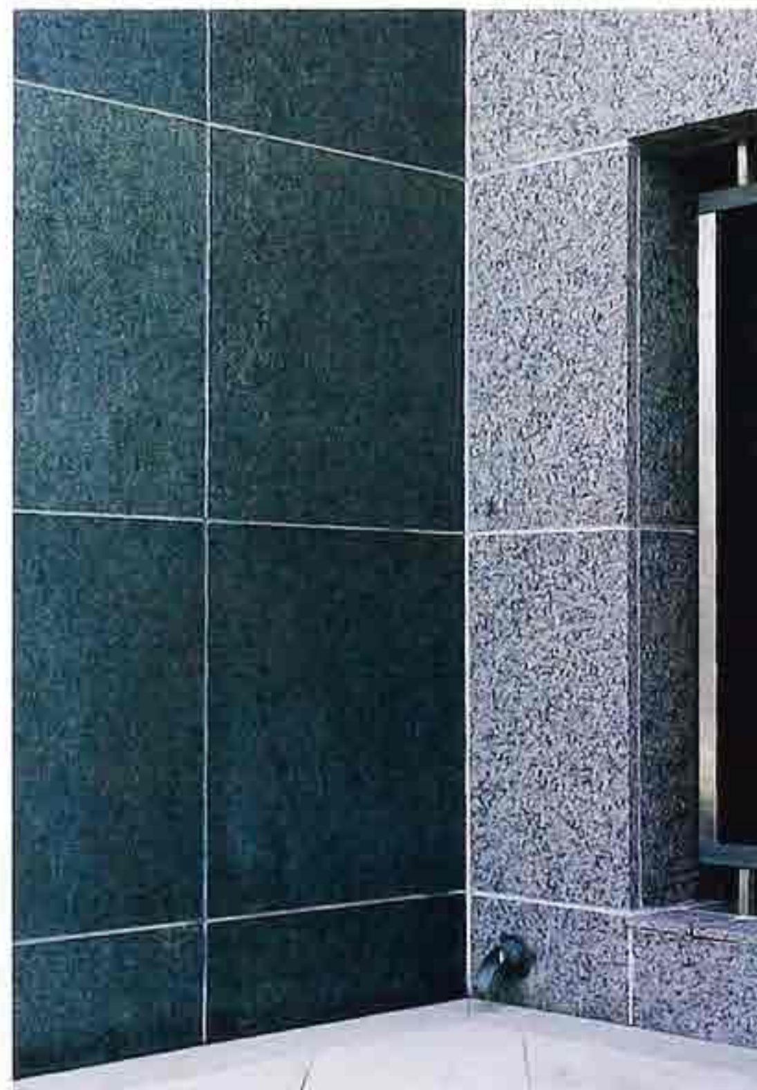
WA-134 Inside corner of honed-granite veneer in stack bond with grouted joints and window reveal, modern commercial building
