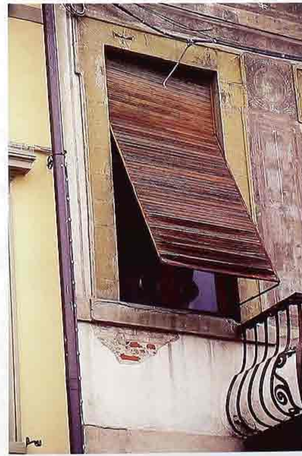
WI-181 Weathered metal awning
