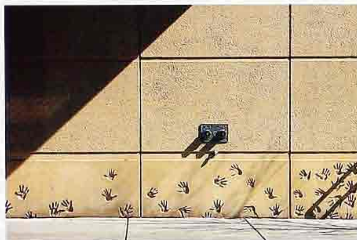
WA-240 Cast concrete walls imitating stack bond, base course decorated with imprints of children's hands, urban public space
