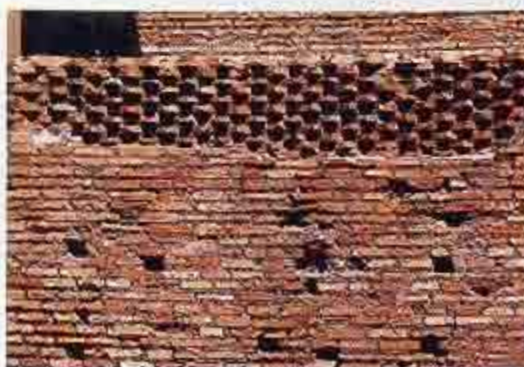
WA-163 Ancient Roman brick wall with structural dog-tooth course exposed by weathering of brick facing layer
