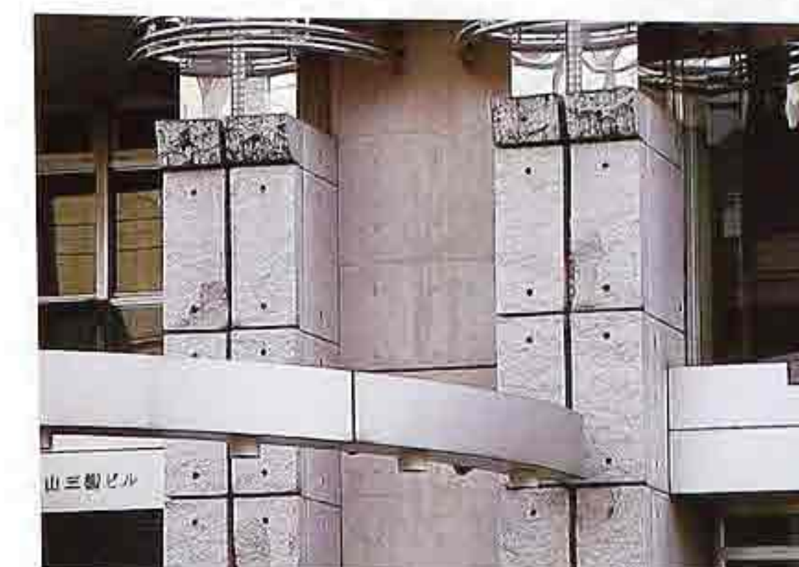
CP-117 Piers built up from split-faced stone or concrete; modern commercial building
