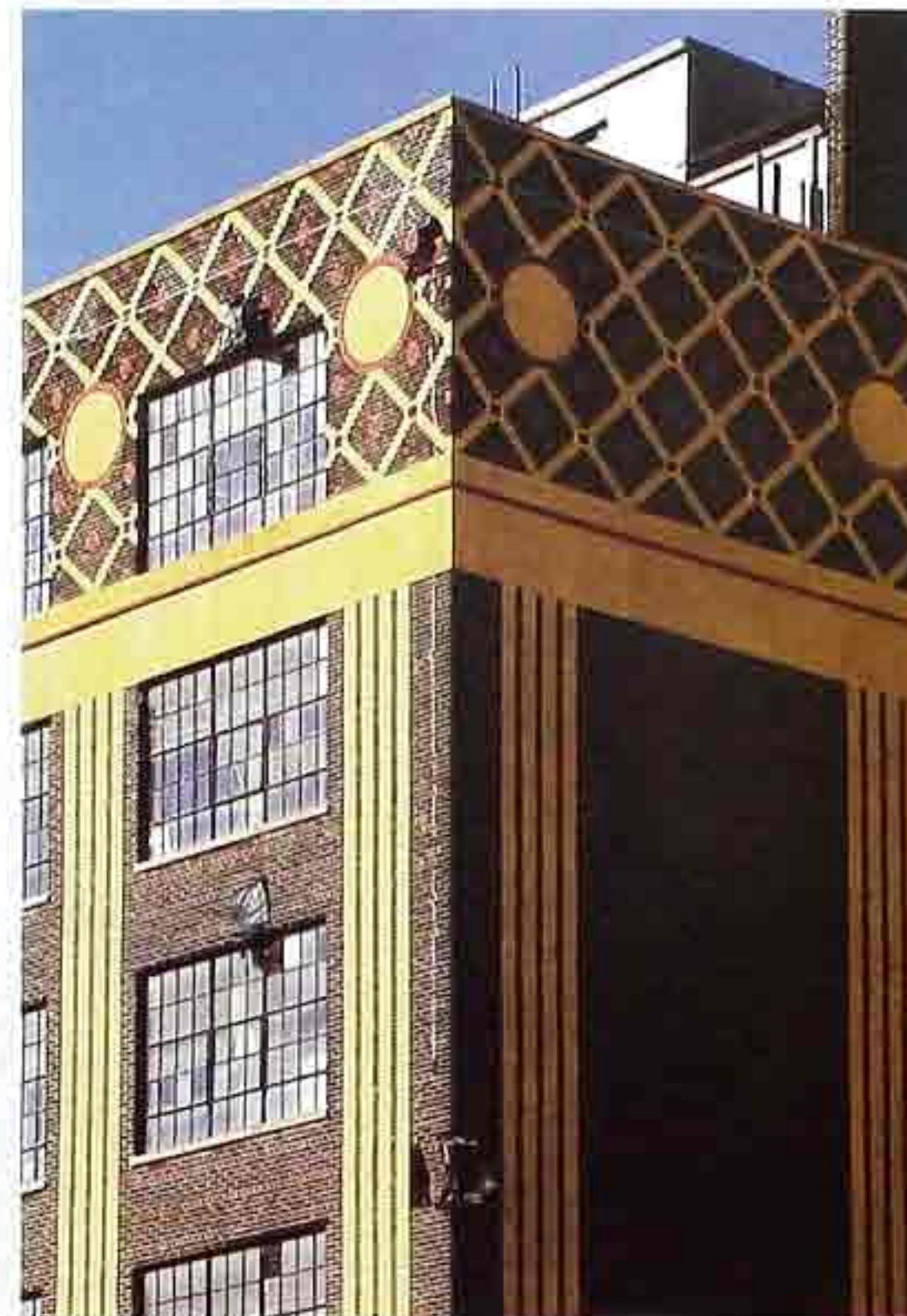
WA-198 Corner detail of decorative brickwork: diaper-patterned brickwork in contrasting colors with roundels and vertical stripes suggesting fluted pilasters
