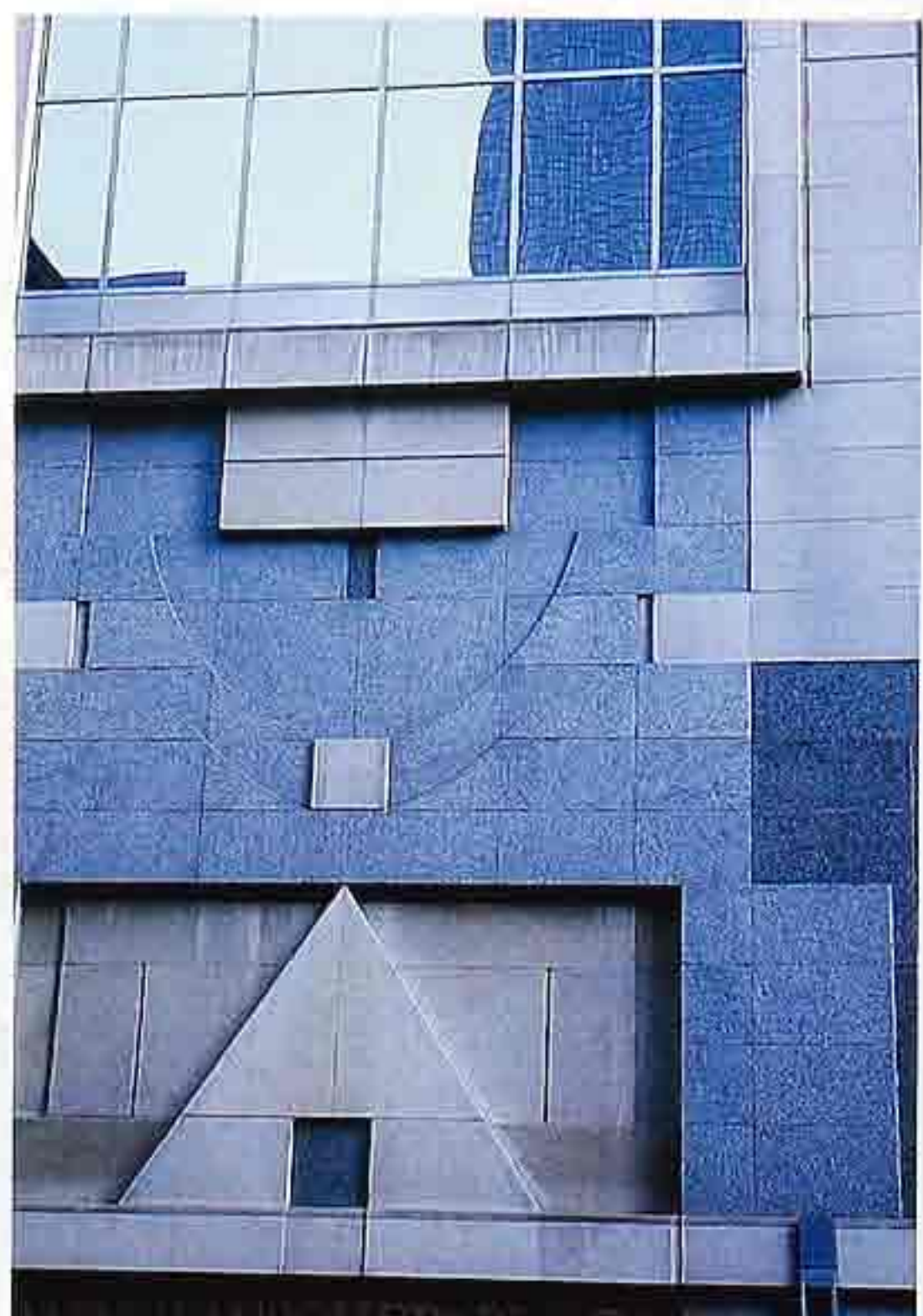
WA-148 Polychrome stone-veneer collage of polished and honed granites, modern commercial building
