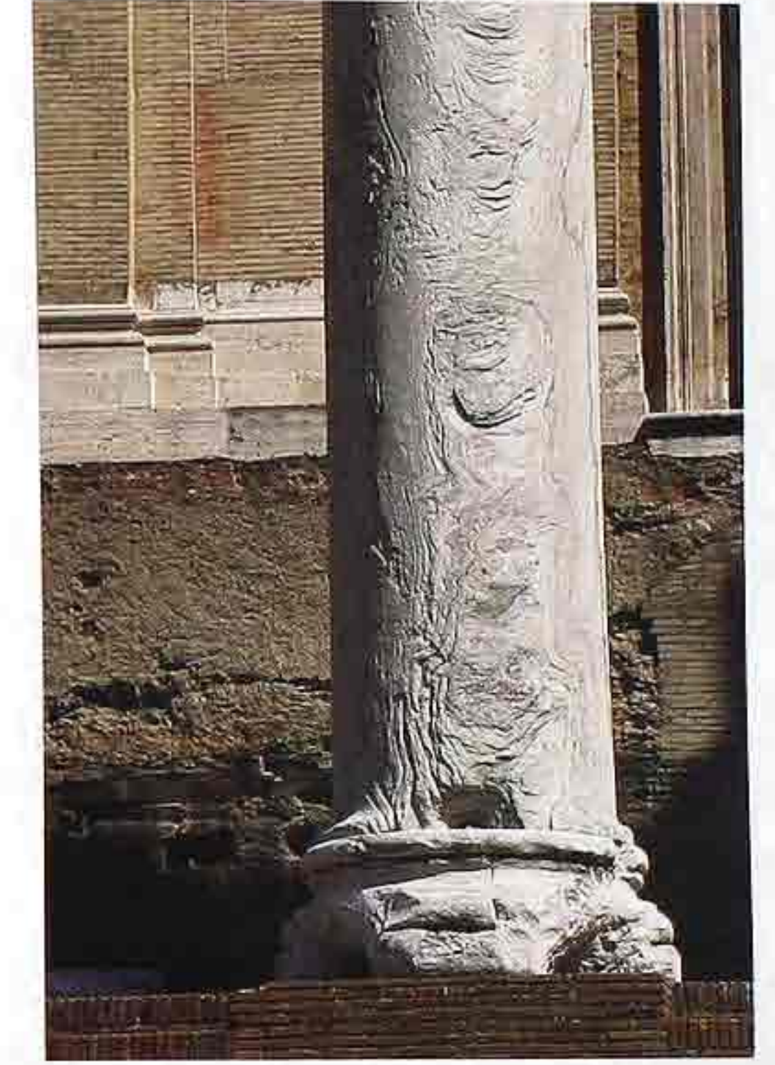
CP-62 Heavily weathered ancient Roman column with remnants of Attic base
