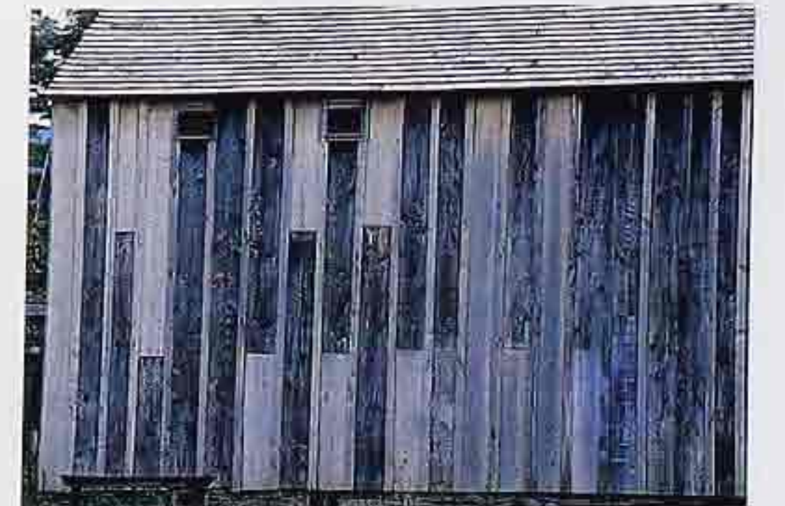
WA-27 Weathered board-and-batten siding on outbuilding
