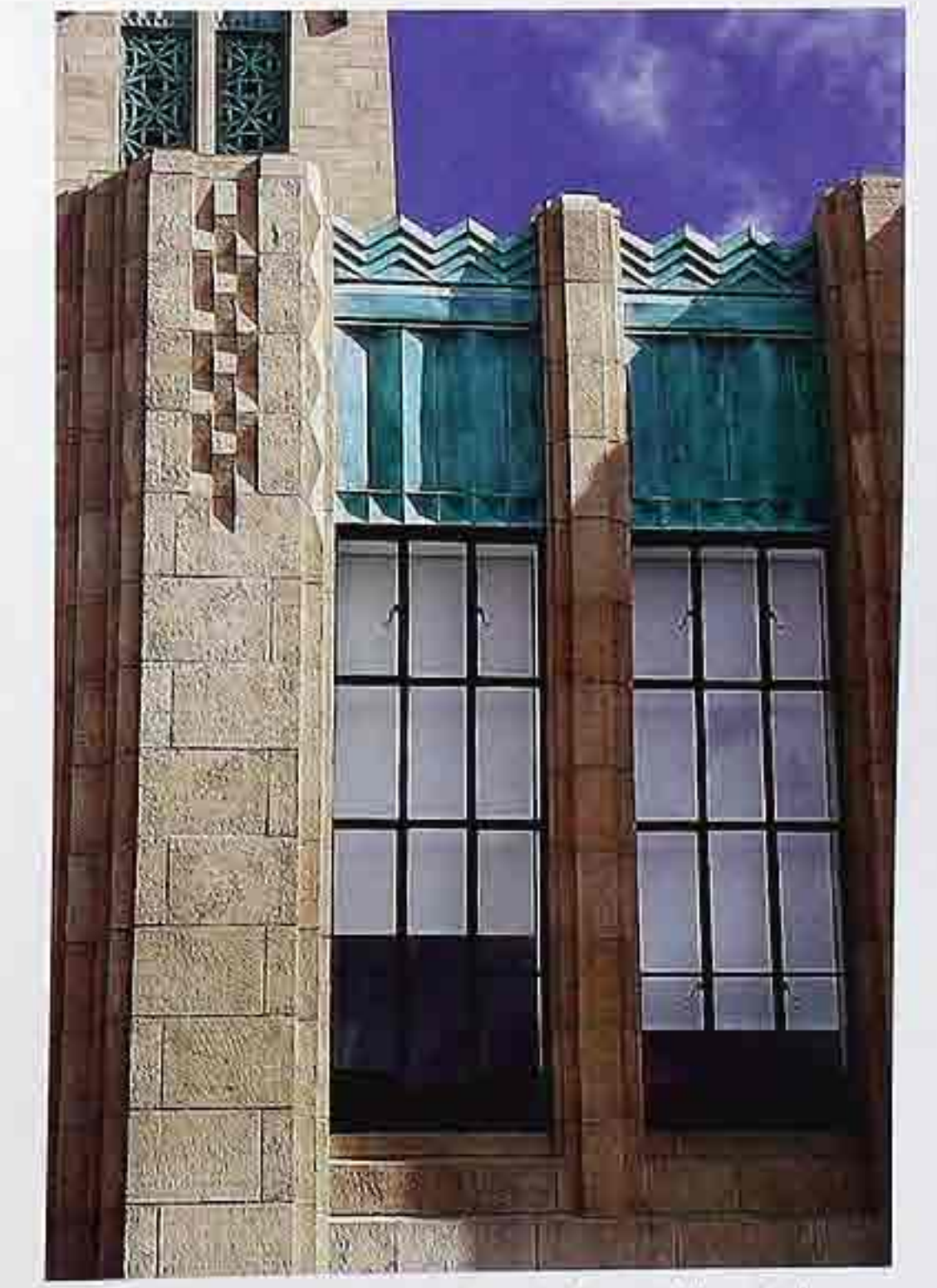
WI-149 Copper panels capping windows with metal sashes in recessed stone casings, 20th-c. commercial building
