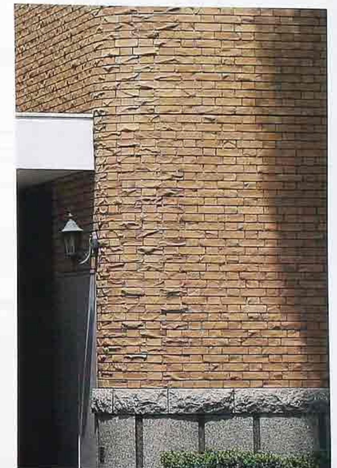
WA-150 Rusticated brick in Flemish bond, shelf angle, with curved corner above granite rock-face belt course and honed base
