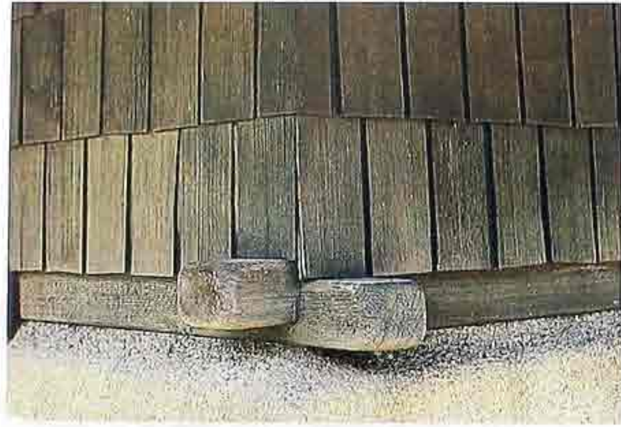
WA-9 Notched corner joint of square timber frame with painted cedar shakes on concrete foundation
