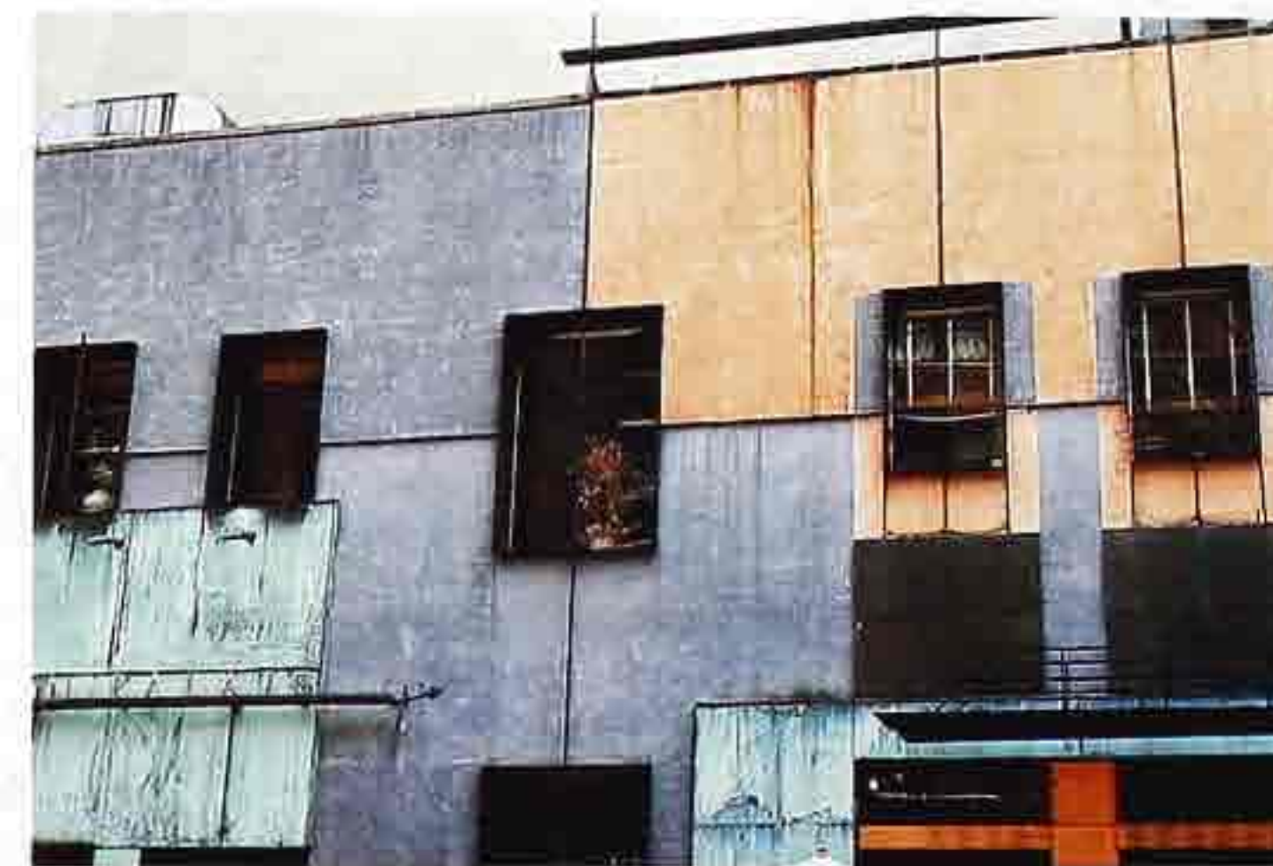
FA-24 Painted and patinated metal panels with lapped seams, modern commercial building
