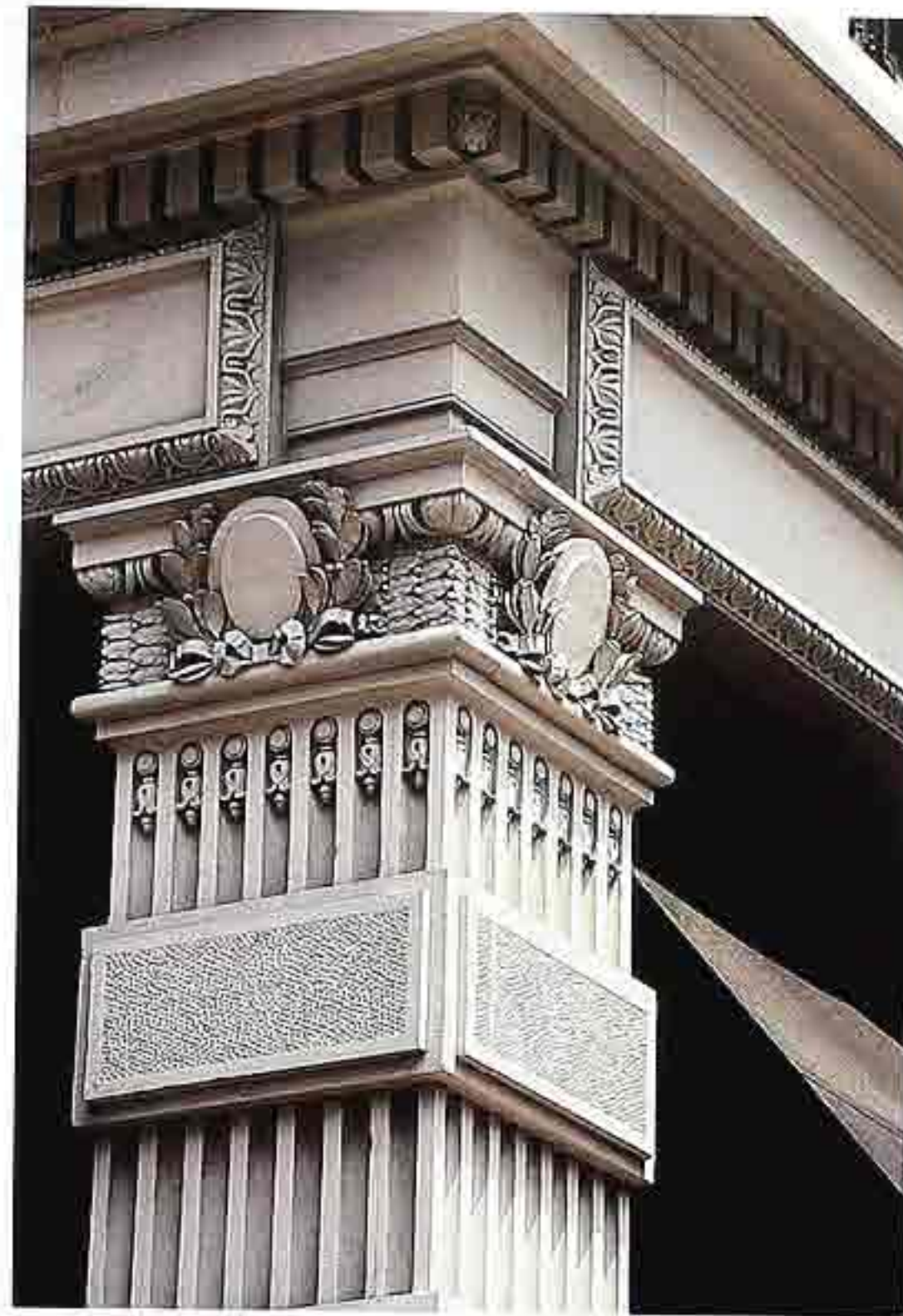
OM-106 Three-banded architrave, plain shallow soffit, raised panels surrounded by leaf-and-dart molding over architrave
