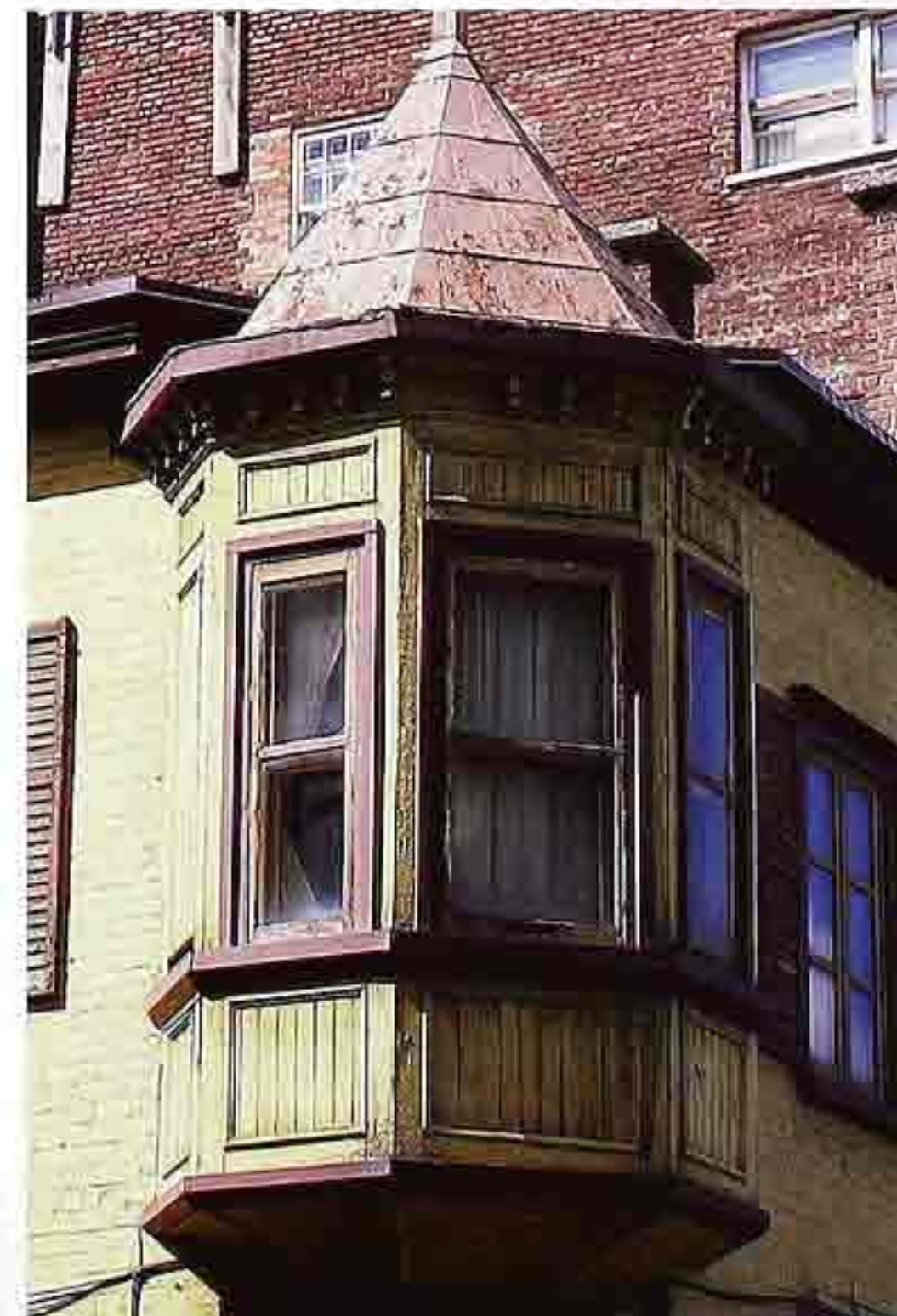
WI-78 Wood corner oriel: one-over-one, double-hung, wood sashes and casings, conical flat-seamed copper roof, 19th-c. American mixed-use building
