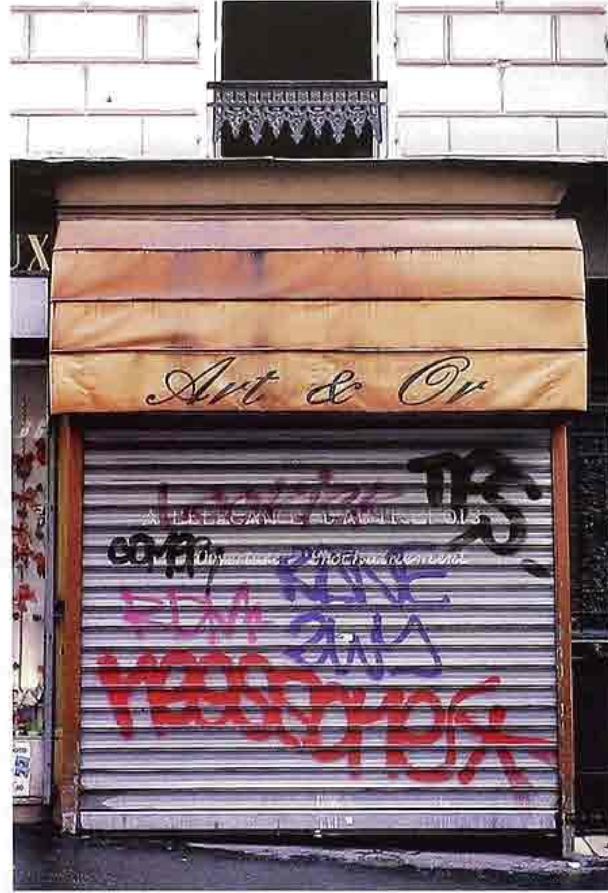
DW-53 Rolling galvanized-metal security door with graffiti
