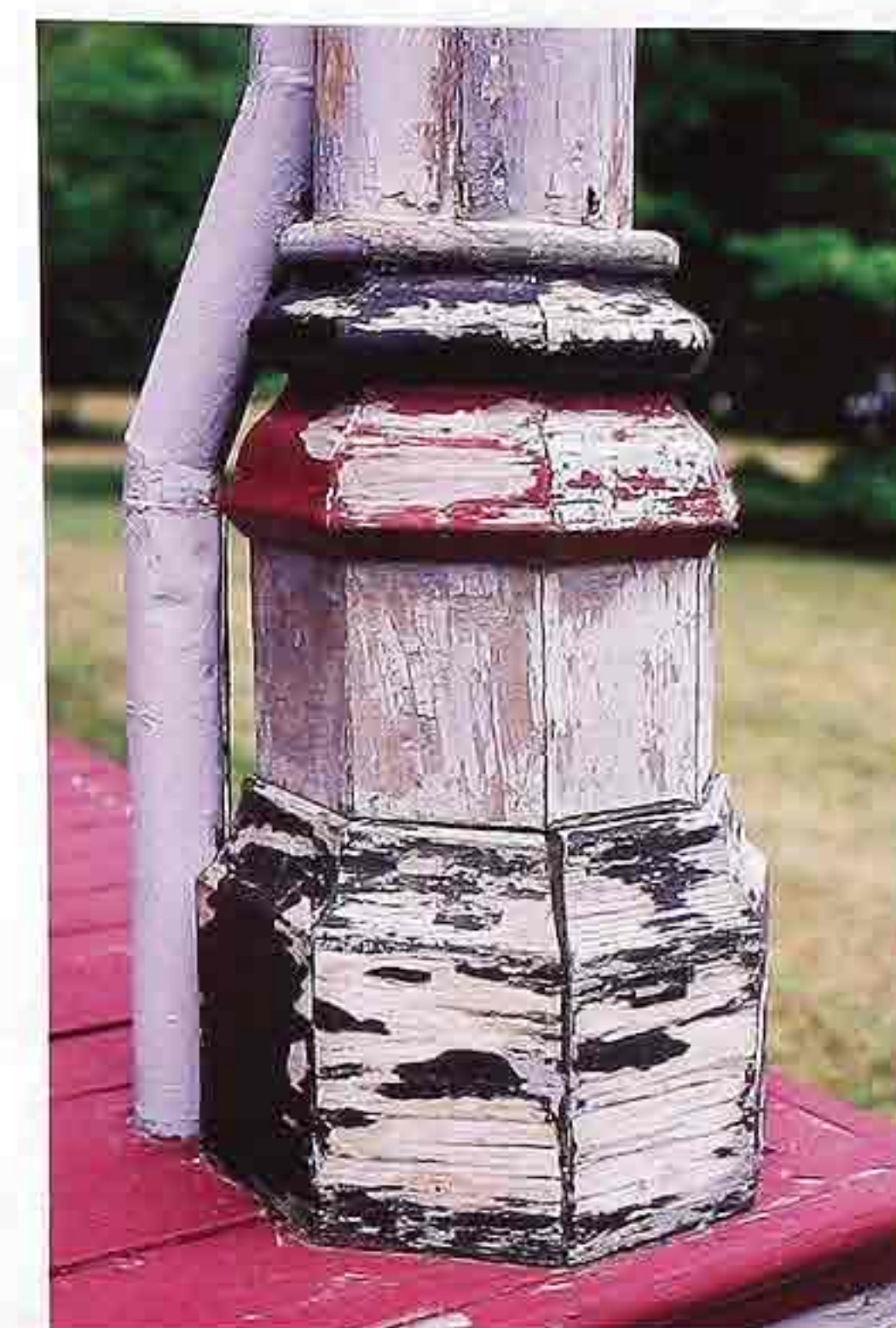
CP-55 Heavily weathered painted octagonal wood base in Carpenter Gothic style
