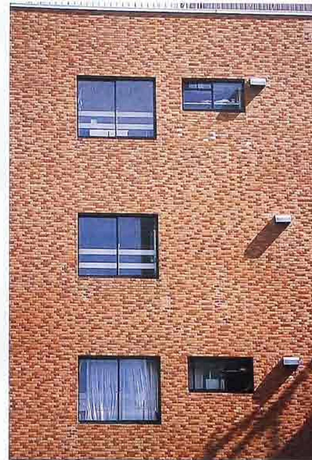
WA-179 Mottled effect in polychrome toned brick, modern residential building
