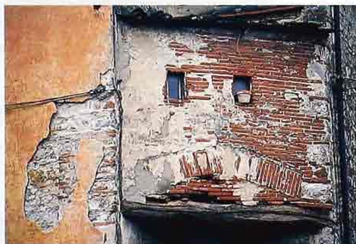
WA-256 Weathered colored stucco revealing timber lintel, scratch coat and structural stone, and Roman brick
