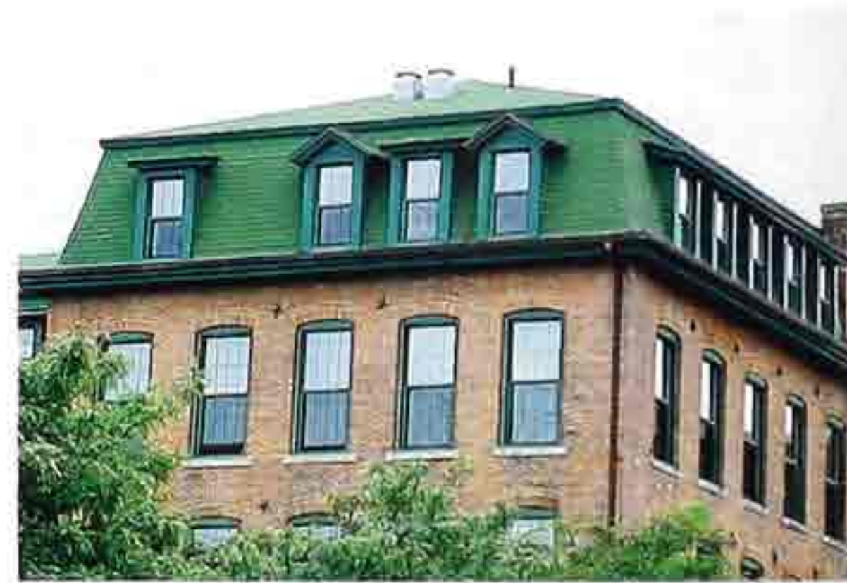
CR-118 Mansard with row of shed dormers (right) and alternating gable and shed dormers (left)
