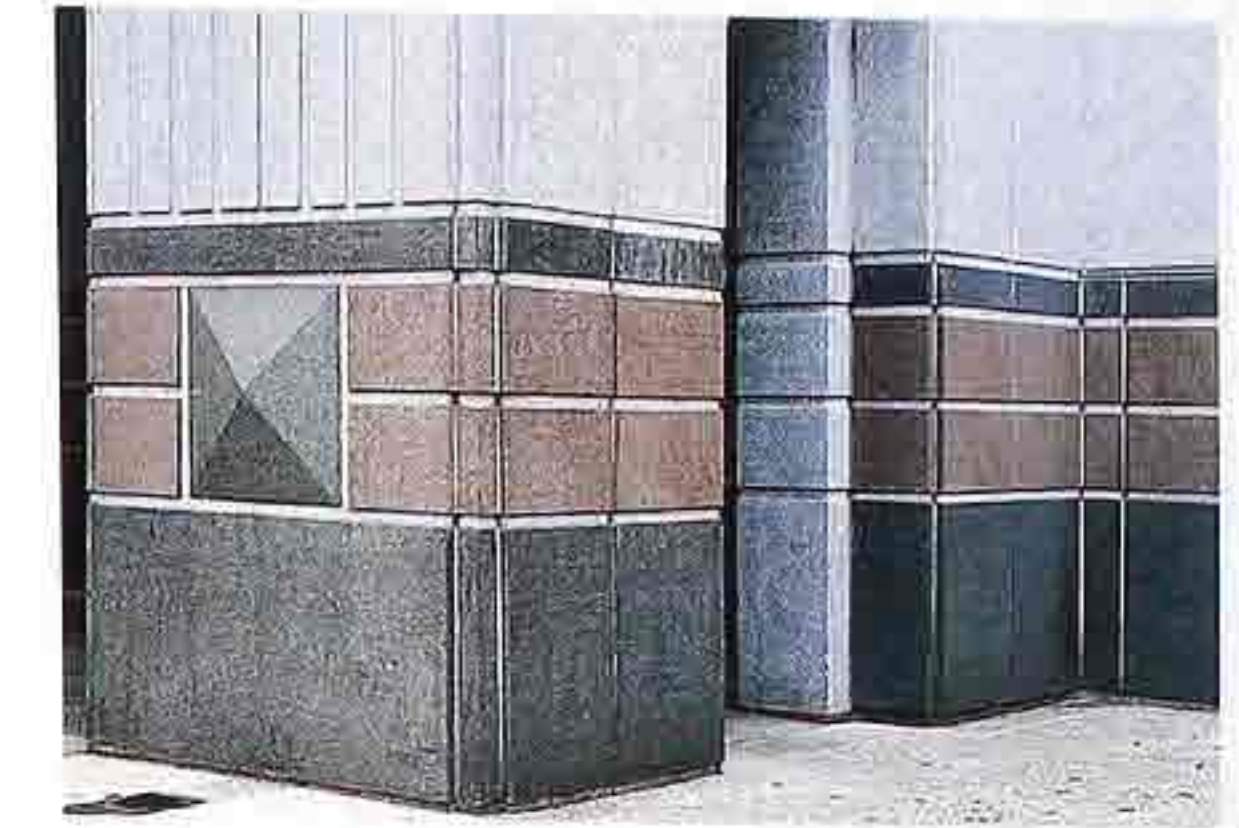
WA-127 Corner detail of polychrome banded granite veneer with gem-cut decorative block
