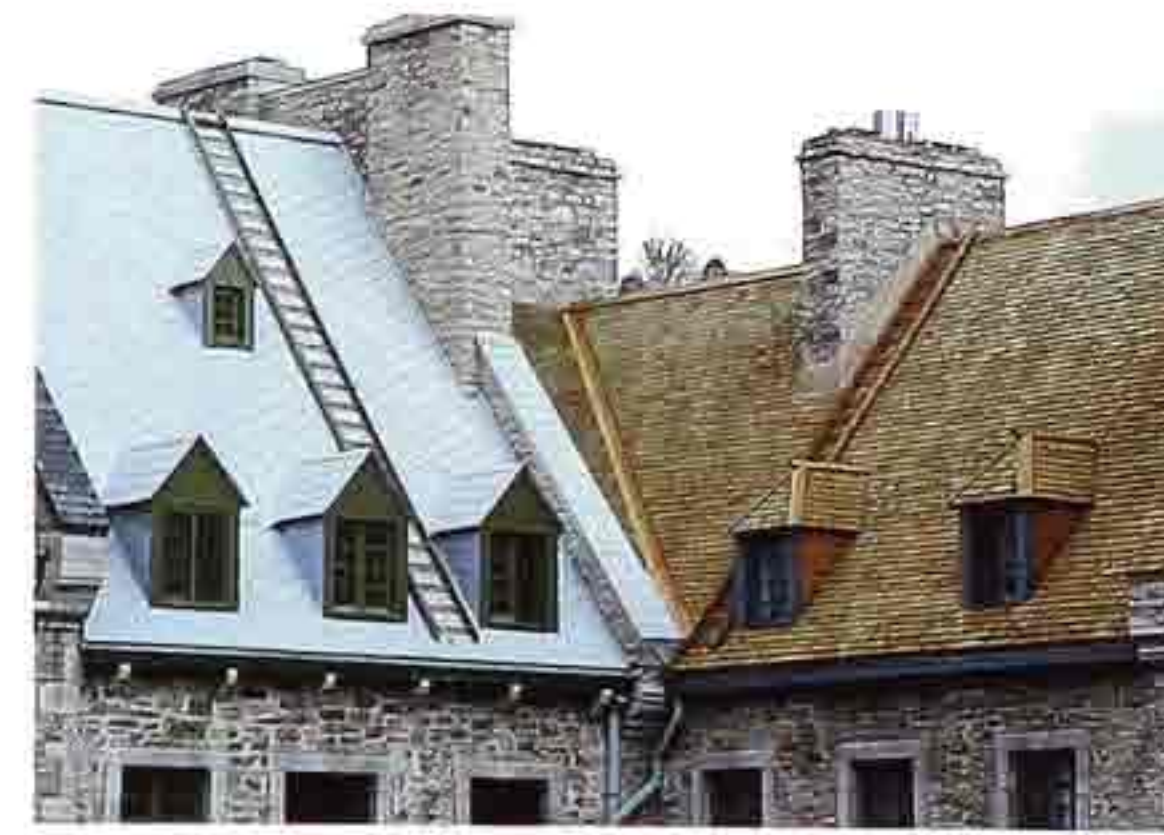
CR-120 Left: gable with roof dormers, metal with flat seam; right: gable with hipped-roof dormers, wood shingle; flashing in roof valley
