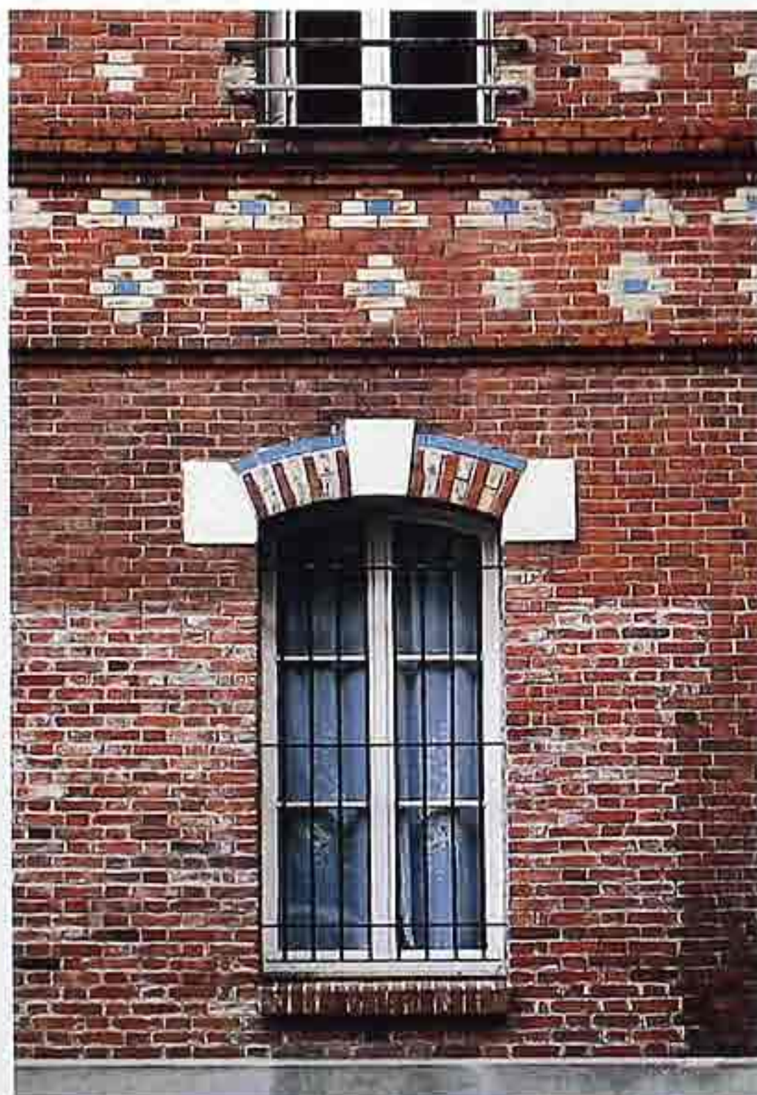
WA-199 Gauged-brick segmental window arch with stone keystone under decorative brickwork of multi-colored English cross bond
