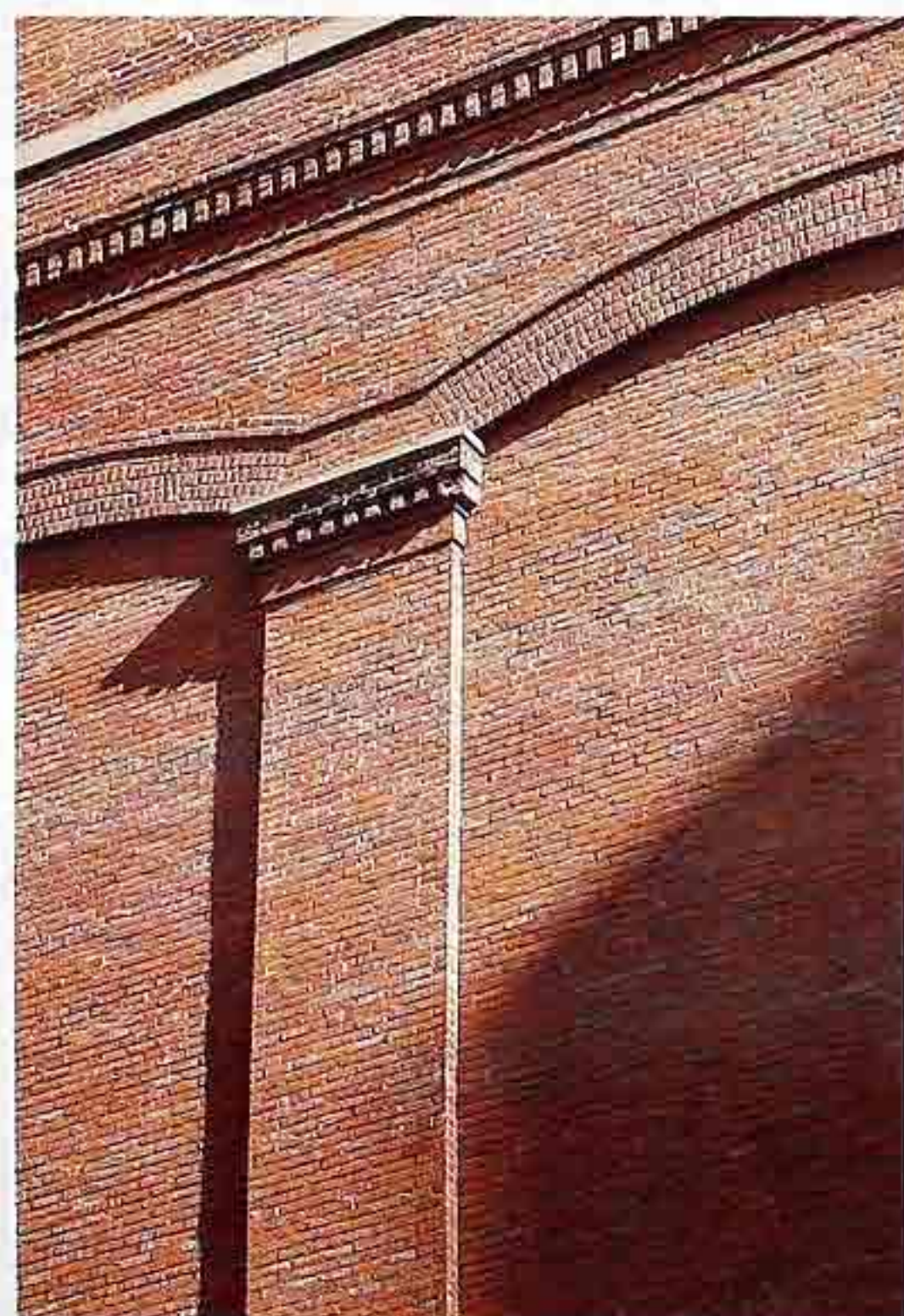
CP-90 Brick pilaster with dentil motif at the capital and blind cambered or very shallow segmental arch; denticulated molding above arch
