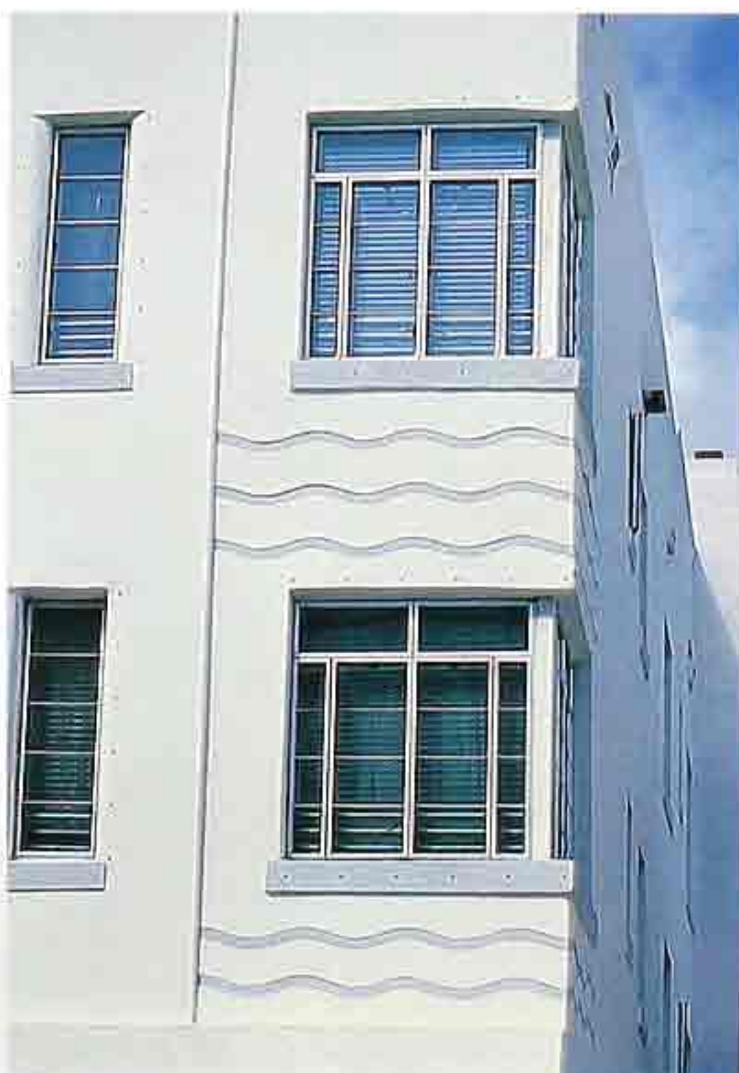
WI-89 Corner windows: double casement with side lights and split transom lights, Art Deco apartment house
