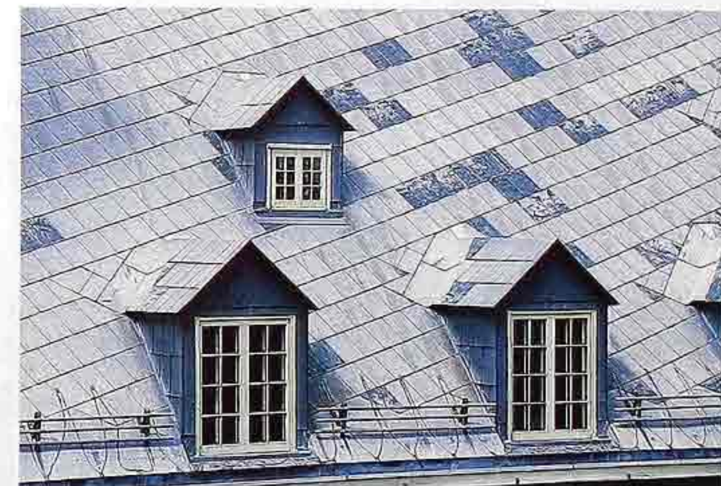
CR-28 Sheet-metal shingles with flat seams on roof and dormers; pipe-style snow guard on lower edge
