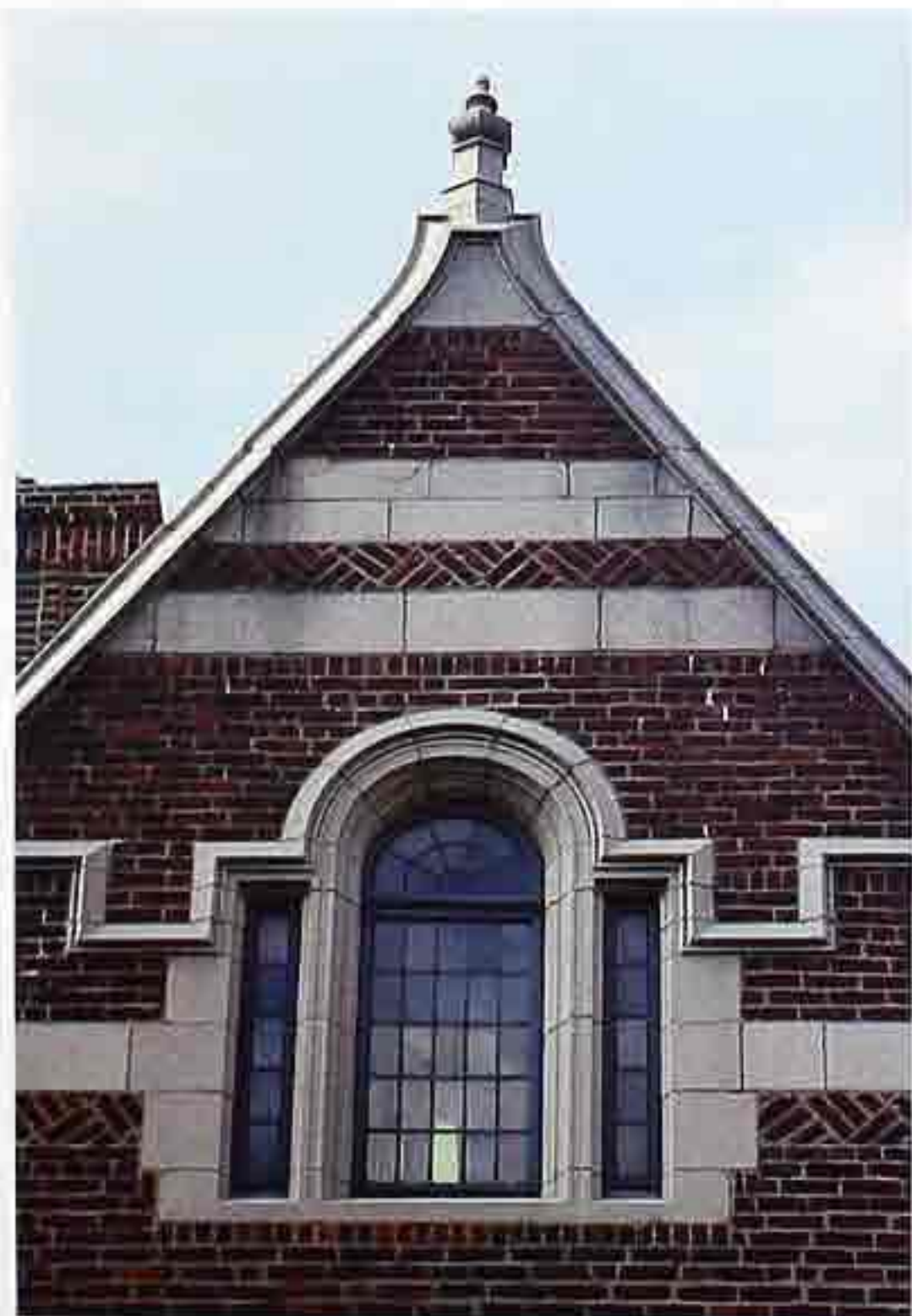
WI-96 Fanlight in Palladian window with fixed leaded lights and stone frame
