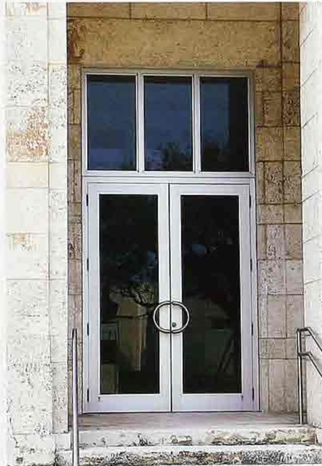
DW-58 Full glass double doors in stainless steel frame with three-light transom in recessed entryway; stone surround and steps, modern commercial building
