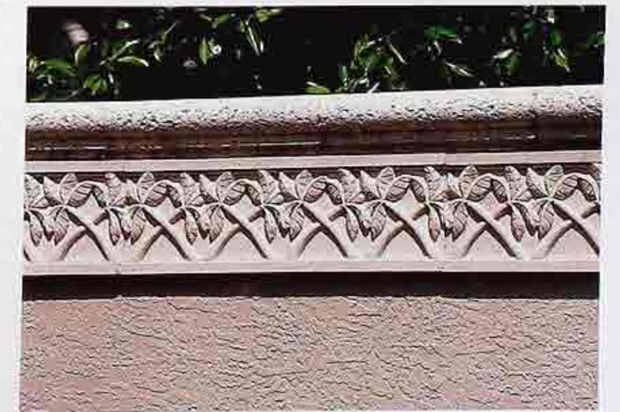
OM-38 Ornamental band with interlocking palm motif below the coping of a garden wall
