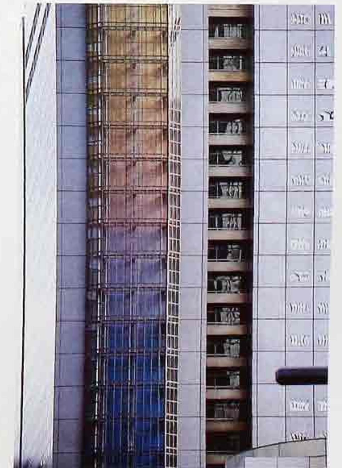
FA-39 Panelized cladding system with fully glazed curtain wall of light spectrum-producing glass or plastic enclosing elevator shaft
