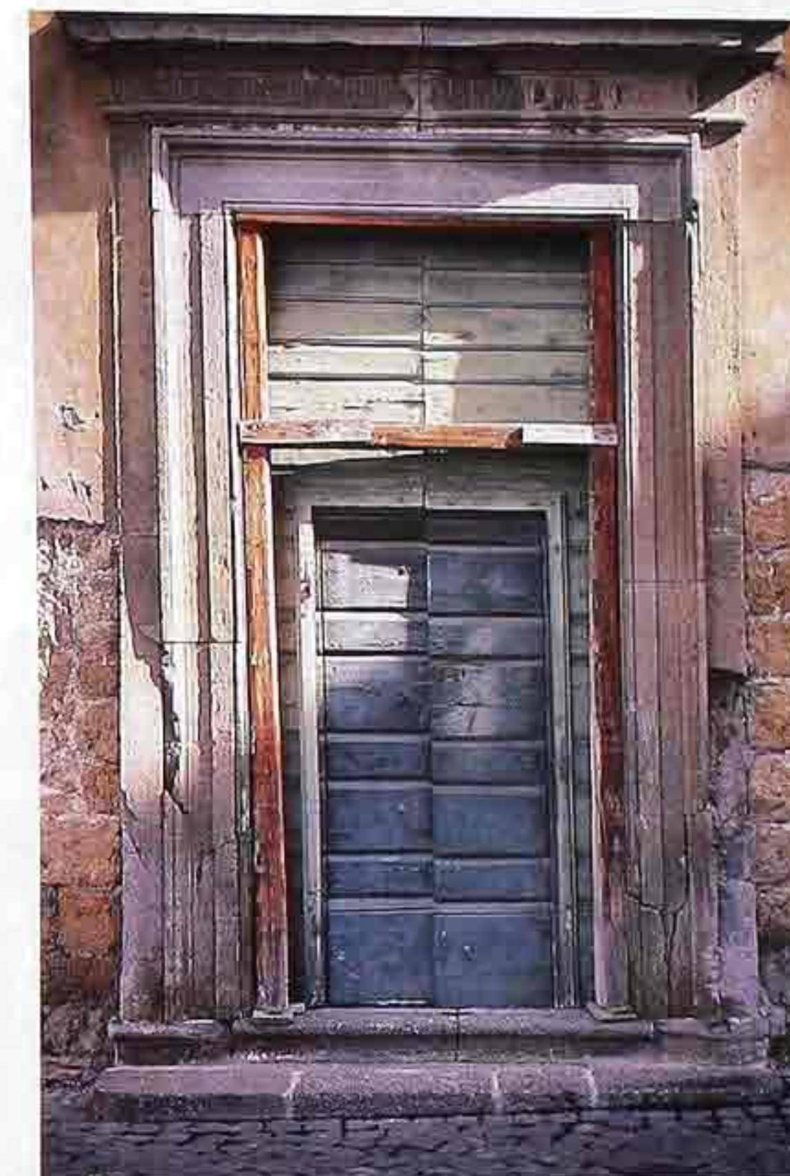
DW-105 Weathered entry with wood molding, transom panel, and painted paneled door
