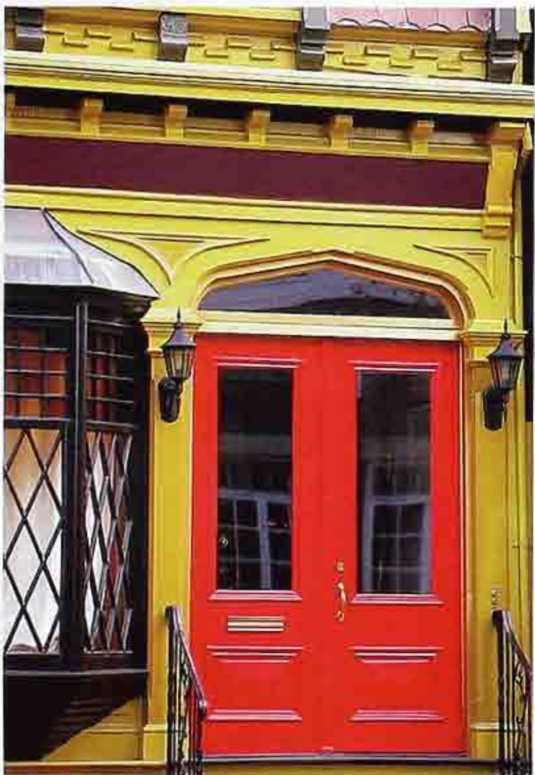
FA-77 Tudor-arch doorway and adjacent oriel painted with exterior gloss colors, 19th-c. storefront
