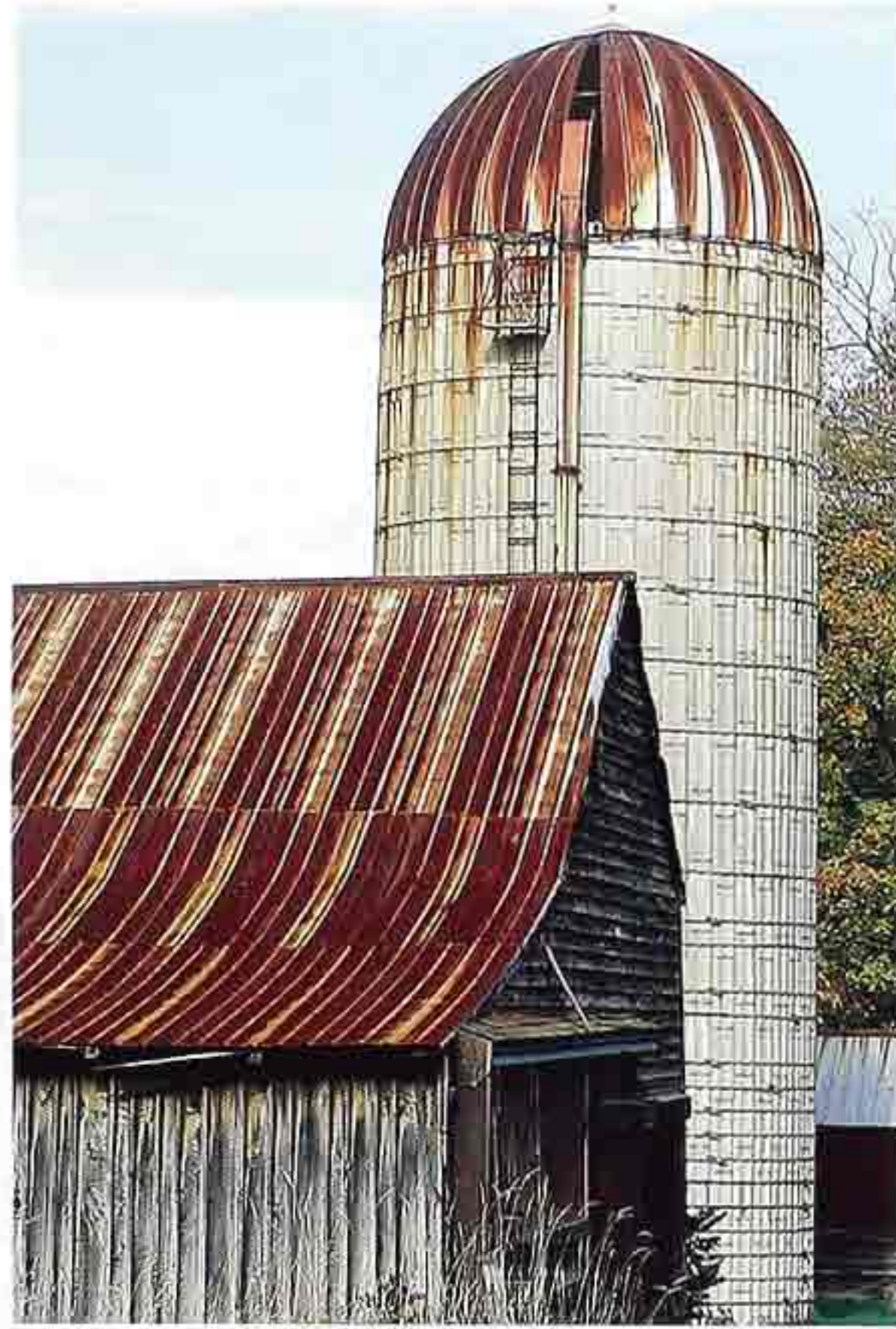
CR-37 Weathered corrugated metal roofs with flared gable on barn and domed roof on silo.
