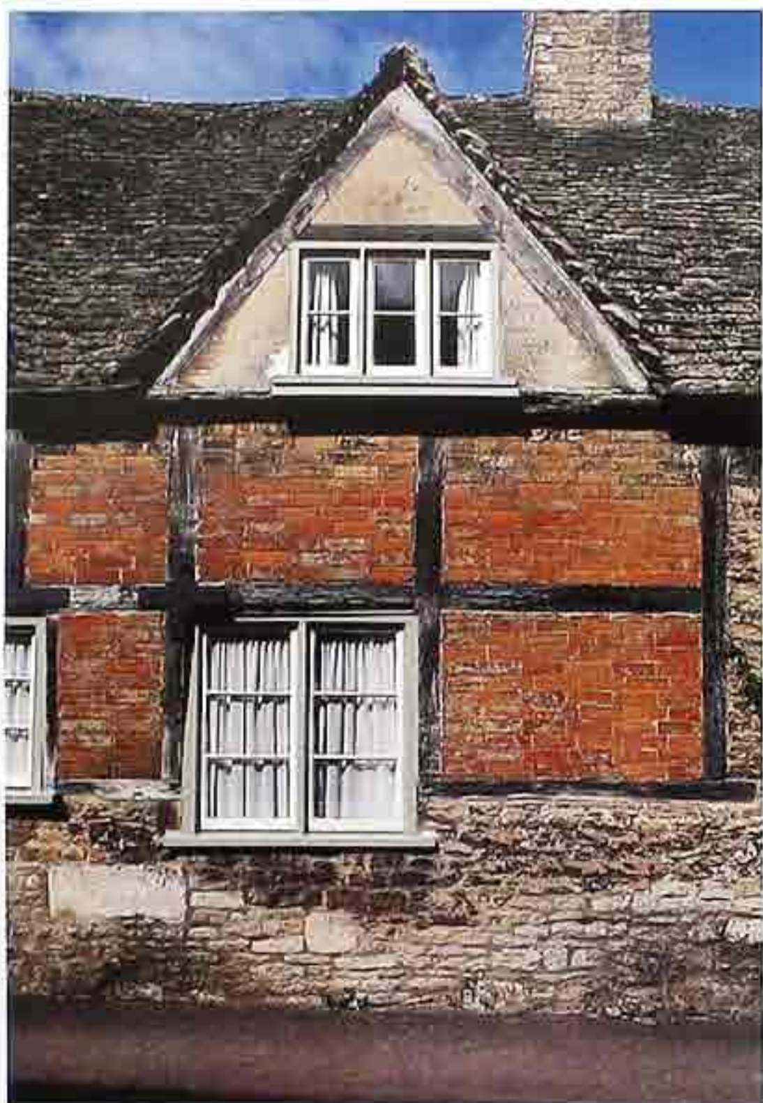
WA-282 Half-timber with brick infill; fieldstone first story, 16th- or 17th-c. English house
