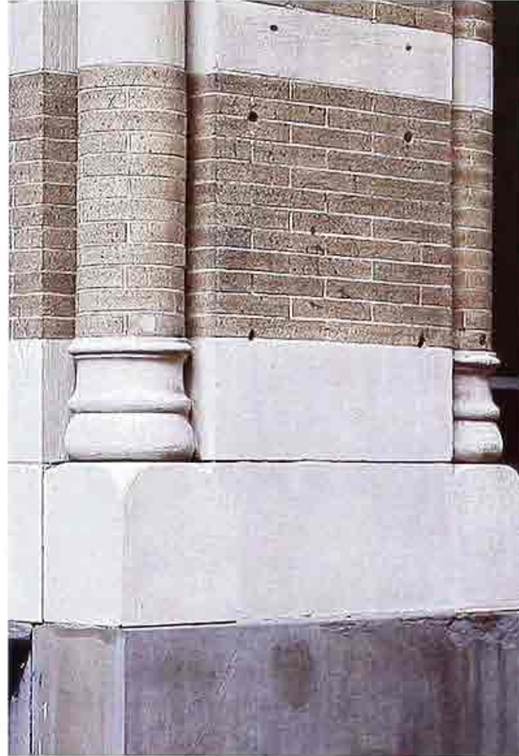
CP-42 Banded brick and stone jamb-shafts; base with shallow, elongated scotia over torus on plinth with scalloped corner
