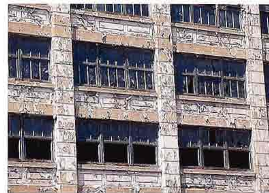
FA-98 Peeling paint on poured-in-place concrete frame with scored simulated masonry joints
