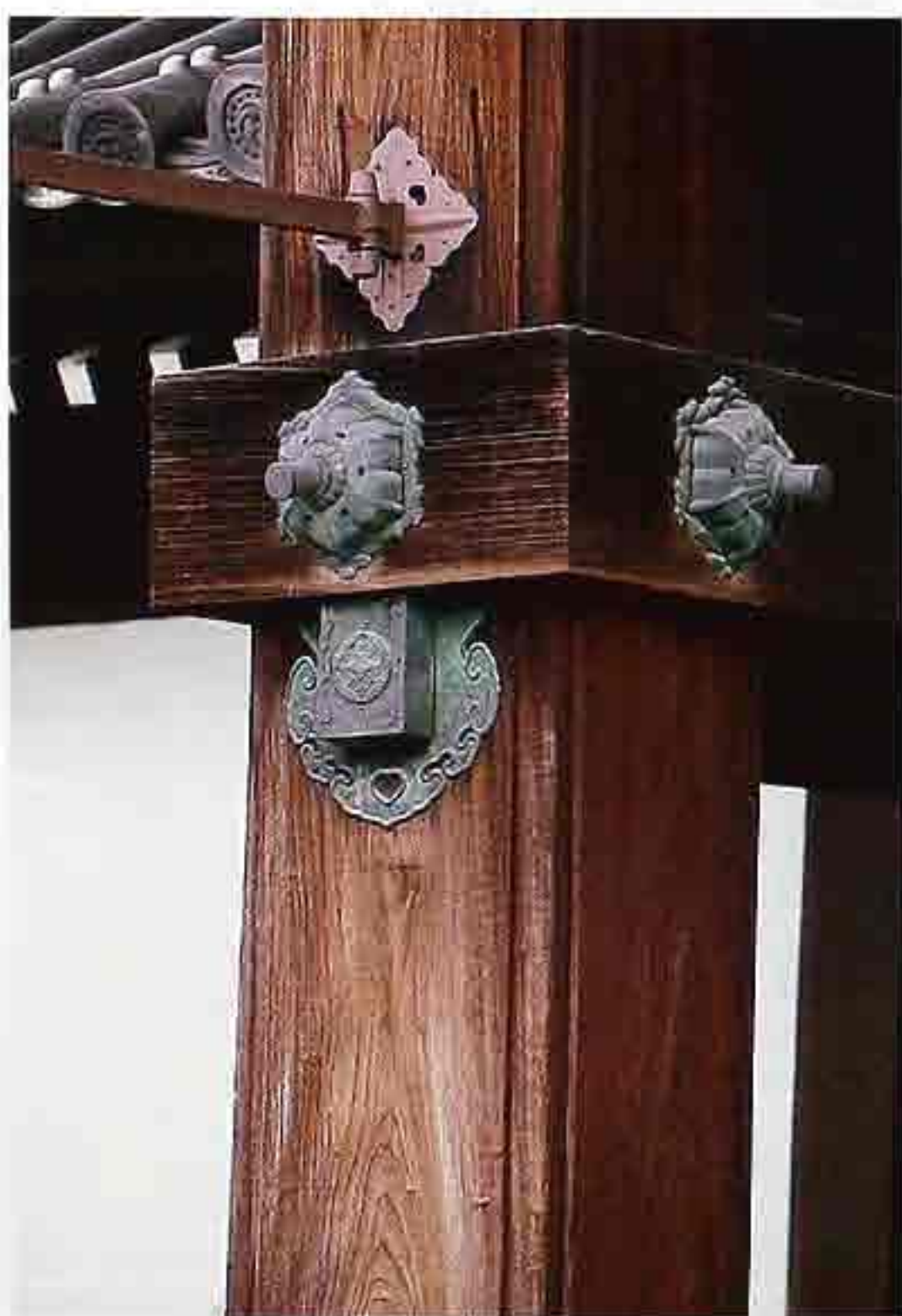
CP-107 Intersection of post and beam. Post appears to go directly through a mortise and is held in place by decorative tie irons.
