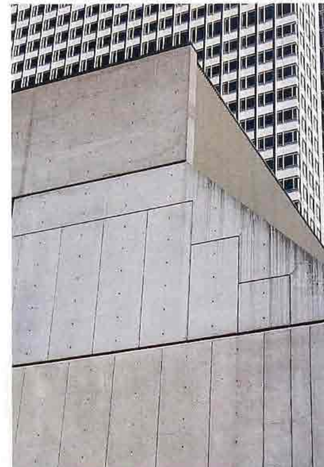
WA-210 Cast concrete with smooth finish, articulated formwork panels, and horizontal expansion joints
