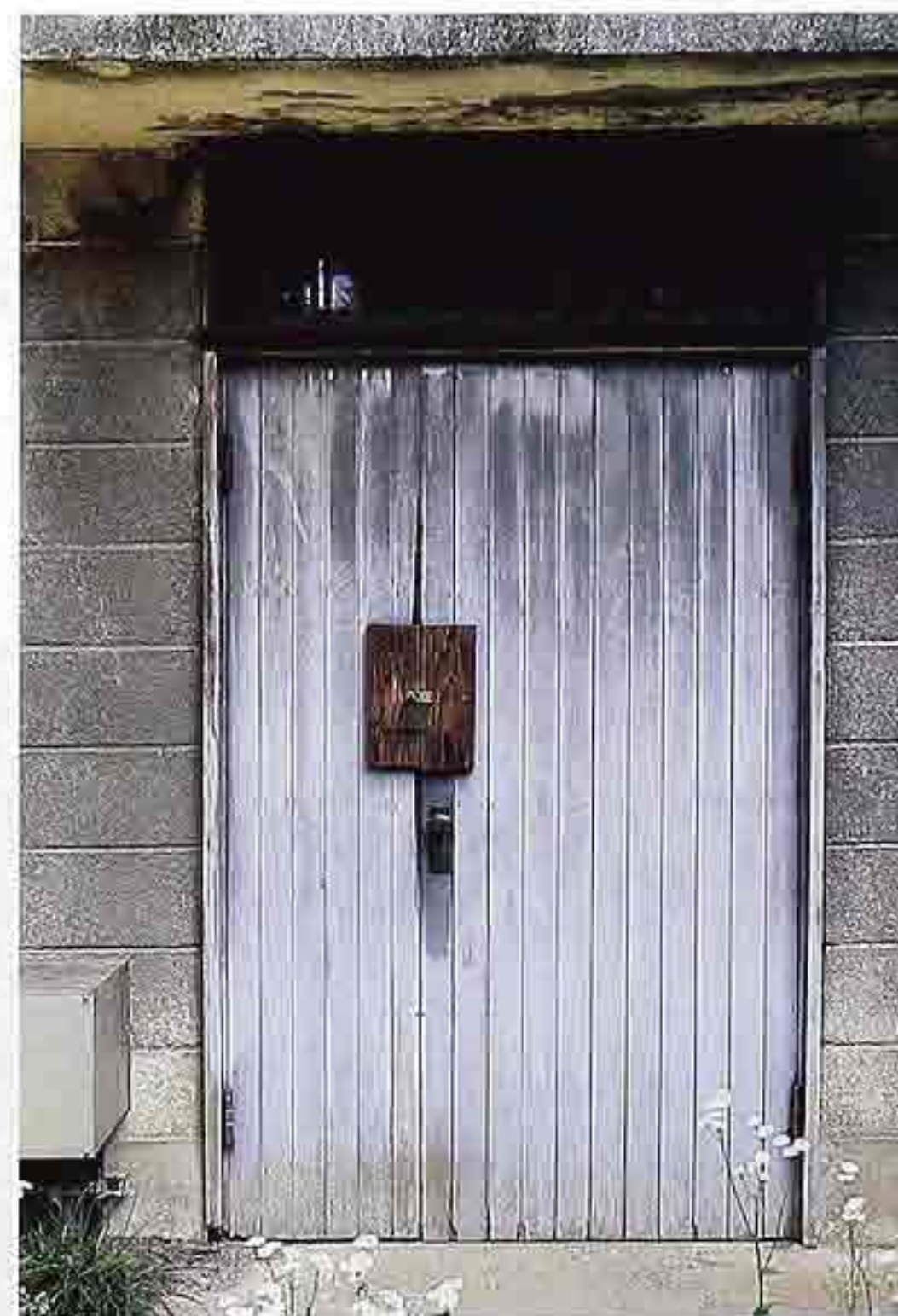
DW-35 Weathered whitewashed wood-plank double doors, concrete-block shed
