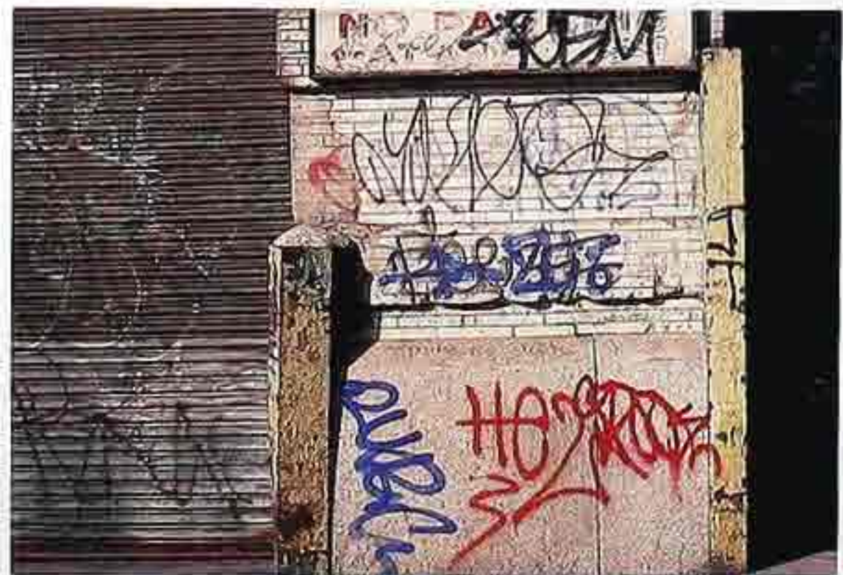
FA-107 Graffiti painted on brick pier between garage doors
