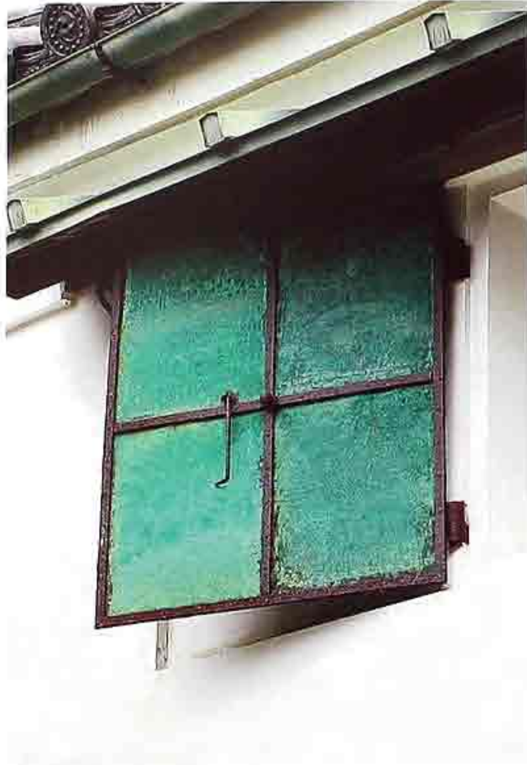
WI-194 Weathered painted metal shutter
