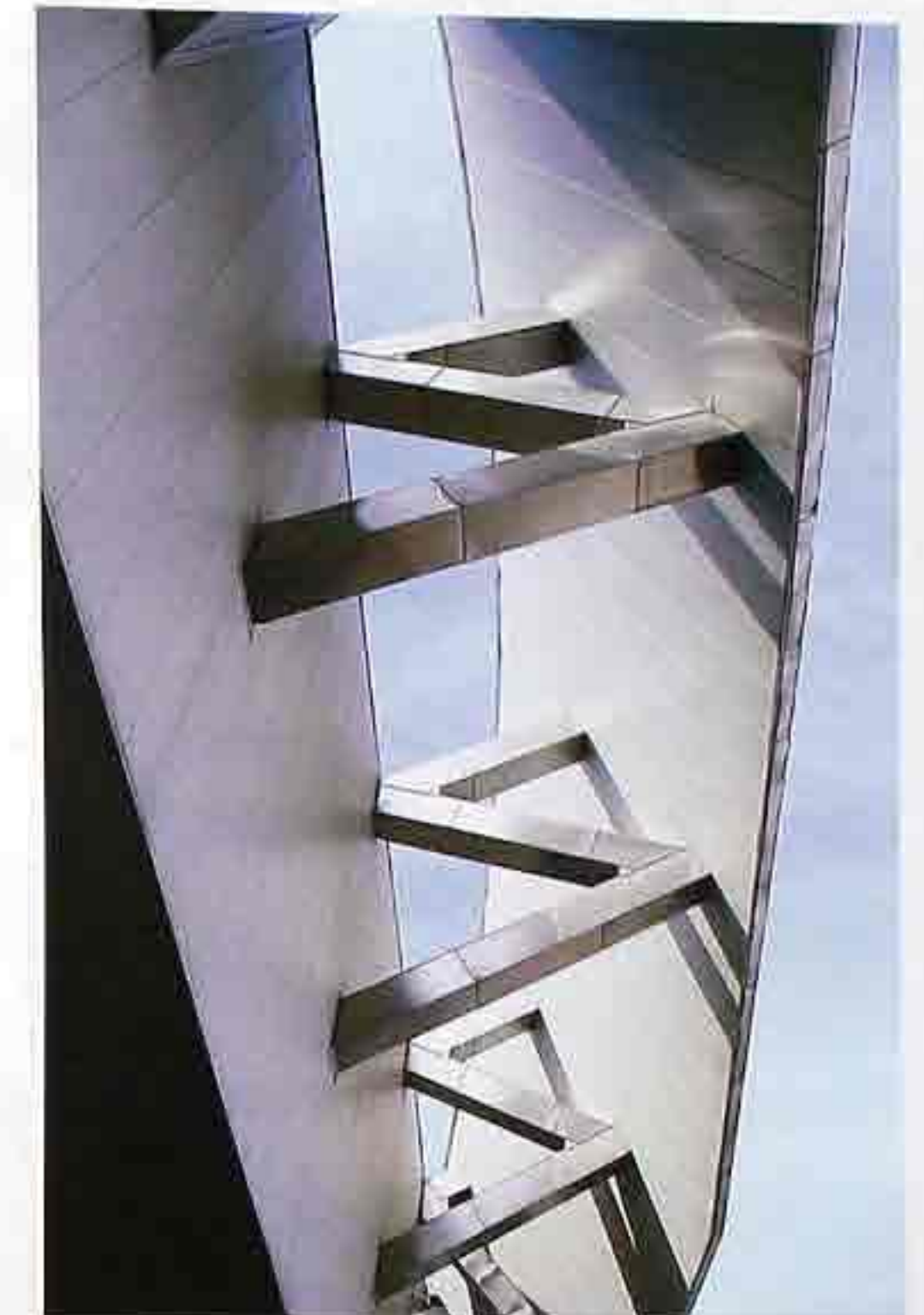
CR-110 Semidetached extension of metal roof connected to facade by Z-shaped brackets, modern commercial building
