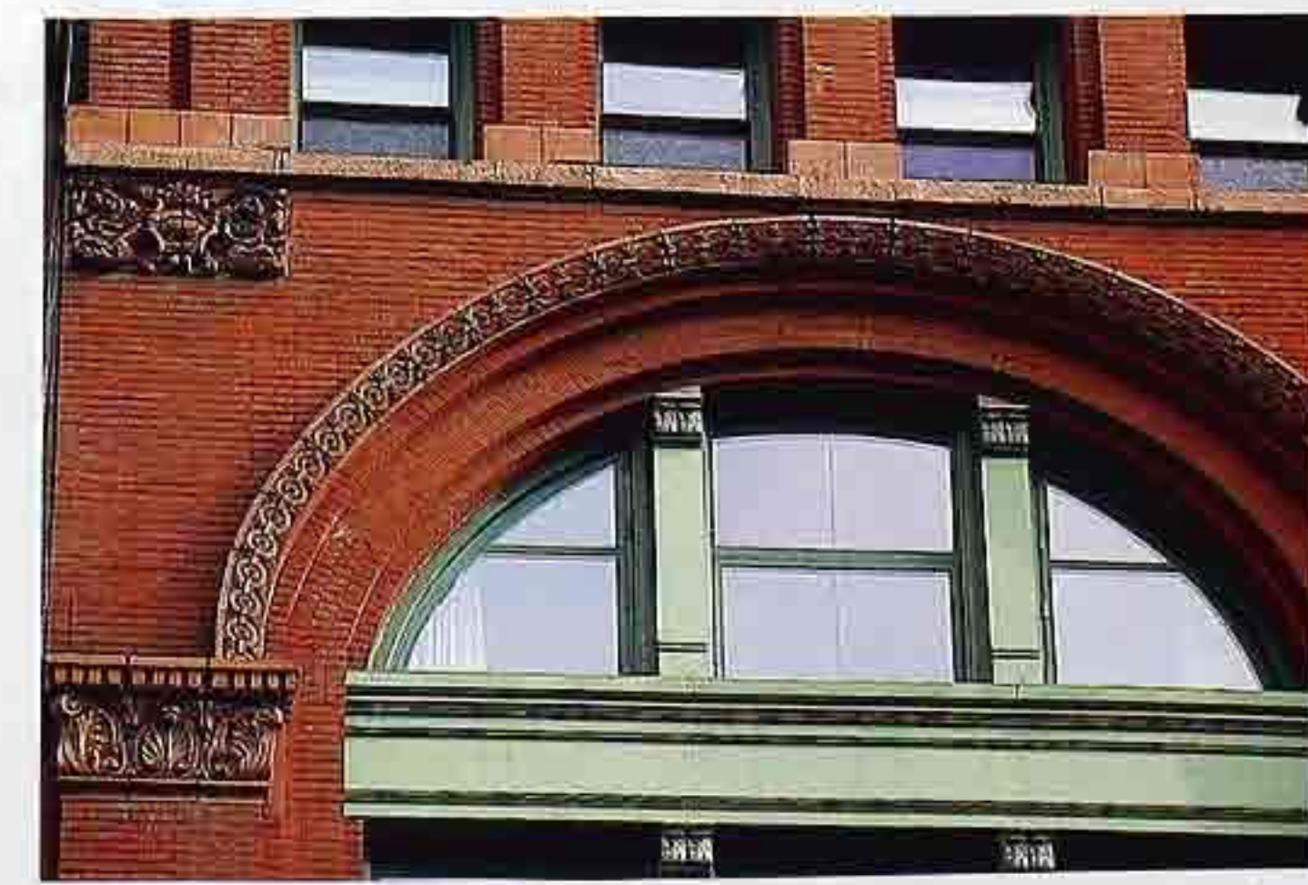
CP-161 Windows in semicircular arch; extrados with carved molding terminating at capitals
