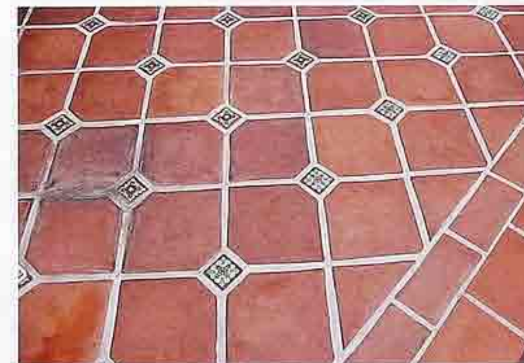
FP-99 Mexican paving tiles, straight-jointed, and inset with small decorated glazed tiles in diaper pattern, vertical-joint border (right)
