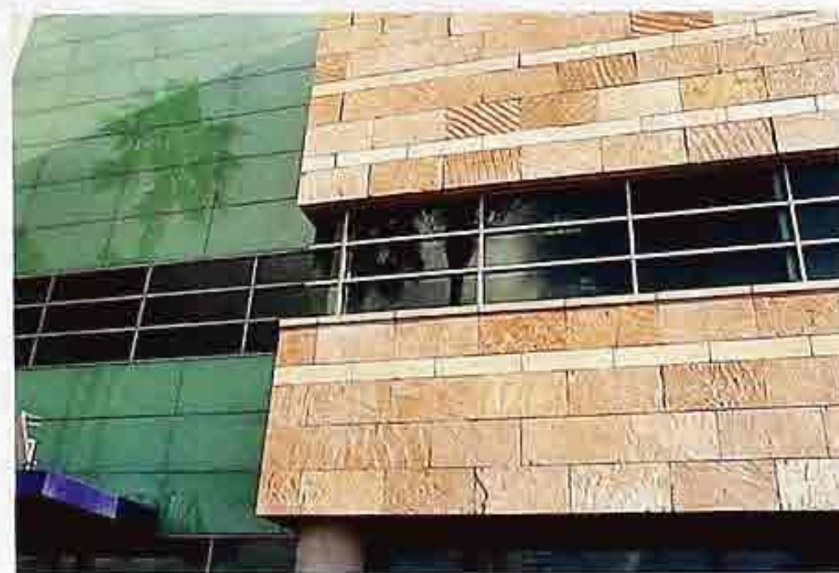
WA-299 Split-face sandstone veneer next to colored-glass or plexiglass-clad wing, modern commercial building
