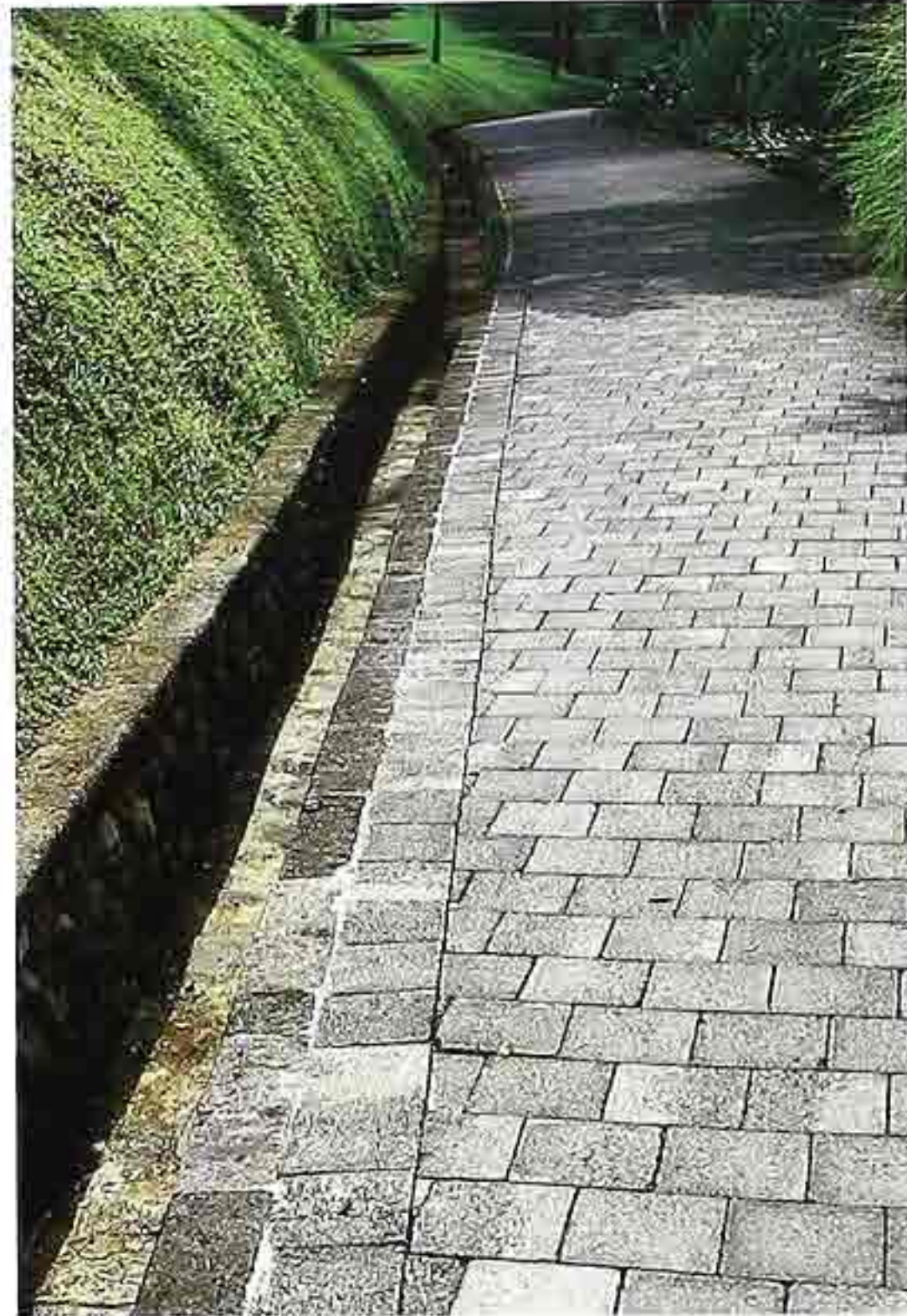
FP-20 Dimension fieldstone in running bond with soldier-course border and stone gutter, garden walkway
