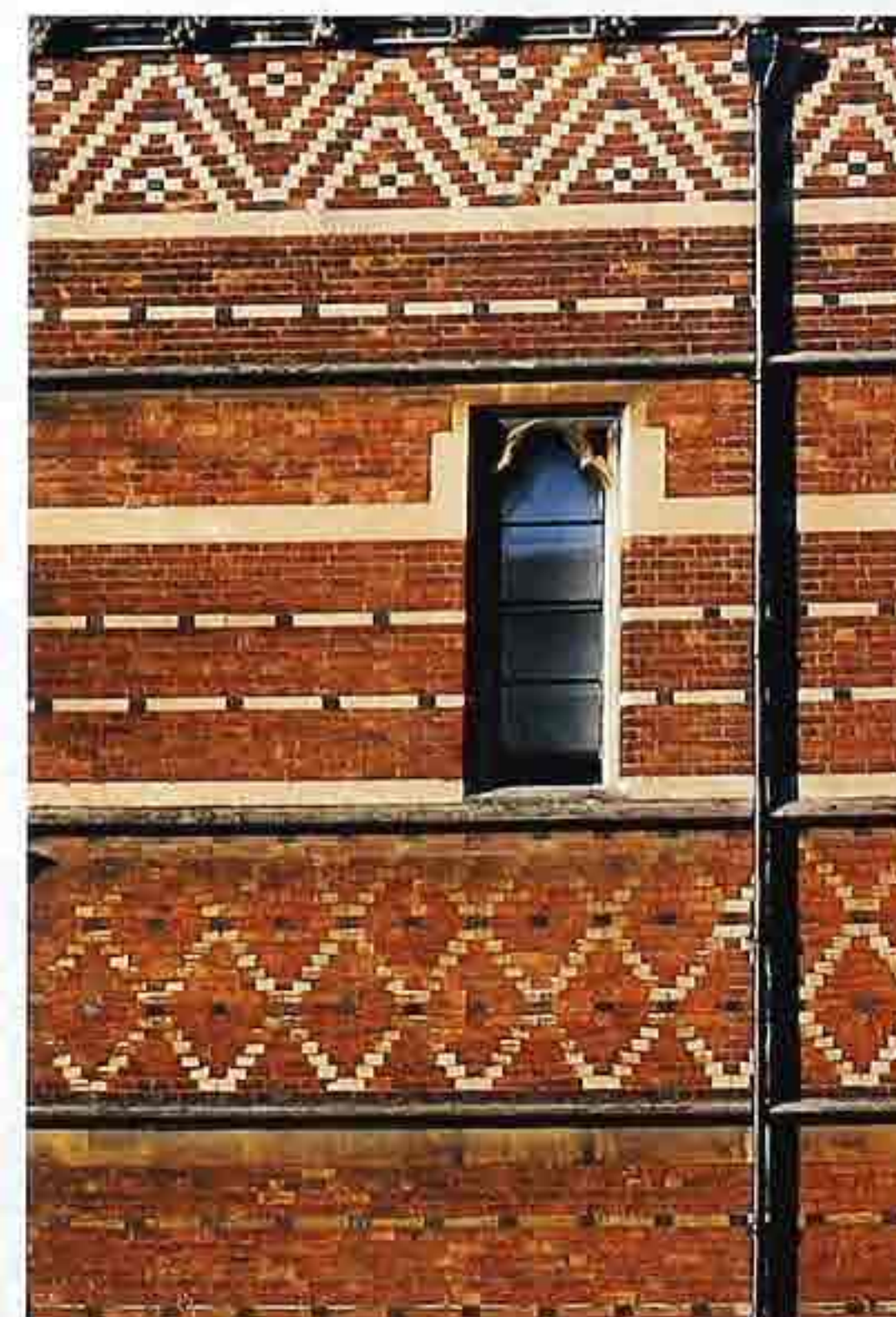
WA-203 Bands of decorative brickwork. Top to bottom: chevron, horizontal banding, diaper-work
