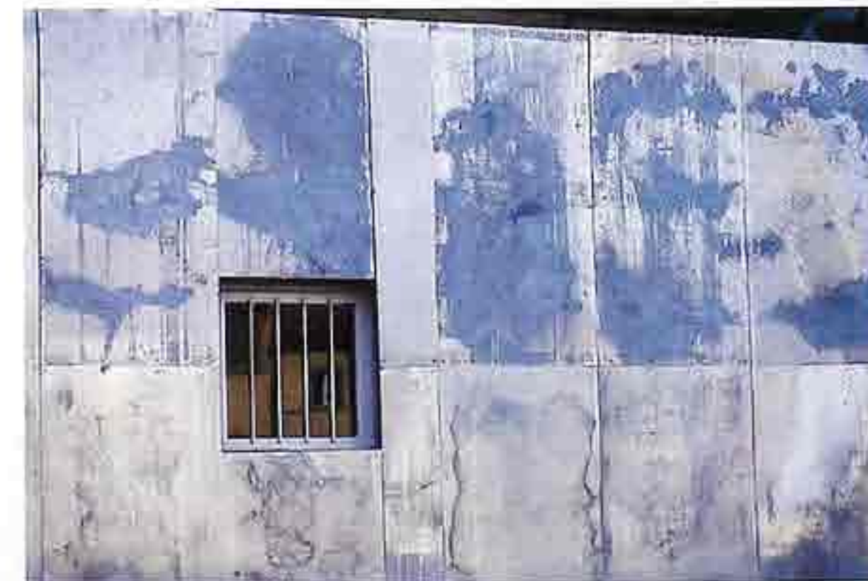
FA-6 Weathered flat metal panels with visible fasteners, probably lapped, exterior wall of industrial building
