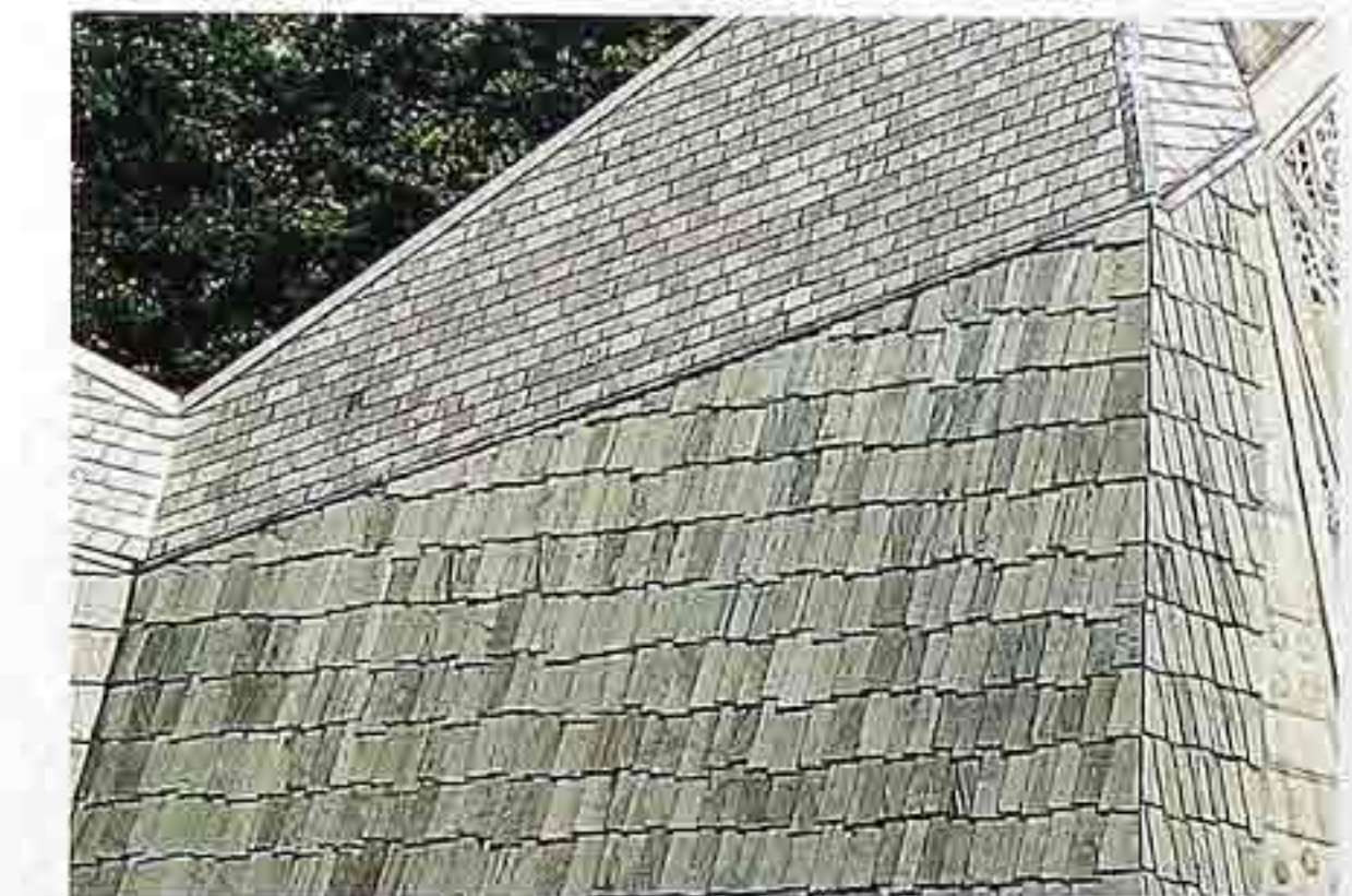
WA-129 Inside and outside corners of slate roof and cladding, modern commercial building
