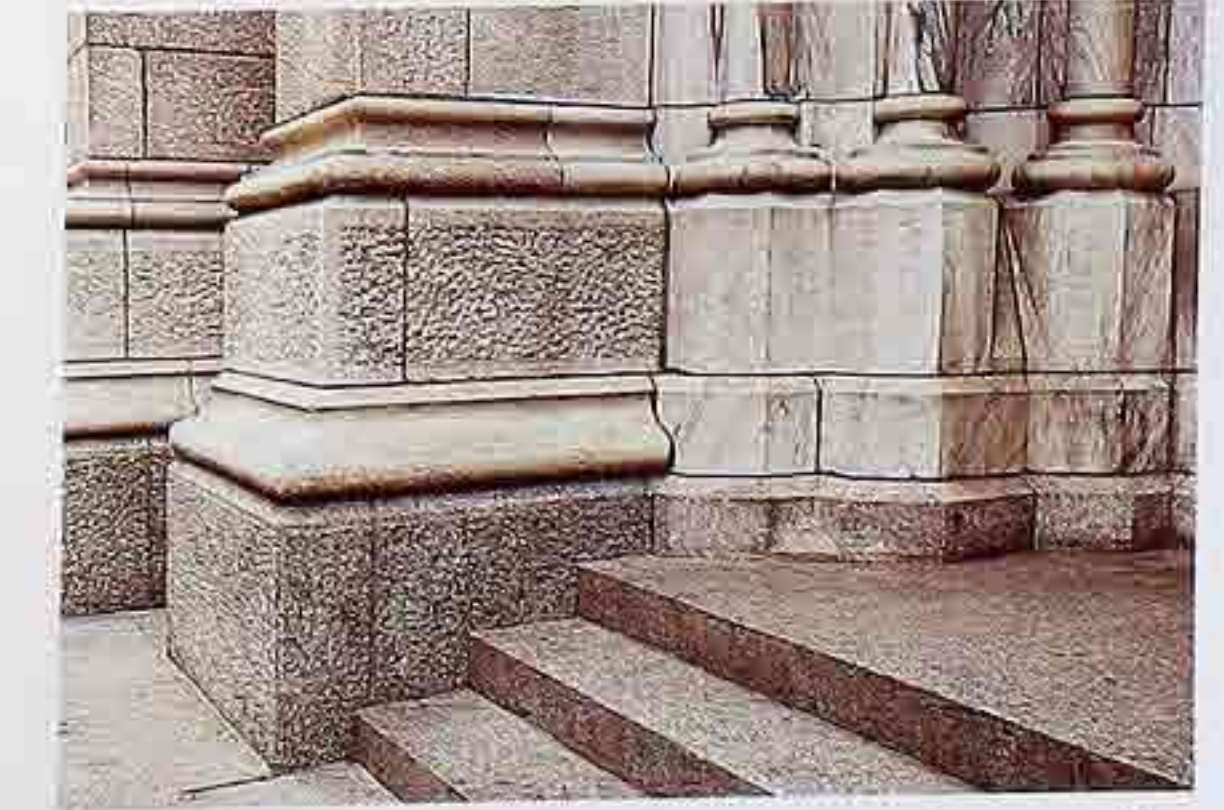
CP-40 Left: marble pier base with Attic profile and ogee molding below plinth; right: jamb-shafts with Attic-profile bases above plinths
