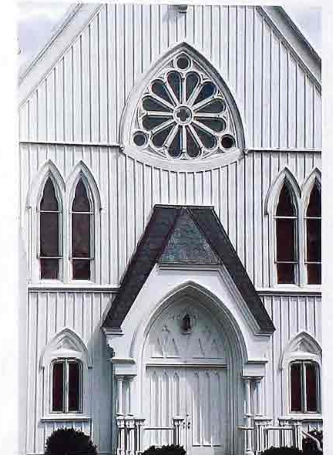
WA-33 Board-and-batten siding with rose window and lancet windows; jerkinhead-roofed entry, Carpenter Gothic church
