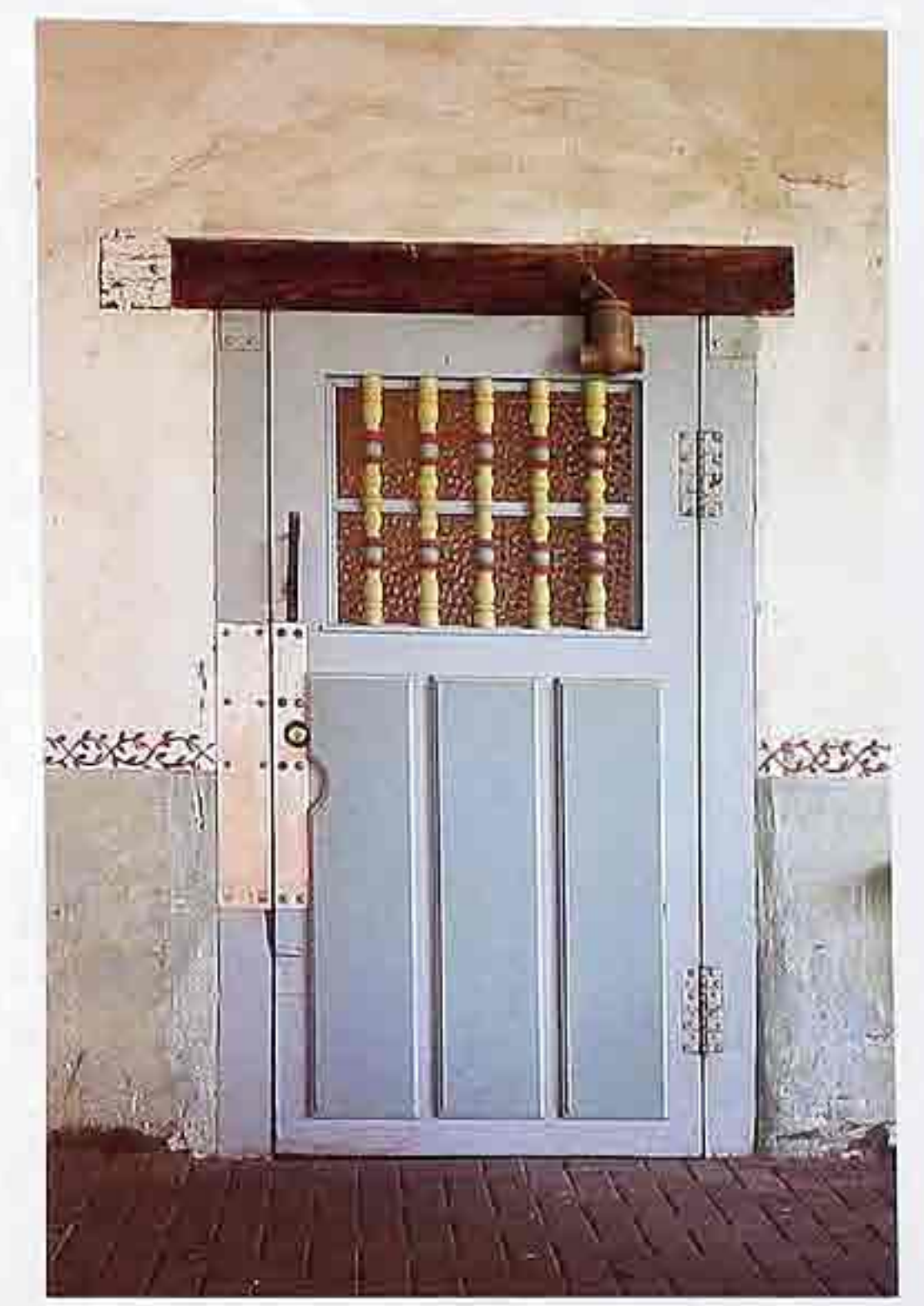
DW-42 Door with painted panels and grille of turned spindles; stucco adobe doorway with exposed timber lintel, American Southwestern mission
