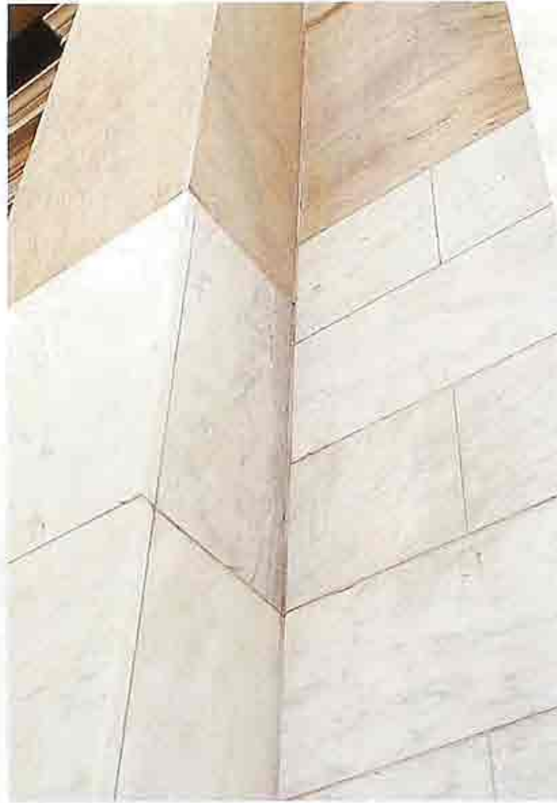
WA-97 Inside corner of honed-veener marble in running bond, bottom recently cleaned
