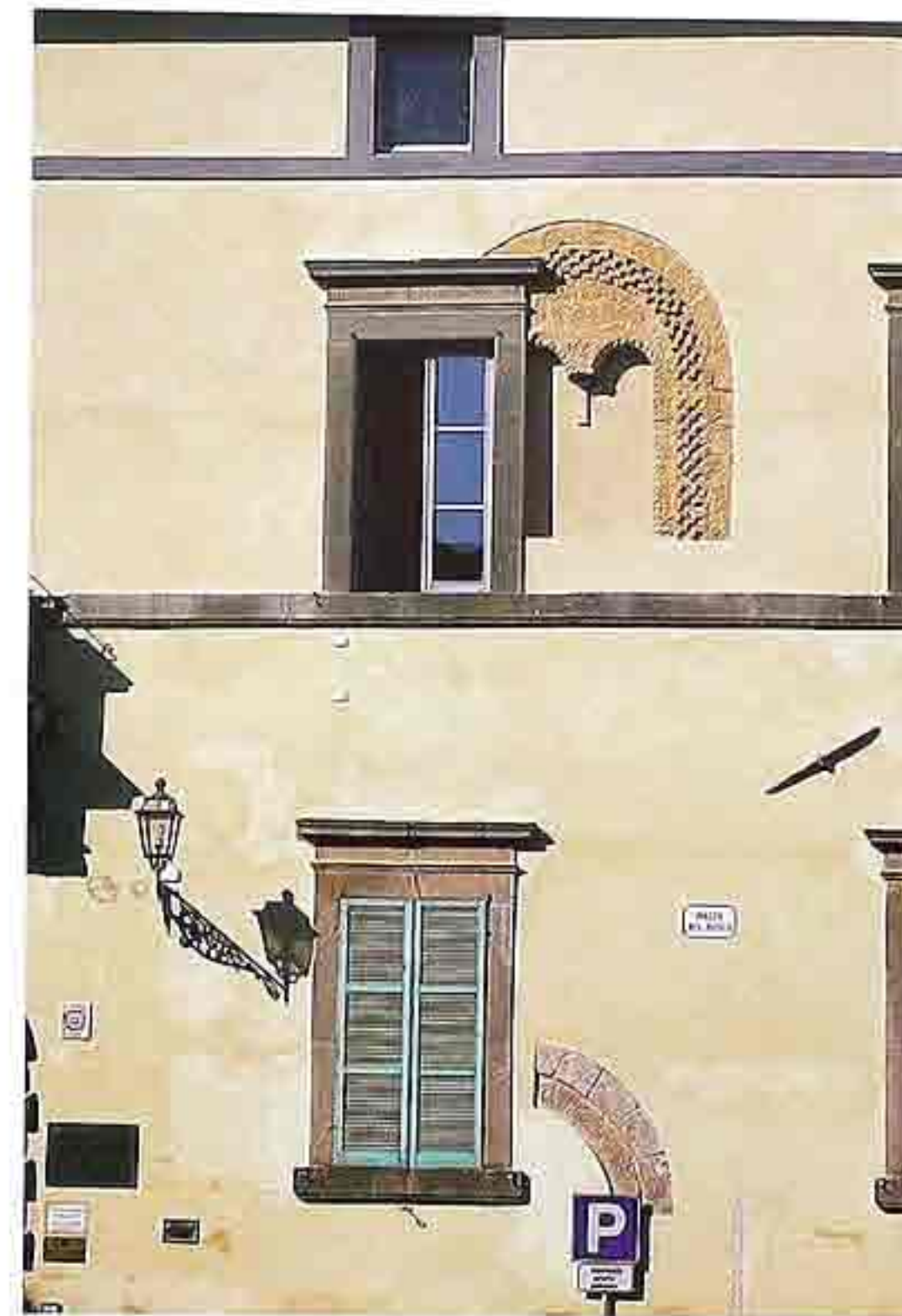
FA-115 Stucco facade with older arches embedded in the wall adjacent to modern windows
