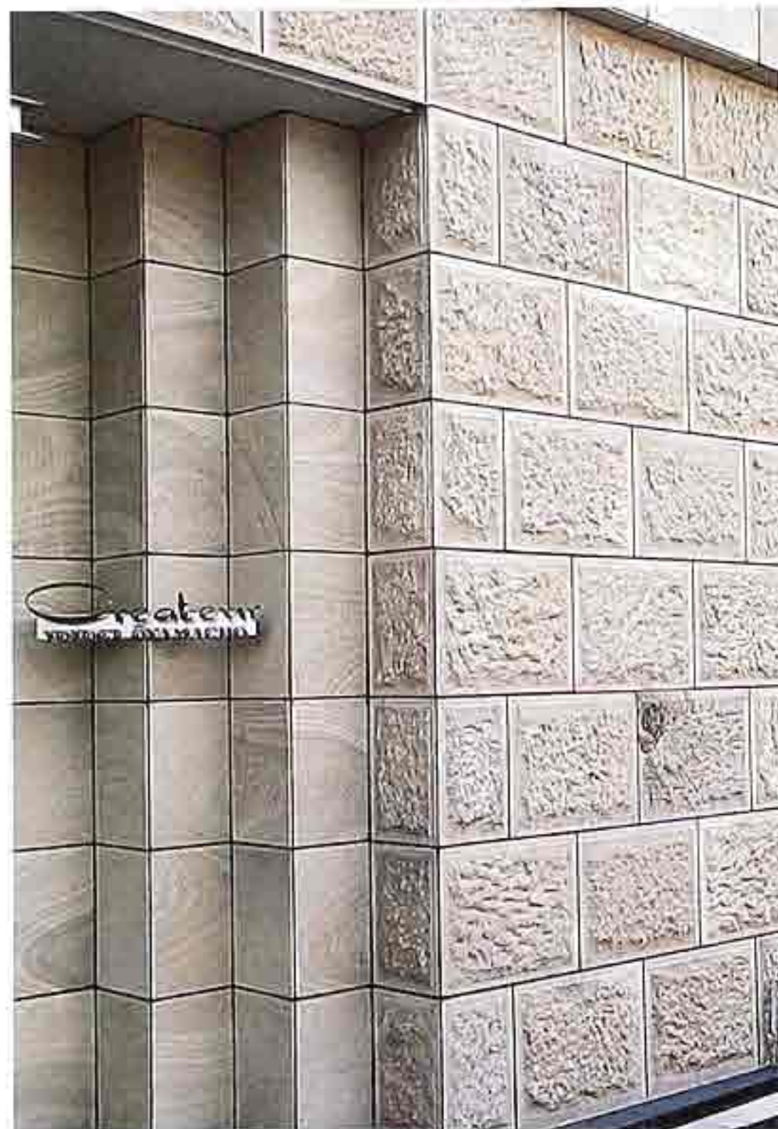
WA-132 Corner of rusticated running bond with reveal; sand-finish pilaster strips in stack bond on entry, modern commercial building
