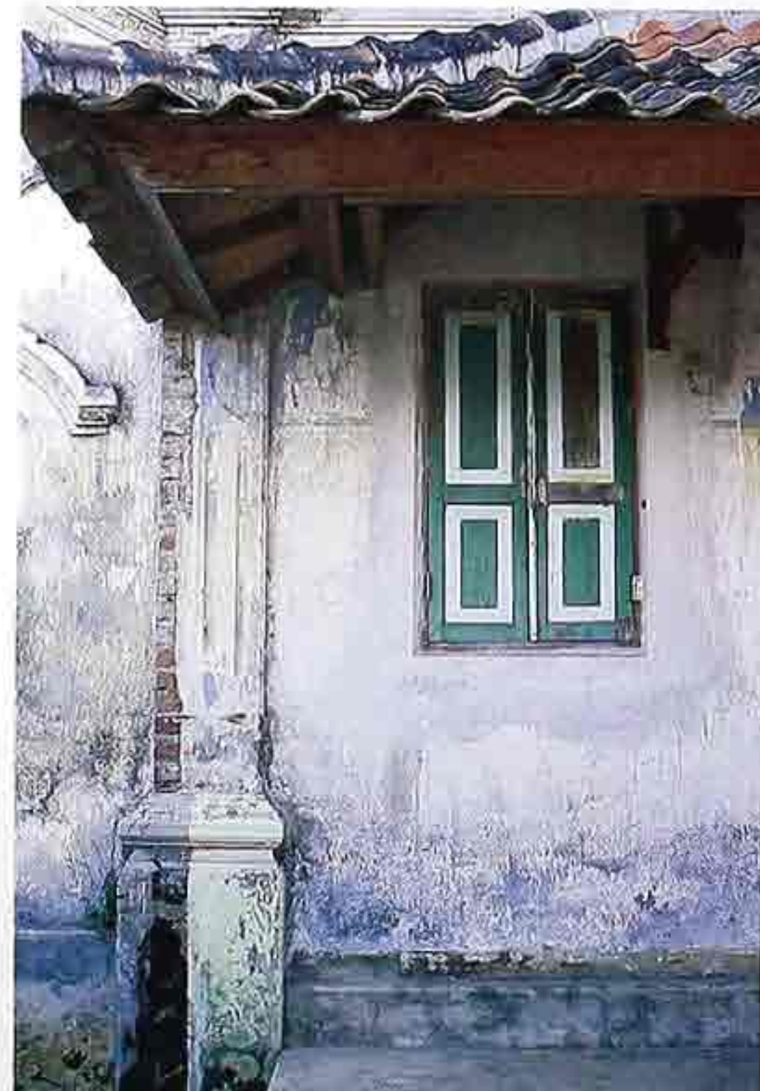
FA-95 Weathered painted stucco over brick
