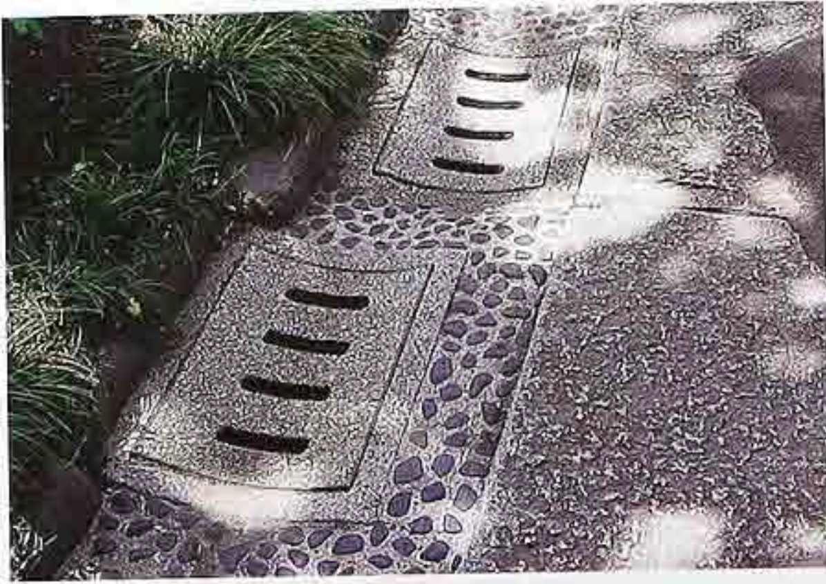
FP-113 Pre-cast exposed-aggregate drain grates in gutter beside a walkway, urban park
