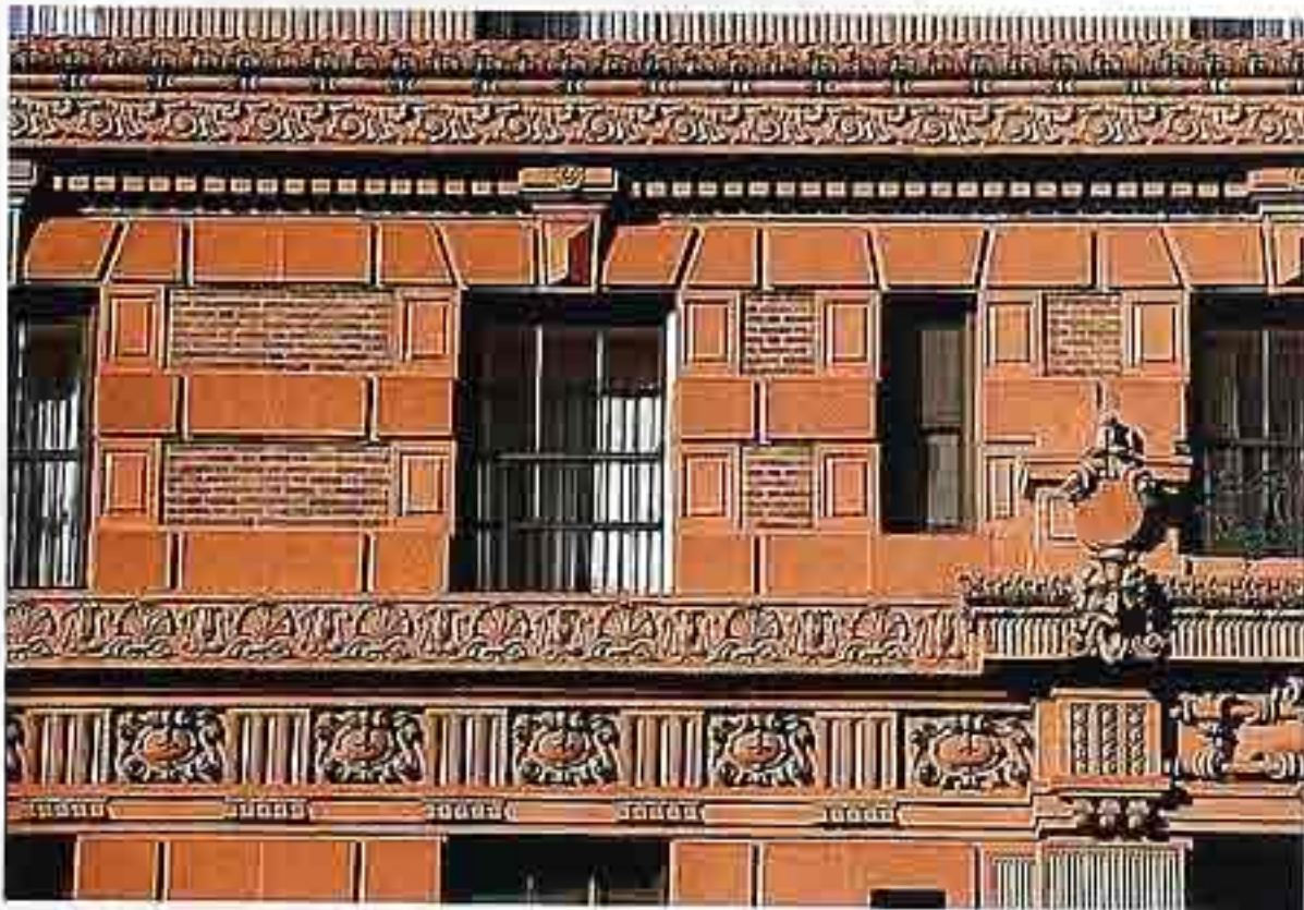
FA-121 Brick facade with rusticated and heavy embellishment in brownstone or terracotta
