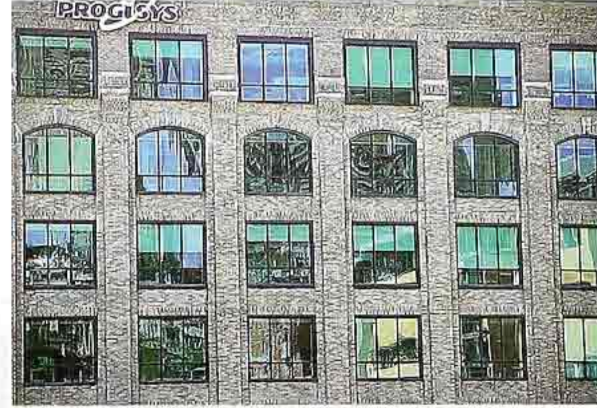
WI-159 Banded fenestration: row of arched windows and rows of square windows; metal replacement windows, 19th-c. industrial building
