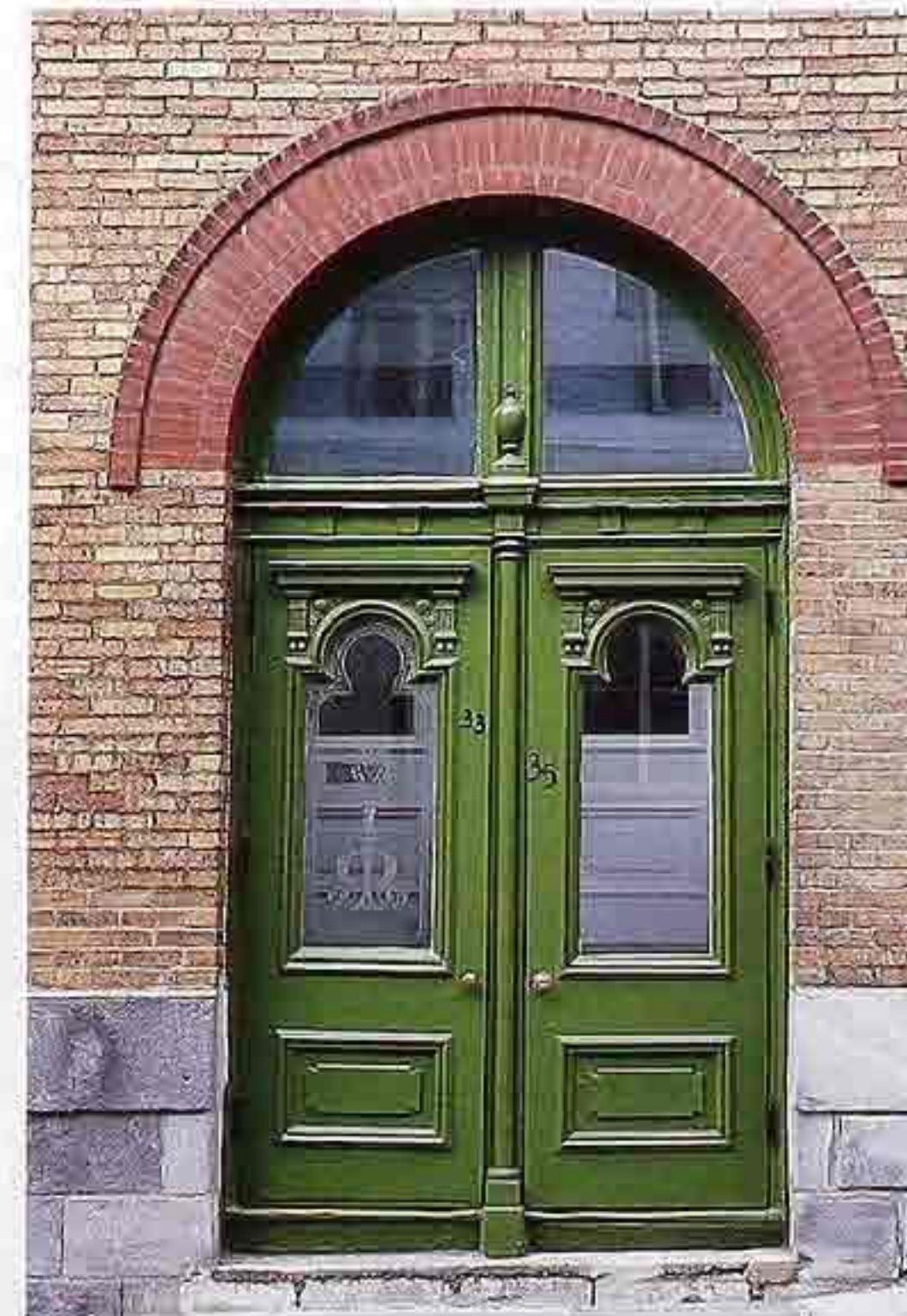
DW-21 Wood double doors with glass upper panels and flush-molded lower panels; split transom light in segment
