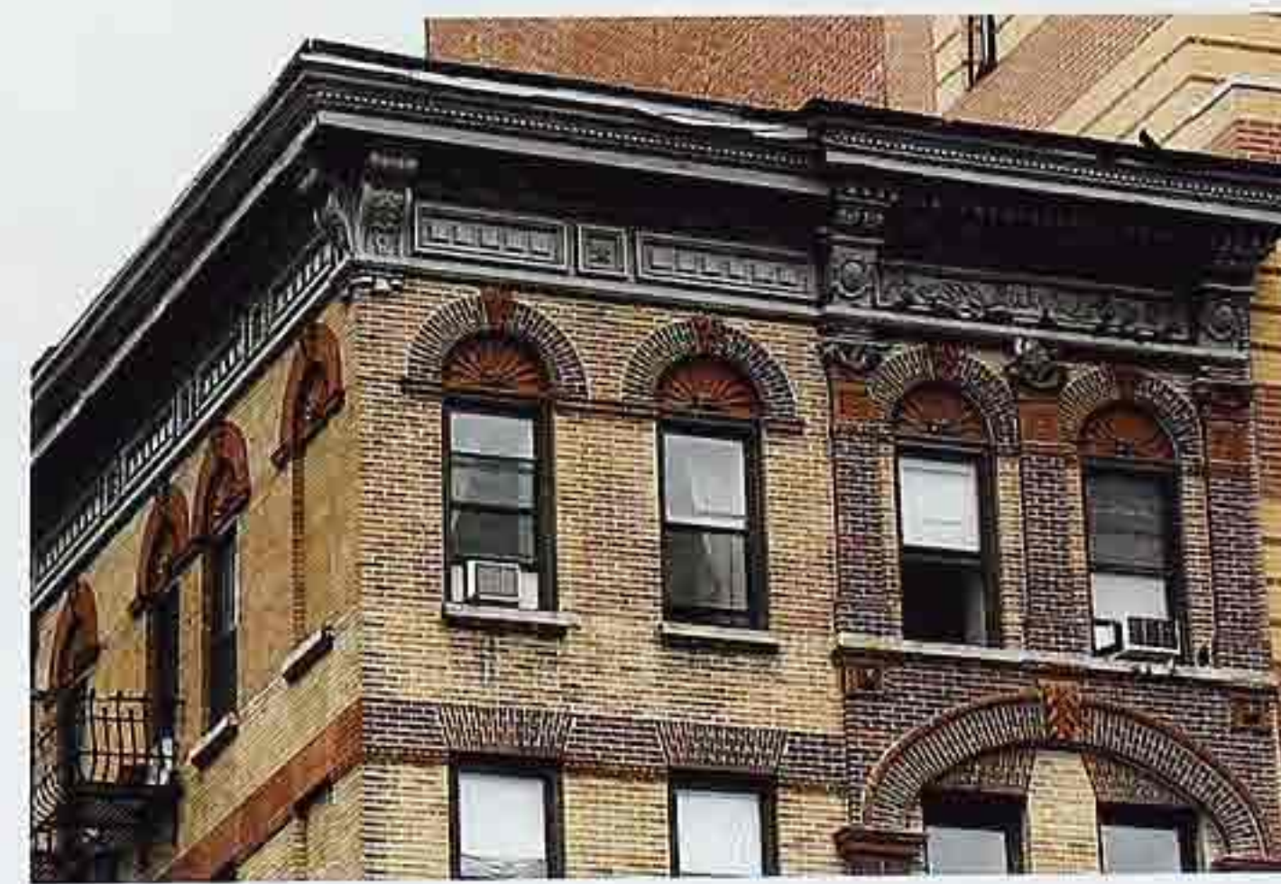
WA-188 Contrasting brick banding and pilasters; gauged-brick semicircular arches on upper windows, 19th-c. apartment house
