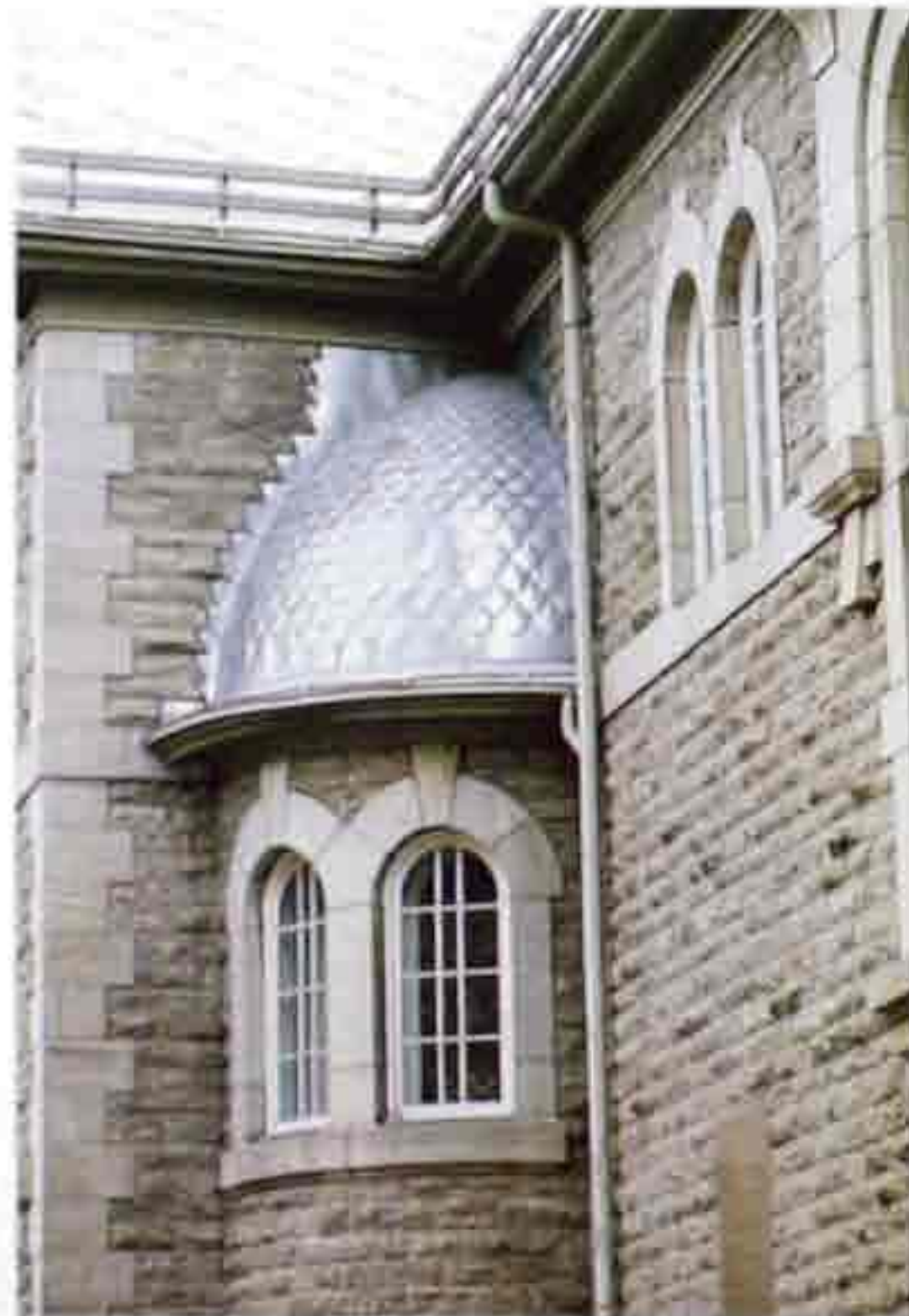
CR-32 Quilted sheet metal on dome roof of corner turret with flashing at juncture of dome and wall
