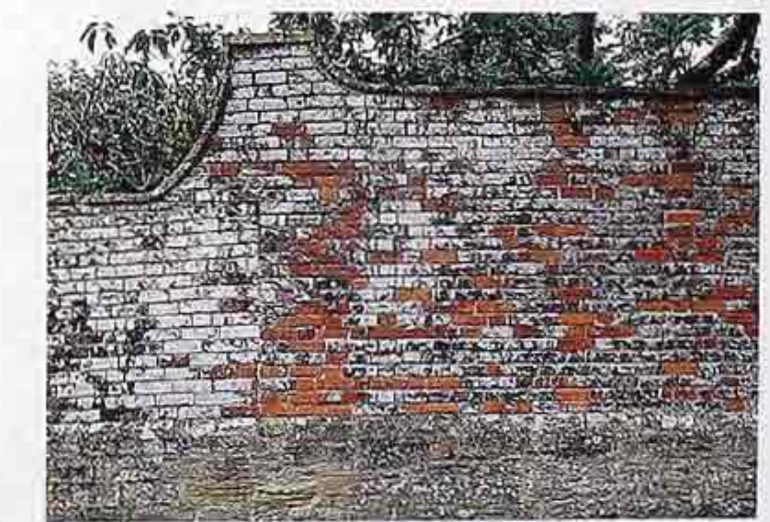
FA-99 Peeling paint on brick garden wall with stone base
