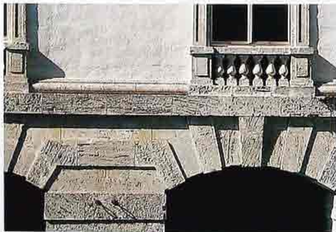
WA-116 Sawn fossil-stone in coursed ashlar with raised voussoirs; engaged balustrade with bead base molding above belt course
