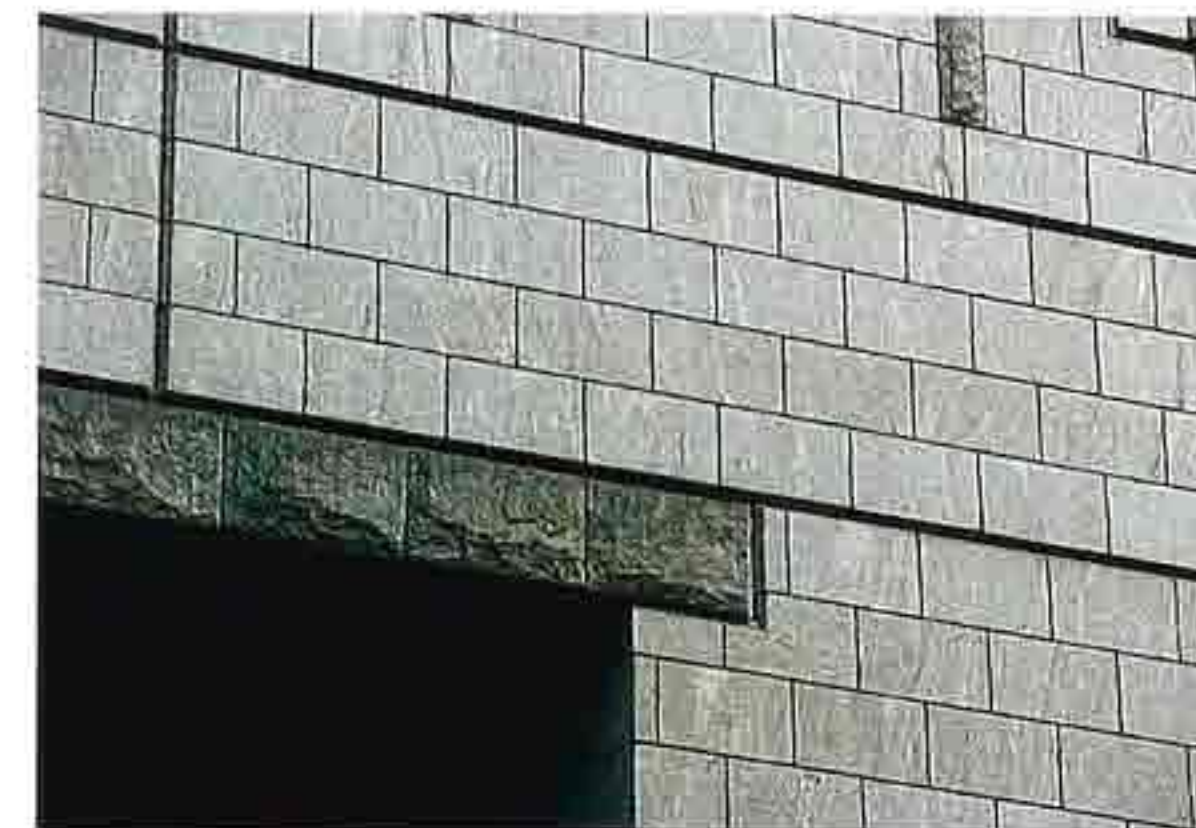
WA-128 Rock-face granite doorway lintel with contrasting sawn-granite panels in running bond with wide V-shaped joints
