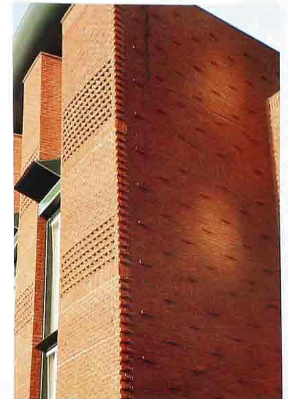
WA-194 Corner detail of custom bond with dog-tooth banding and diaper pattern of projecting stretchers, modern apartment house
