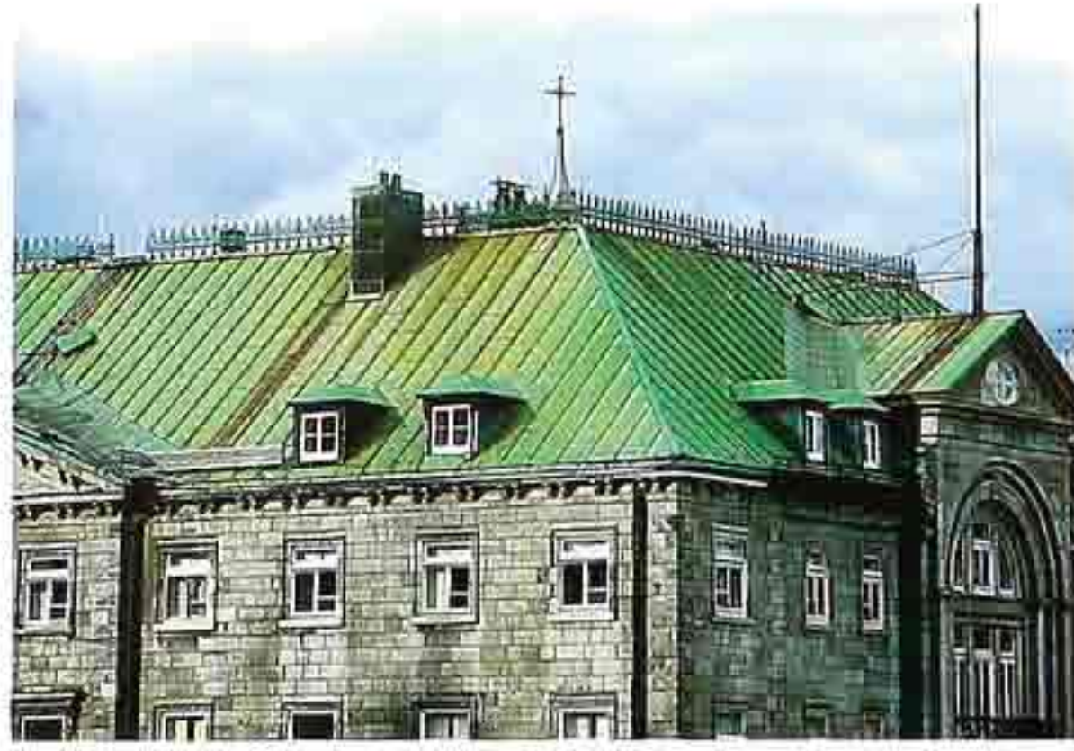
CR-115 Hipped, copper with standing seams; hipped-roof dormers (left) and pedimented wall dormer (right)
