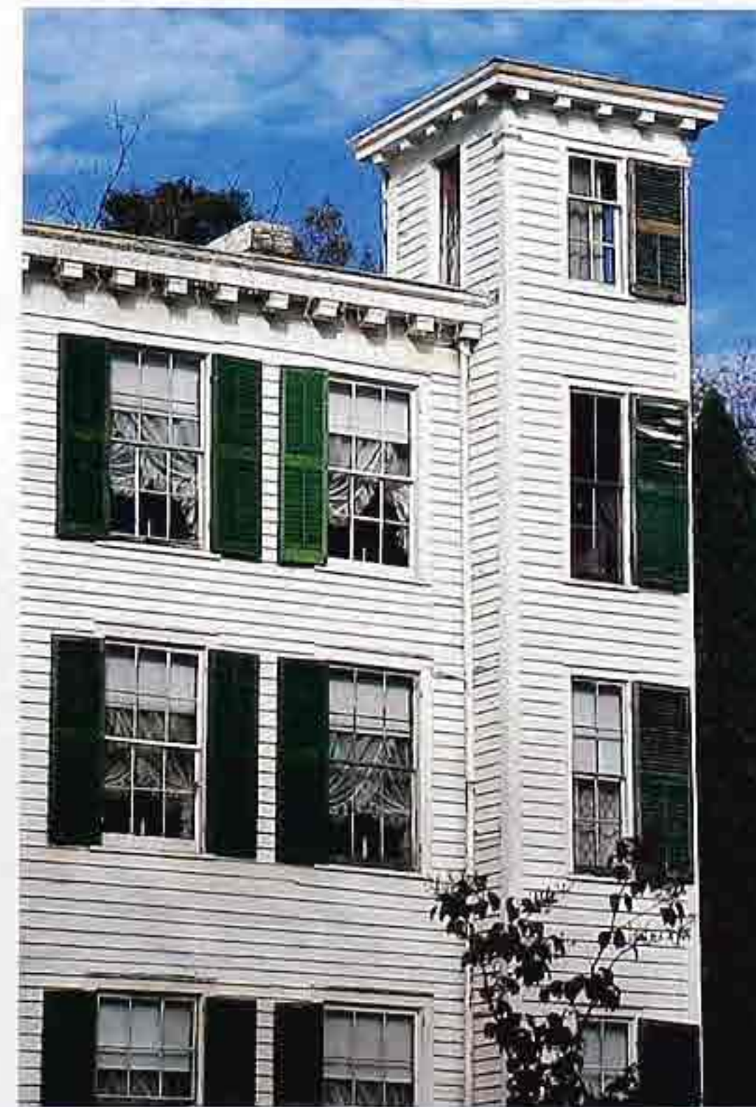
WA-34 Painted clapboard and block modillion cornice on corner tower, Italianate house
