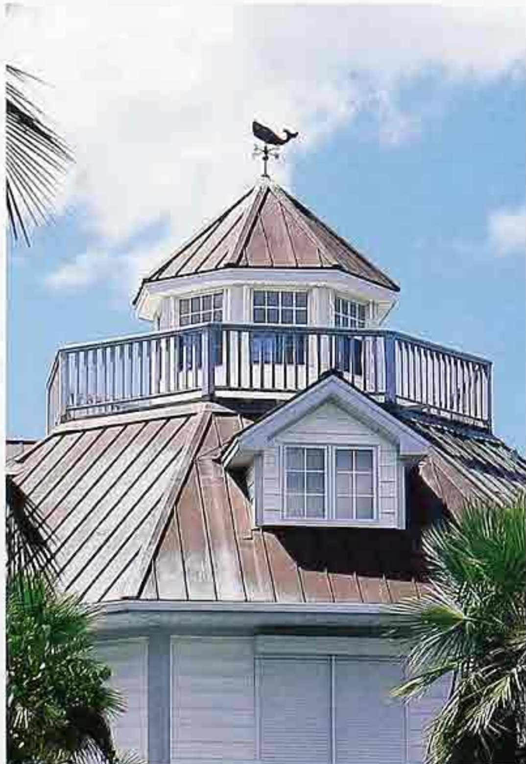
CR-128 Octagonal painted standing-seam metal roof with widow's walk and gabled roof dormer
