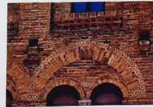
WA-164 Medieval arcade under relieving arch in gauged brick with chevron-decorated extrados and recessed spandrels
