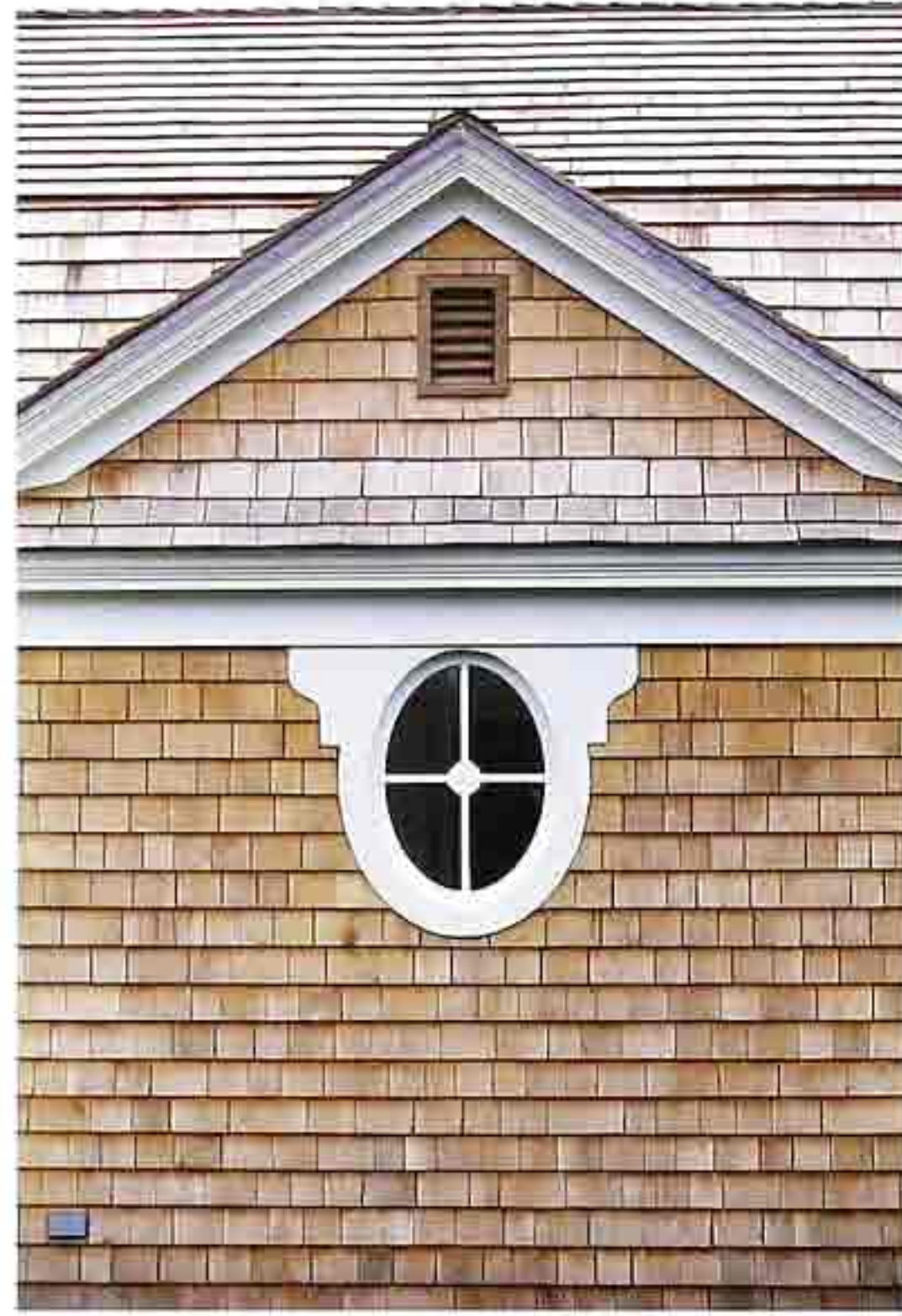
WI-66 Oval window divided by muntins, with flat wood casing in white cedar-shingle gable wall
