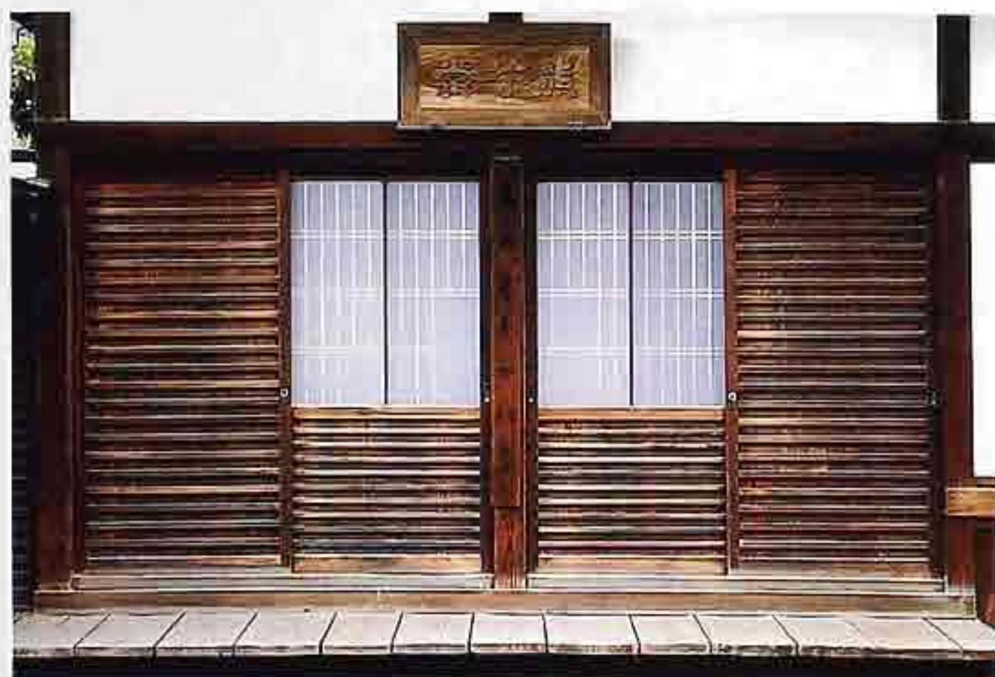
WA-46 Timber frame with infill of planks and battens with sliding doors and paper-covered windows
