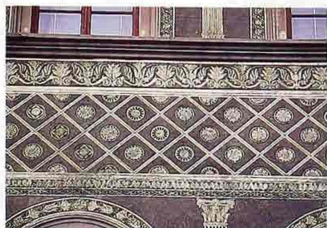
FA-87 Sgraffito depicting pilasters, enriched archivolt, classical moldings, reticulated band with paterae on wall, Italy
