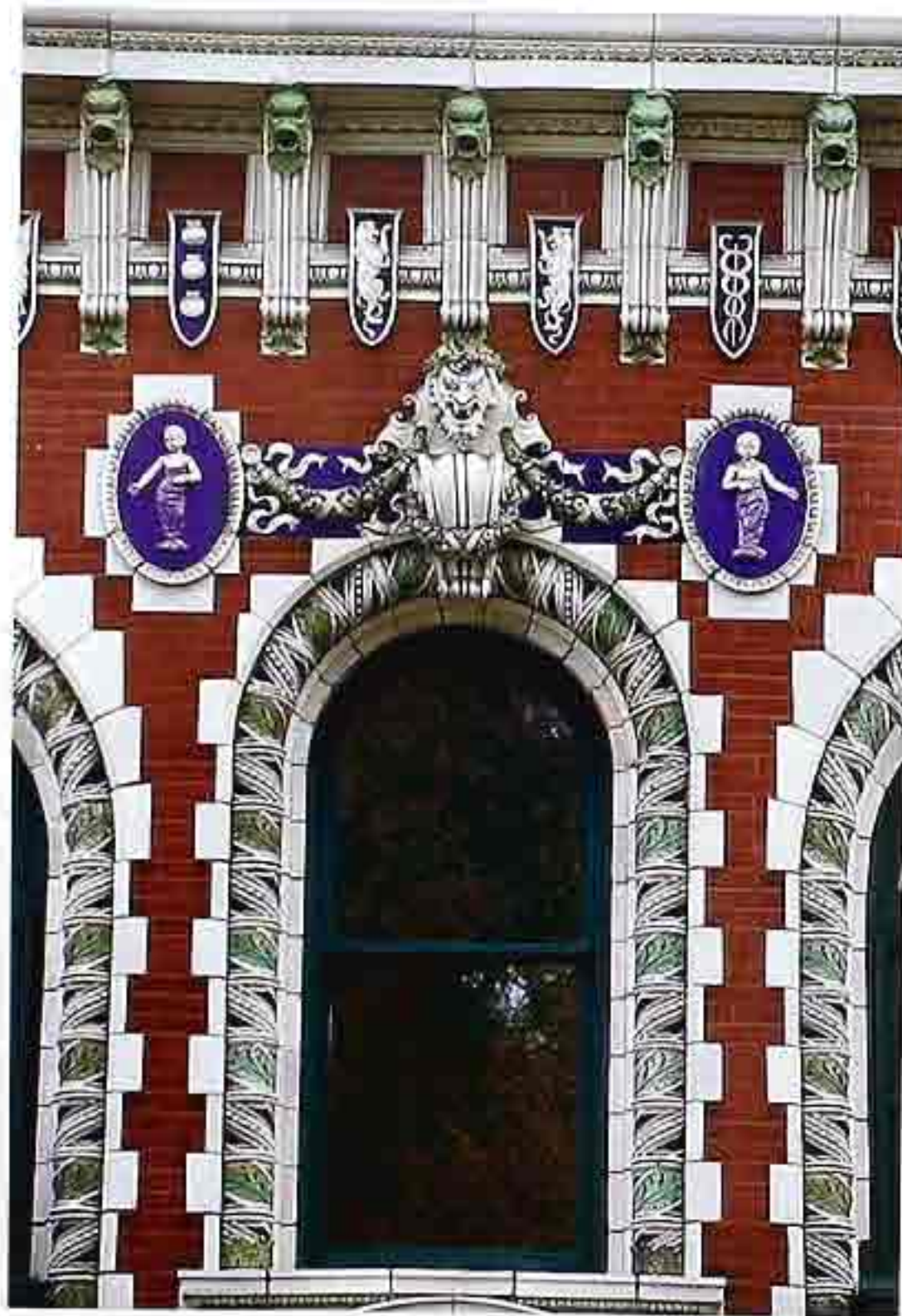
FA-59 Brick facade with polychrome glazed ornamental details: bracket cornice, cartouches, garlands, ancon, and rope molding around semicircular windows.
