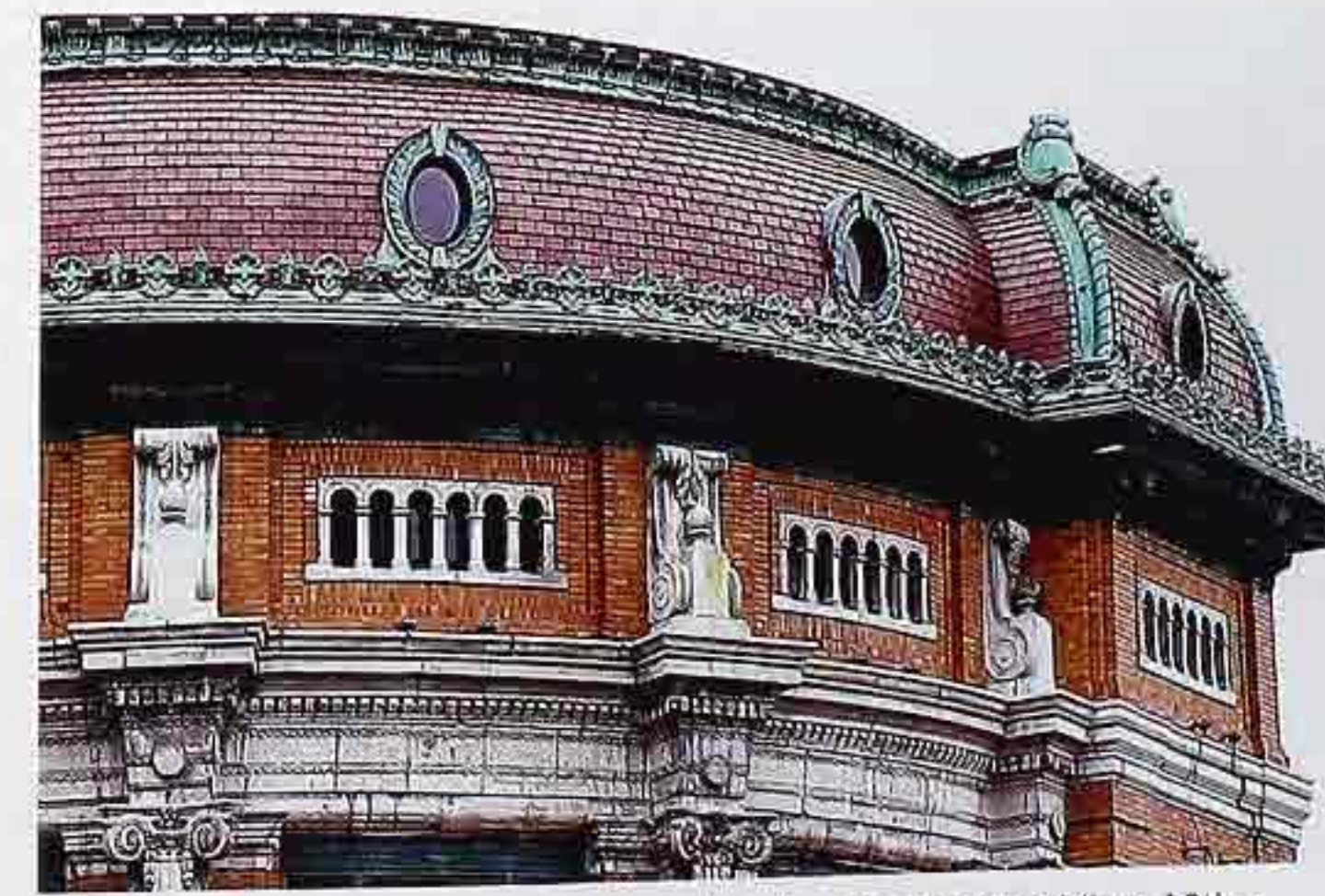
CR-53 Flat shingle tiles on convex curved roof with copper molding, 19th-c. mixed-use building
