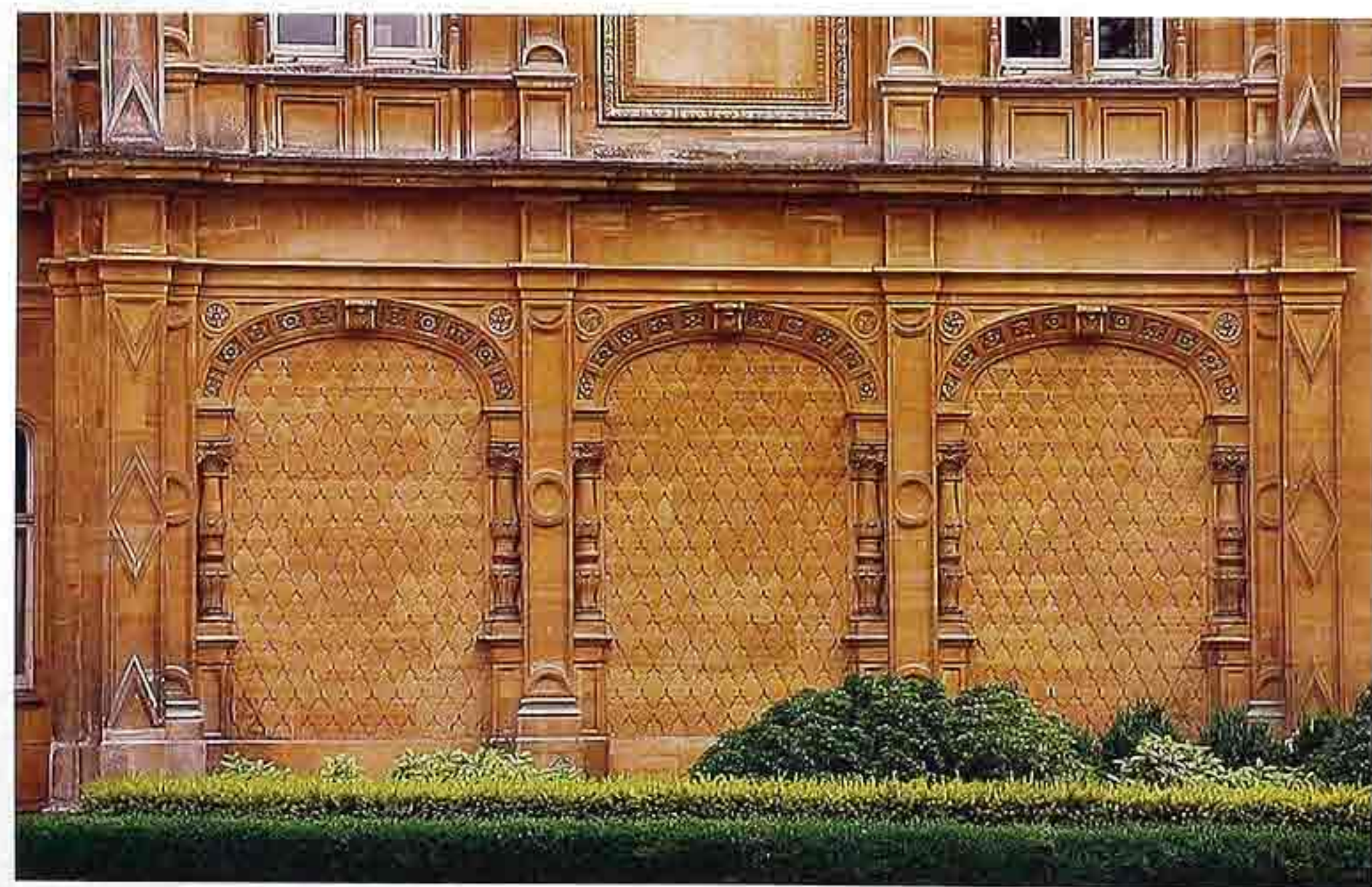
CP-172 Blind arcade: basket-handle (three-centered arch) stone arches with ornament, late-18th-c. courtyard
