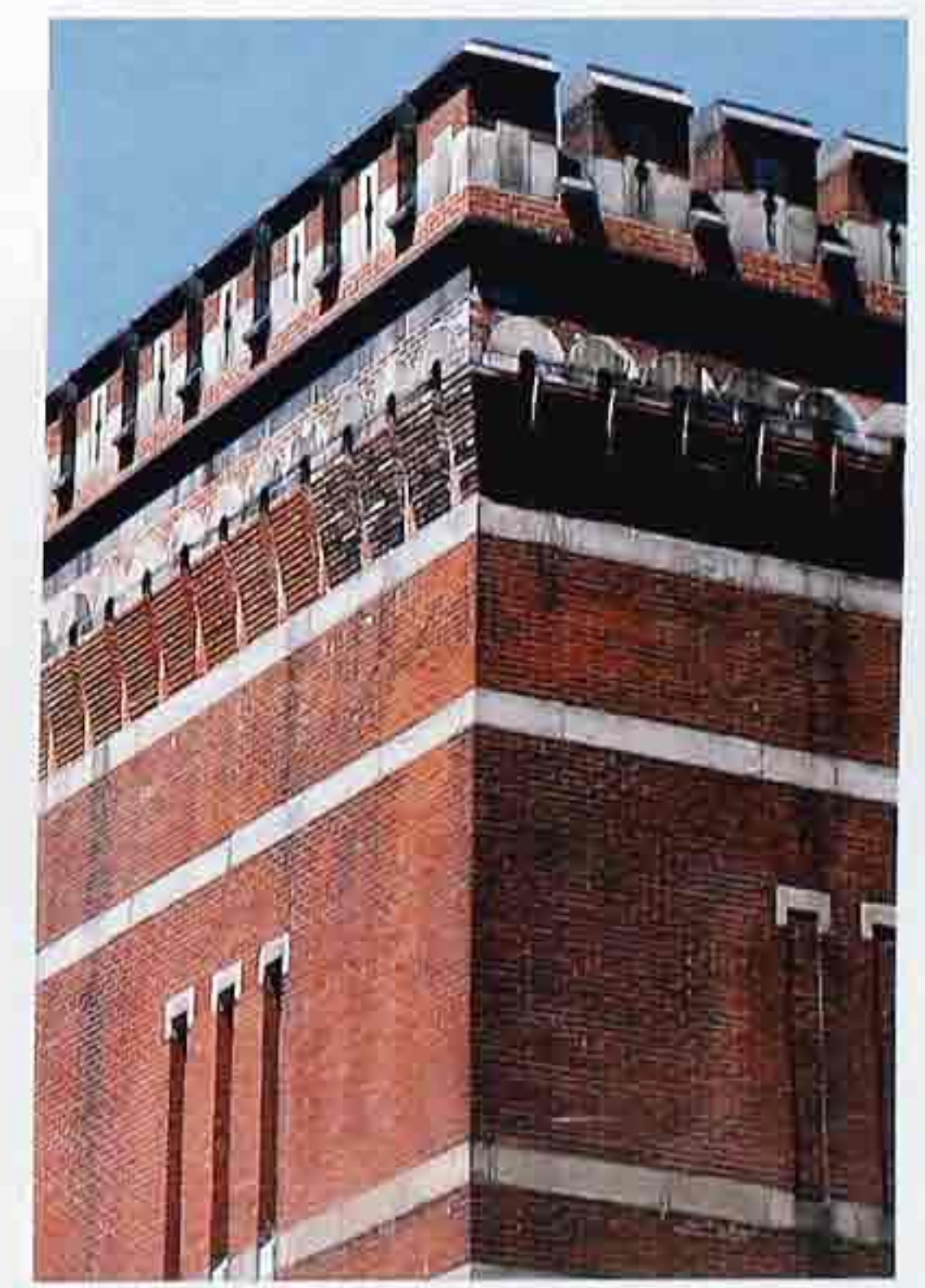
WA-196 Corner detail of Romanesque-style brick building with stone banding, parapet roof with crenellation
