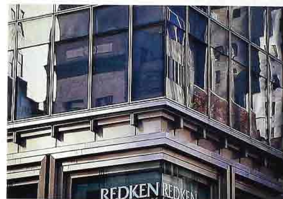
OM-75 Corner detail of metal fascia bands suggesting a classical entablature, the continuation of mullions suggesting a modillion band
