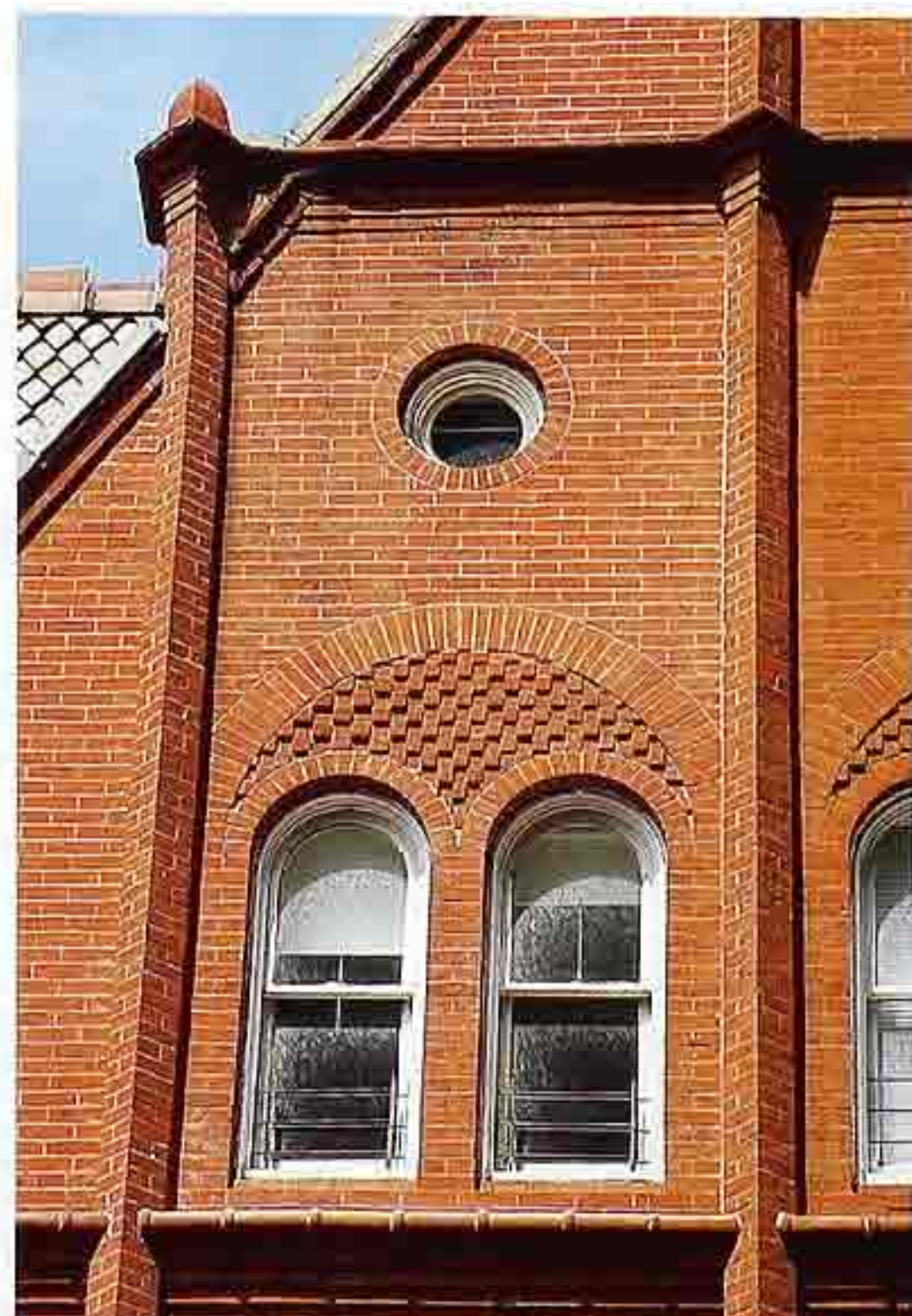
WI-58 One-over-one double-hung, arched top sashes with fixed lights; fixed bull's eye window above
