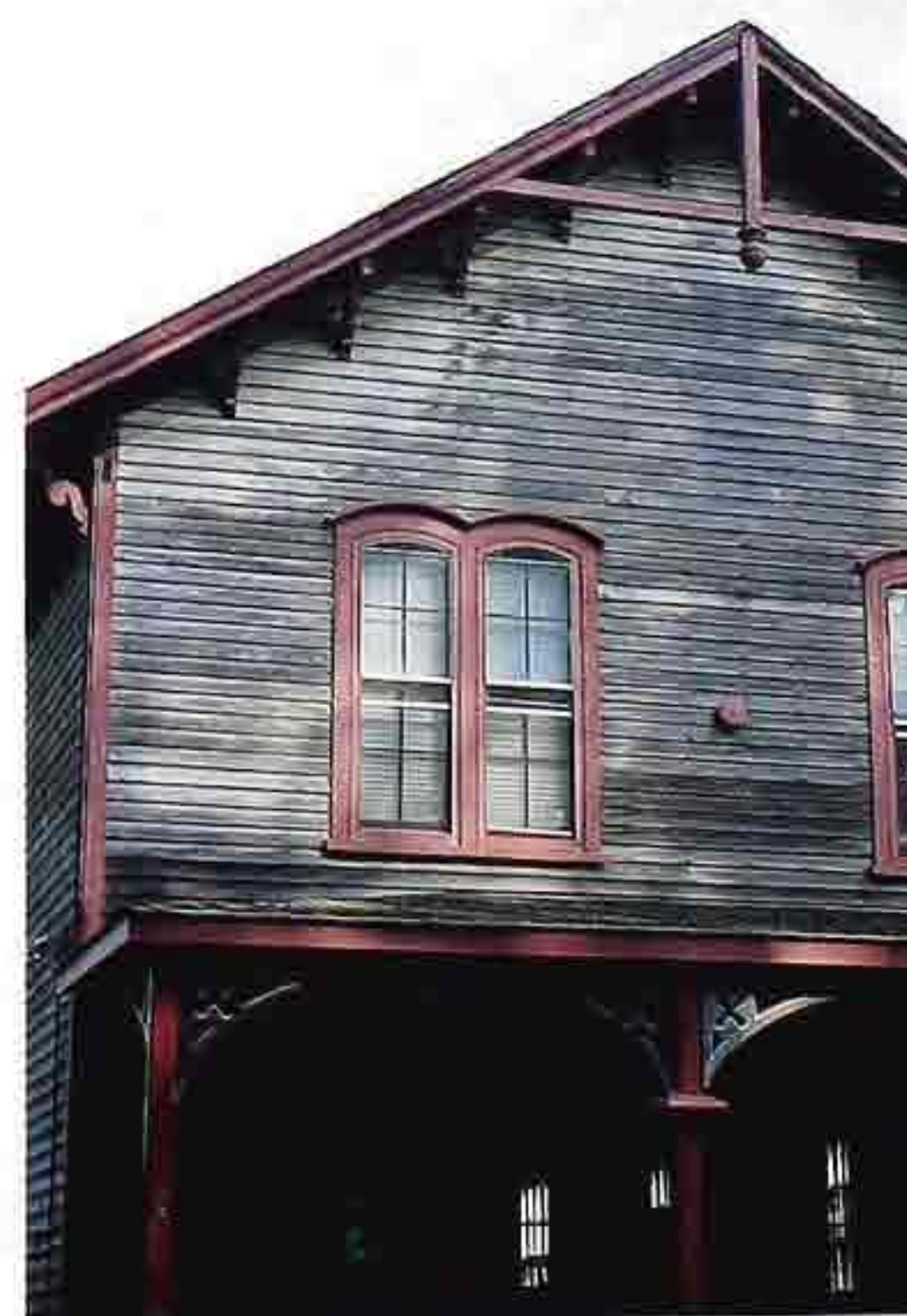
WI-53 Four-over-four double-hung windows with wood frames and modern storm windows, 19th-c. clapboard house
