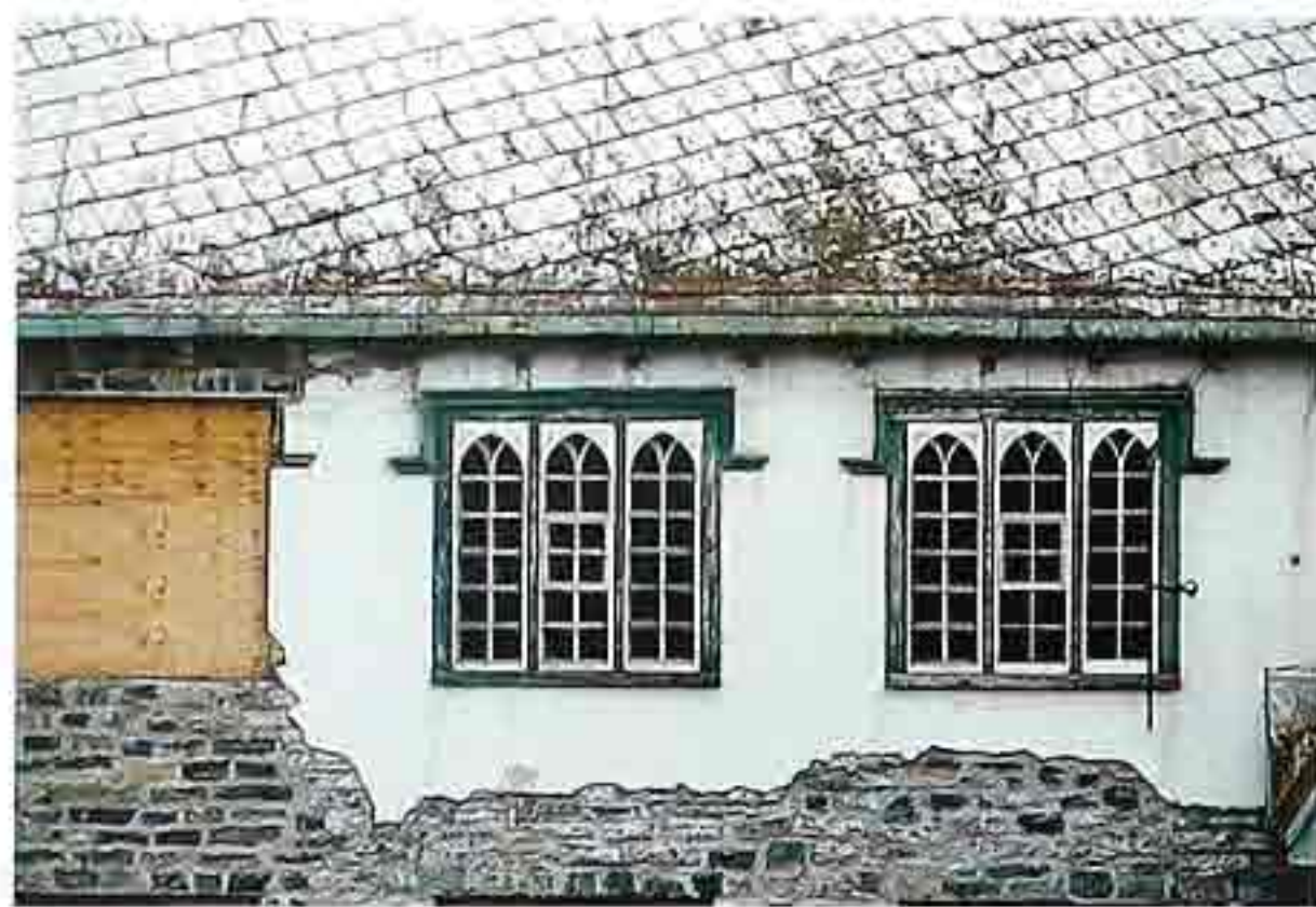
WA-254 Weathered painted plaster revealing structural stone and wood cladding
