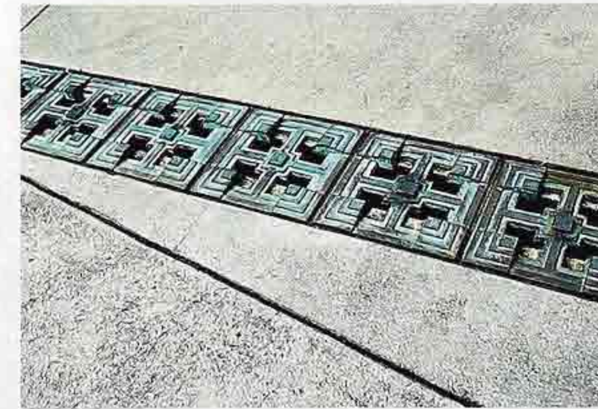
FP-111 Ornamented and patinated bronze drain covers in concrete driveway
